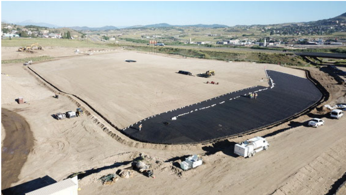
Construction of the engineered repository at the Montana Pole & Treating Plant site.
