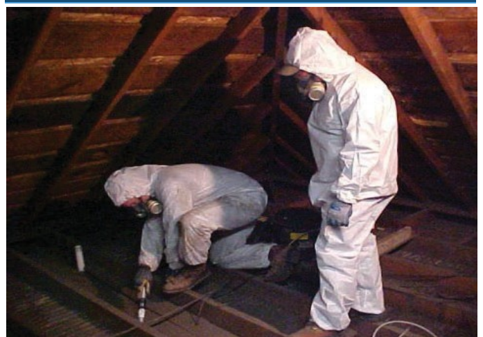
Picture of RMAP workers in Butte, MT in early 2000s, cleaning-up attic dust photo provided by Nikia Greene
