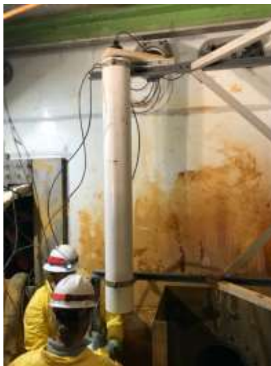
Photo 7: GK flow control structure weir box and associated water depth sensors.
