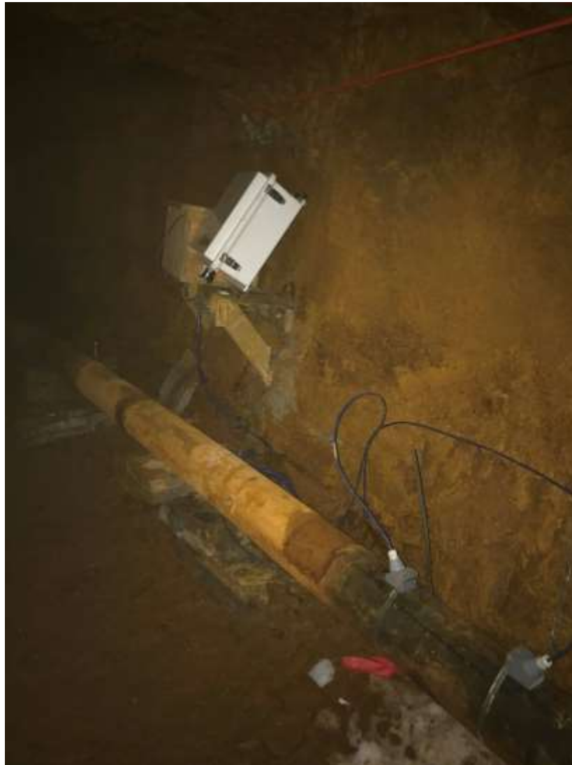
Flow sensor and data logger for the R&B discharge pipe, installed November 2017. Sensor located inside the mine tunnel but downstream of the bulkhead. Data logger powered by battery located in the adjacent storage box.
