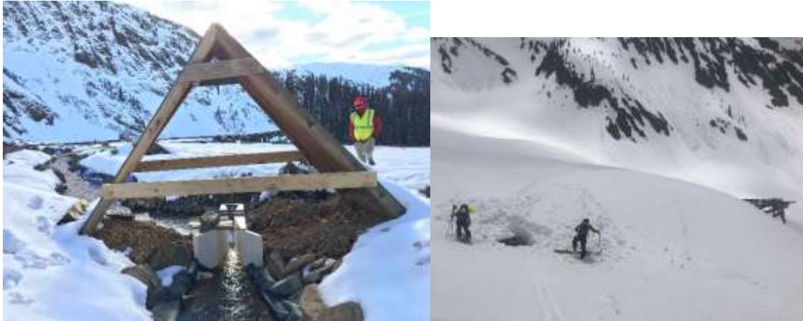
Left; Blackhawk flume and snow shed, installed fall 2018. Right; Location of functioning flume protected by the snow shed, May 15, 2019.
