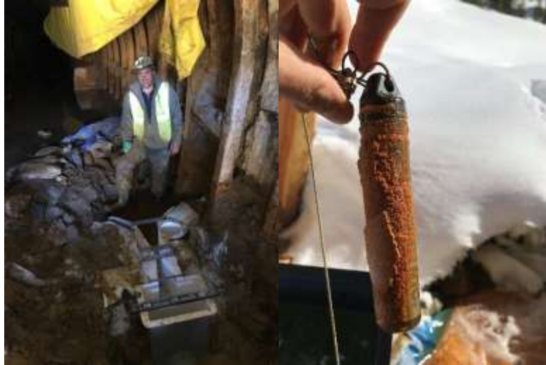
Installation of fiberglass flume in the American Tunnel drainage ditch, October 2018. The downstream end of the flume is a fill basin connected to a pipeline that conveys water out of the mine portal. Second photo is an example of sludge build up on the pressure transducer at American Tunnel in less than 30 days.
