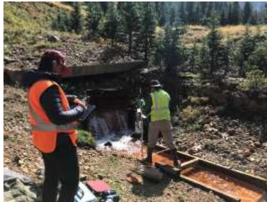
Natalie Occidental custom weir box installed summer 2017. The 30" wide weir box designed to measure large variations (>1,000 GPM) in flow and enable use of a flow meter to accurately measure discharge.
