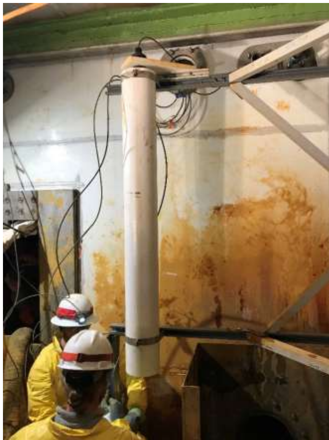
Installation of the water level monitoring devices adjacent to the weir box behind the Gold King flow control structure, October 4, 2018.
