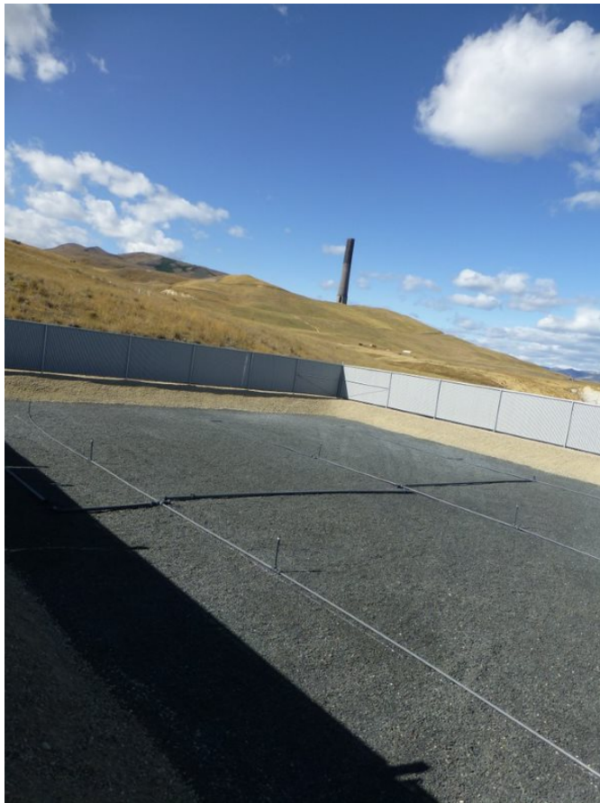
OU11: Flue Dust leachate collection and evaporation system
