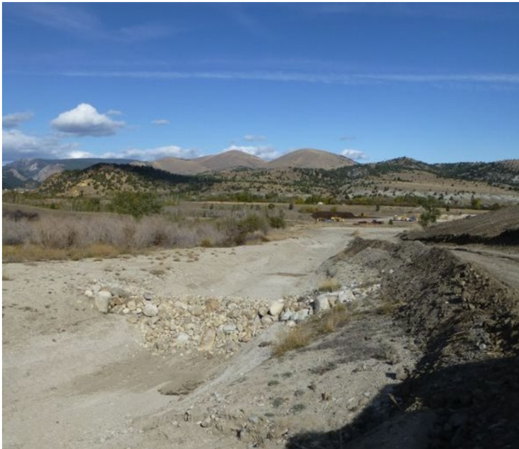
OU4: North Opportunity area showing check dam for stormwater control
