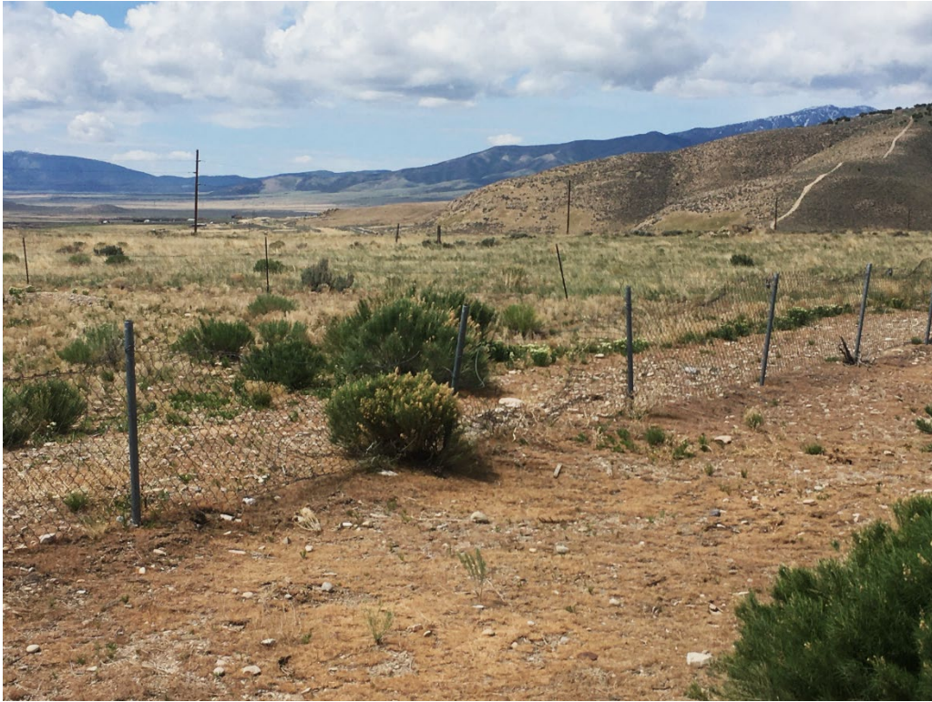
Photo 5: OU2 Fence Damage at Rawhide Ranchettes Repository (Location 1)
