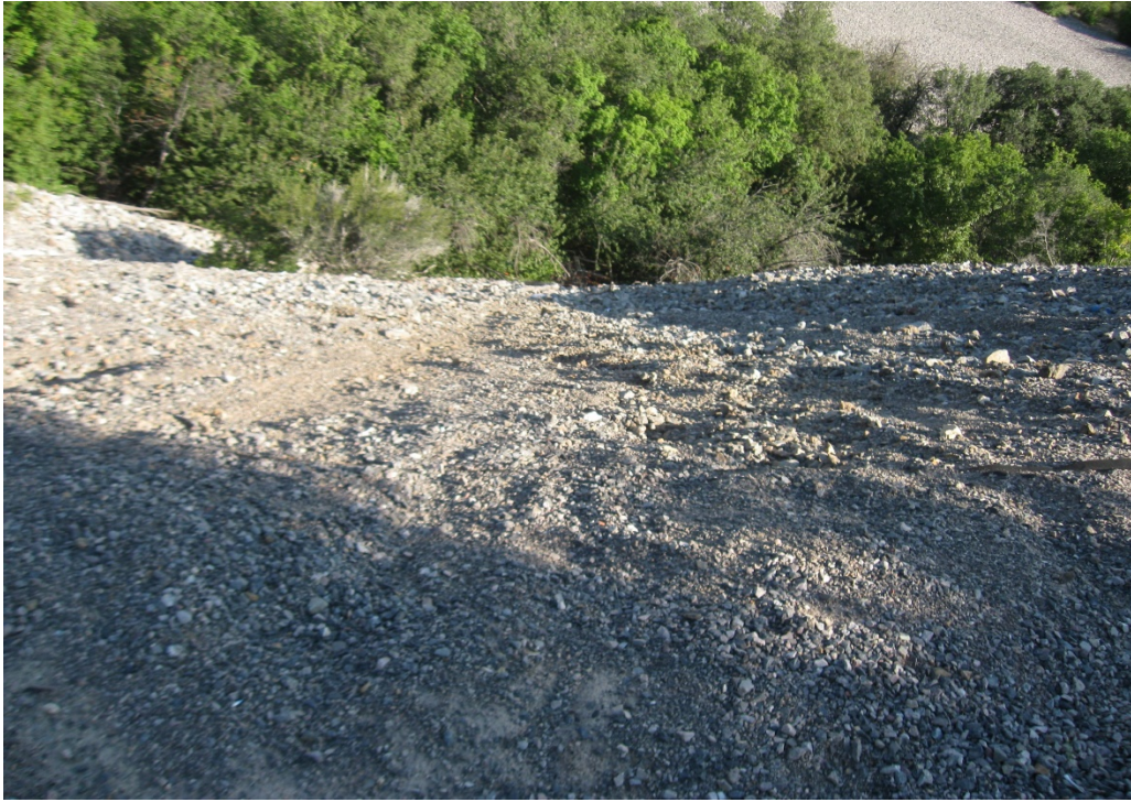
Roadbase eroded of lower slope of Upper Godiva
