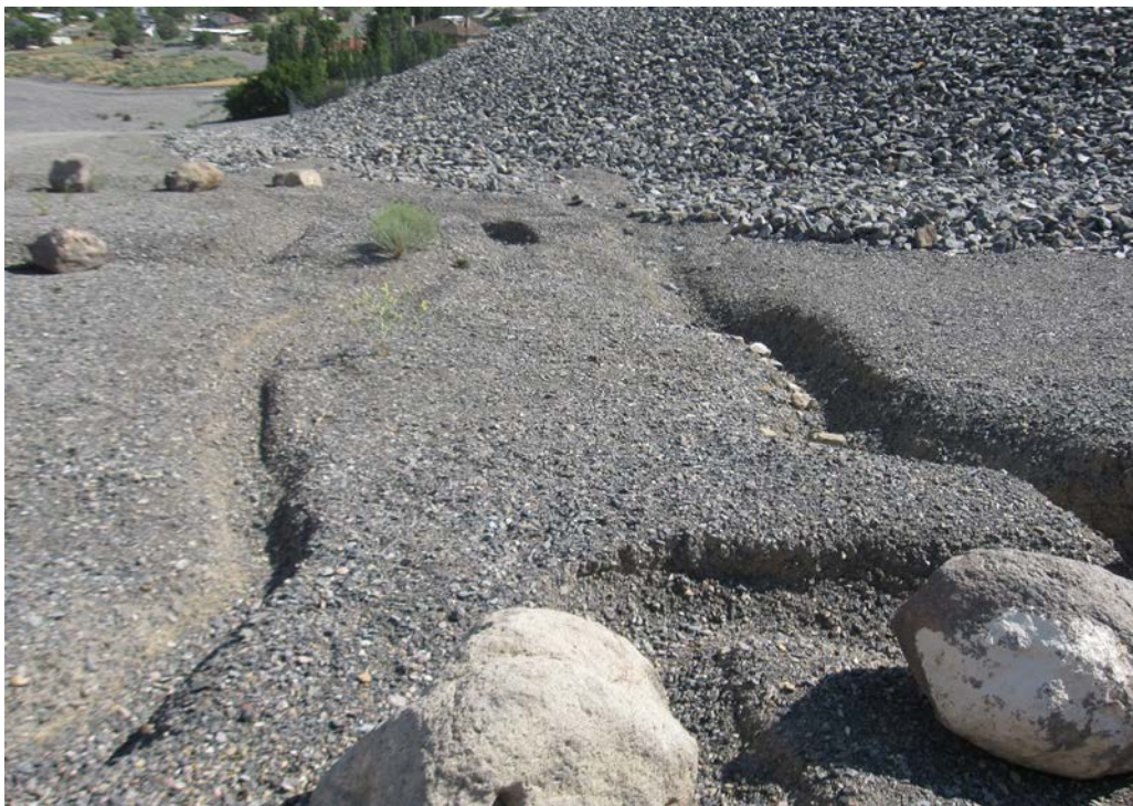
Erosion rills on west side of Eagle Blue Bell Water Bars
