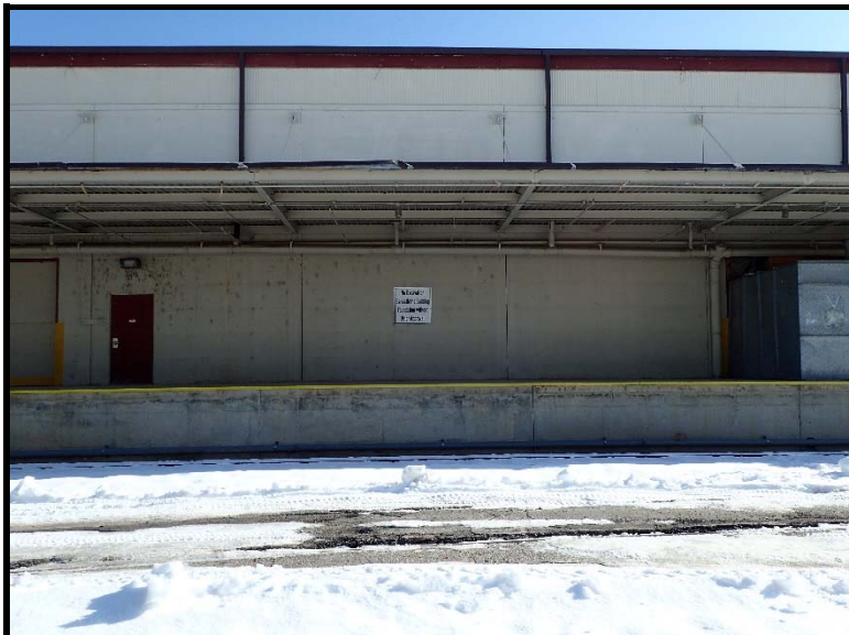
Warning Sign on Building 16C
