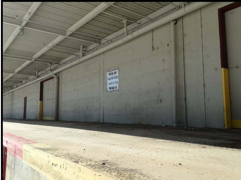
Warning Sign on Building 15C
