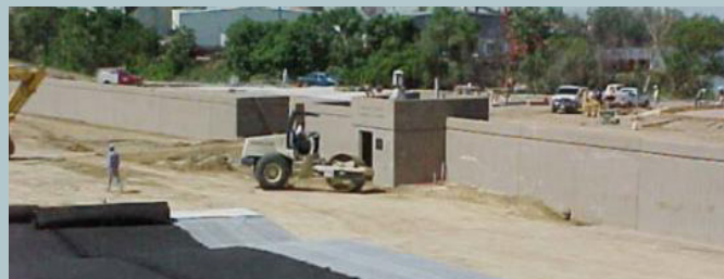
Placement of a liner system to contain lead-contaminated soils in a "burrito" prior to adding several feet of clean soil as a cap.
