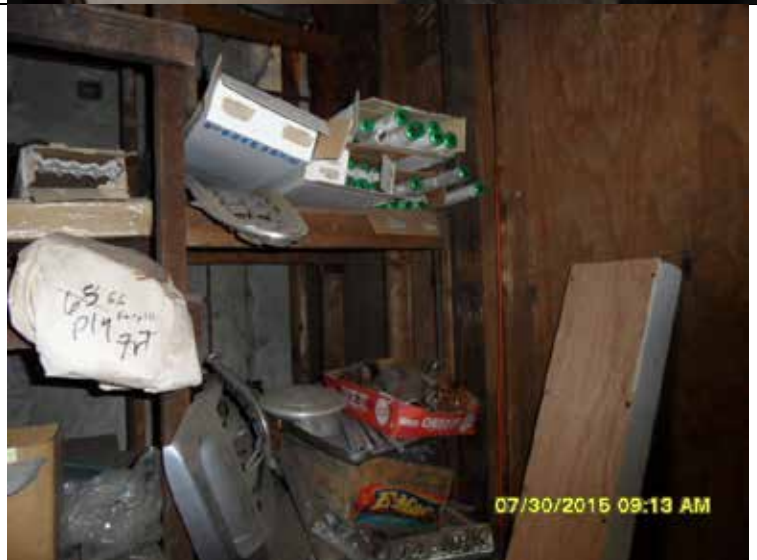
PHOTOGRAPH# 12 DATE TAKEN: 7/30/15 BY: Michael Davis DESCRIPTION: Maintenance Area- Used lamp storage area. Boxes not closed (Violation-S3 in checklist).
