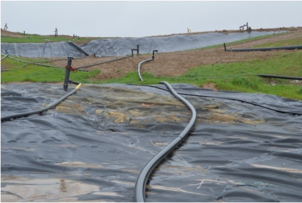
Photo 3. Heat Deterioration of FML, Measured Temp. 128°F, April 2013 (Source: DNR Staff, 2013).
