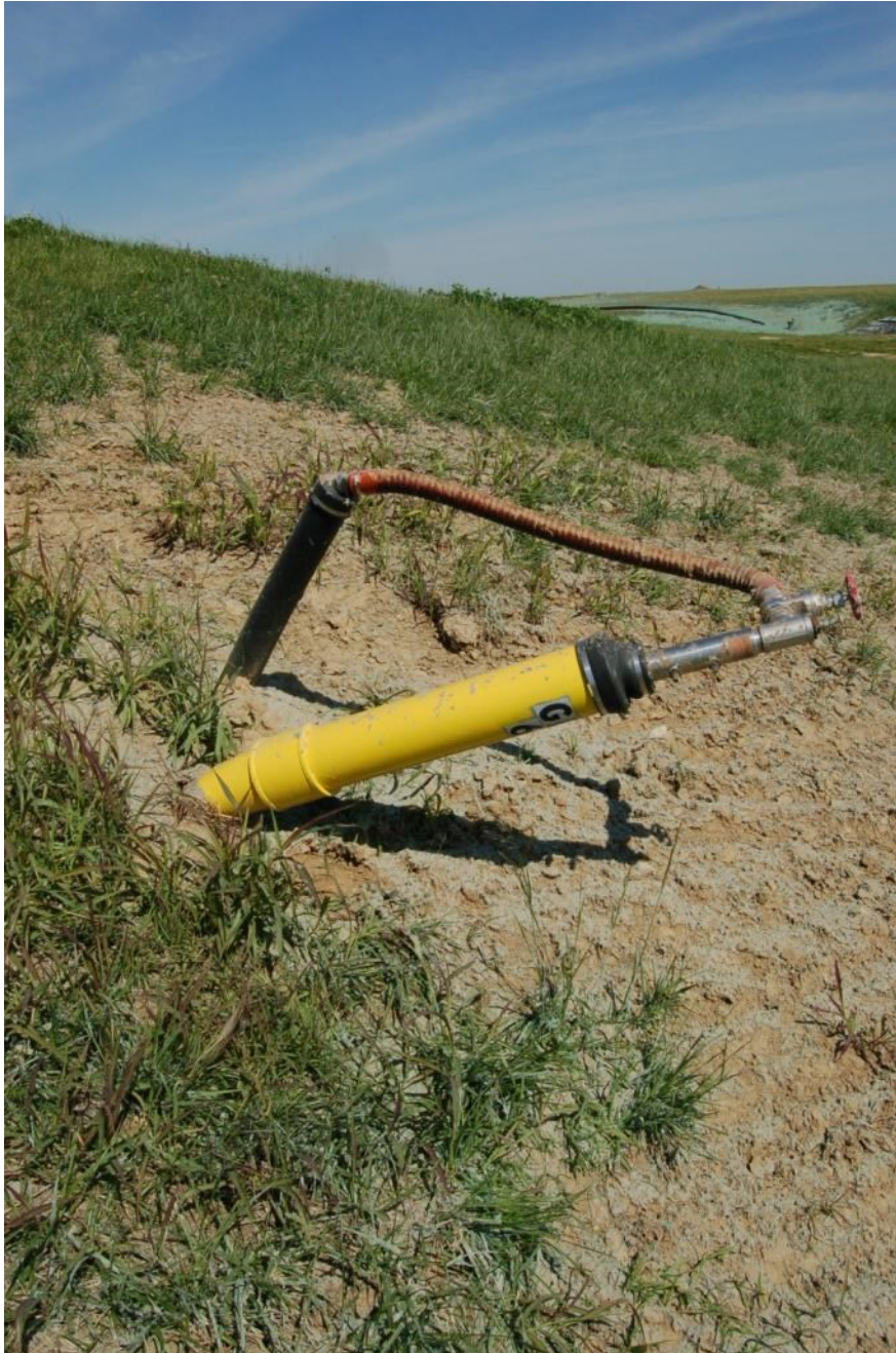
Photo 2. Damage Gas Collection Well (Source: DNR Staff, 2012).
