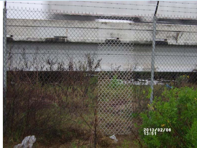
Photo 26: Repaired fence fabric, south alignment, west bank of the San Jacinto River I-10 crossing (view north)
