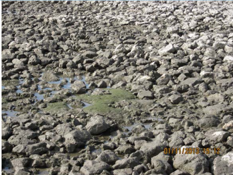
Photo 17: Background location from Photo 16 of thin armor cap area and exposed geotextile identified during visual inspection (view southwest)
