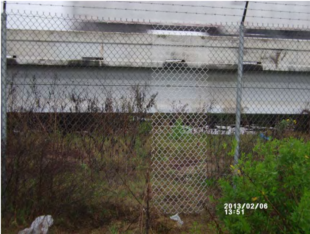
Photograph 1 – Repaired fence fabric, south alignment, west bank of the San Jacinto River I-10 crossing
