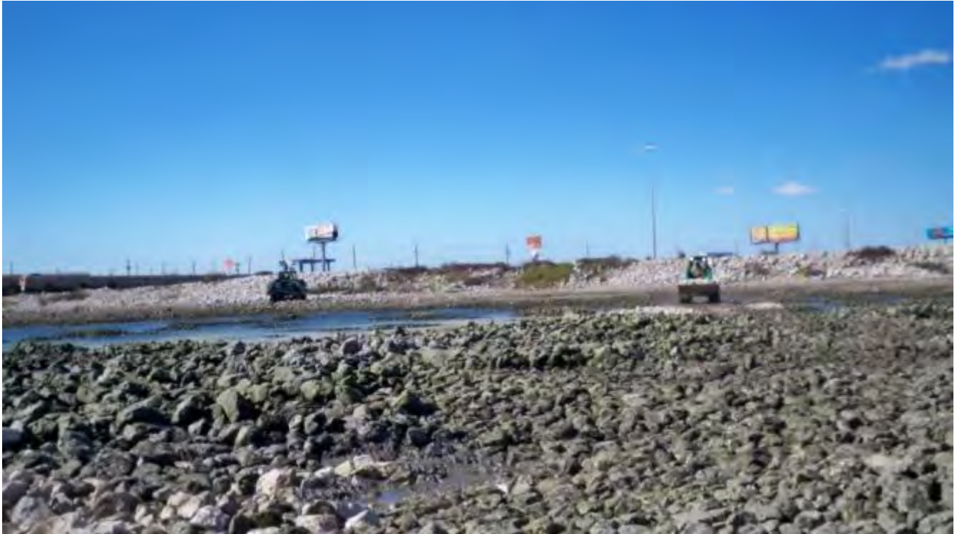
Photograph 2 – Skid Steers transporting rock along central berm, then across MA 2 to MA 3.
