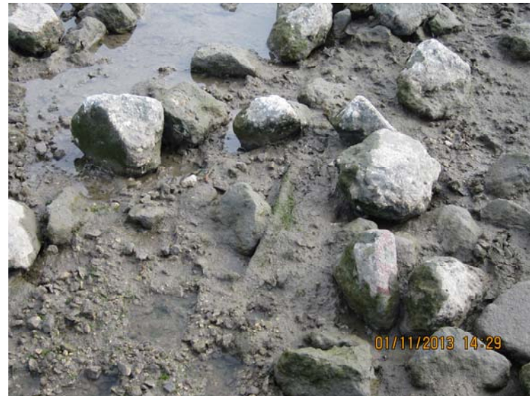
Photo 12: Thin armor cap area identified during visual inspection (view north)
