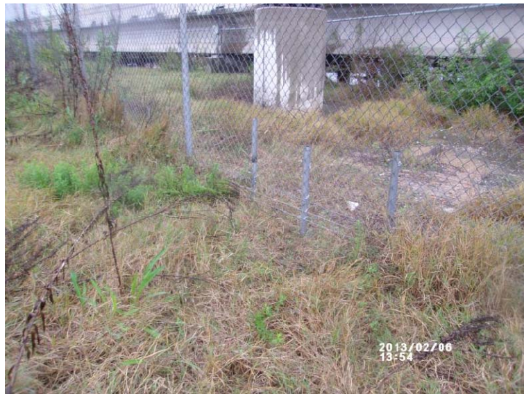
Photo 27: Added lower supports on adjacent panels to secure fence fabric and barb wire (view northwest)
