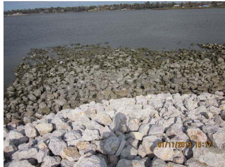
Photo 20: Northern end of the central berm; color variation in armor rocks indicates the submerged portions of the cap under normal tidal conditions (view north)
