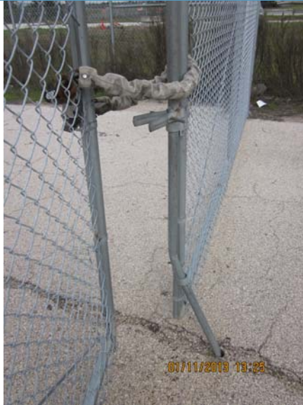
Photo 05: Bent center post of east access gate (view east)
