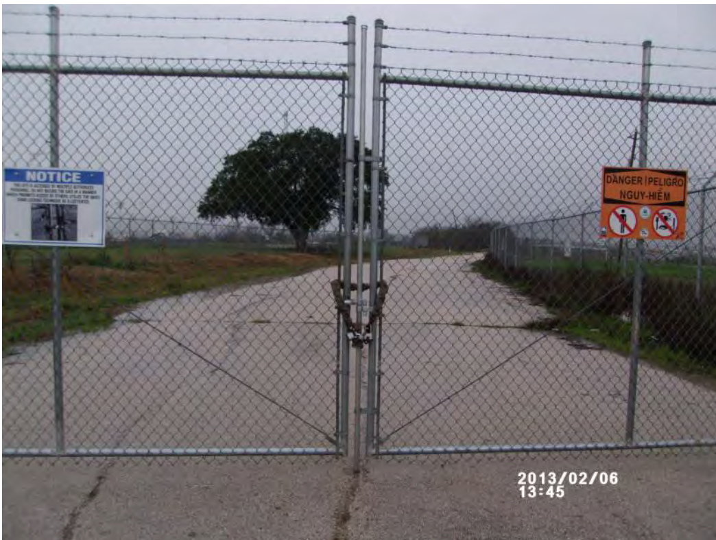
Photograph 5 – New gate center post installation, east bank. All fence maintenance actions complete.
