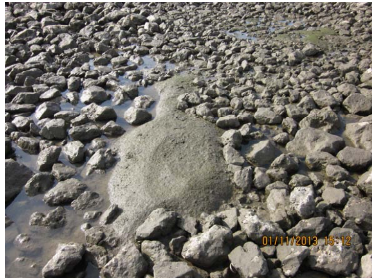
Photo 16: Areas (foreground and background) of thin armor cap area and exposed geotextile identified during visual inspection (view northwest)
