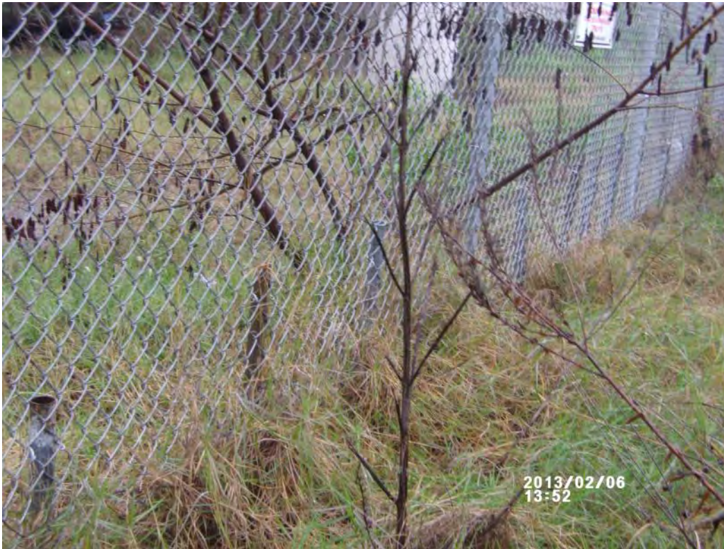
Photograph 4 – Added lower supports on adjacent panels to secure fence fabric and barb wire.
