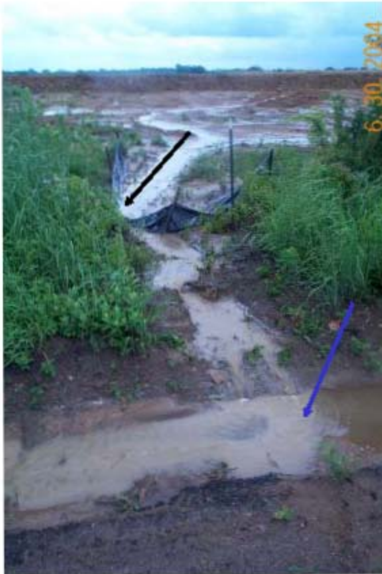
Photo 49: View of drainage ditch and runoff discharge point from borrow source property. The silt curtain erected across the discharge point has collapsed (black arrow). Water in the drainage ditch becomes discolored where runoff enters from the borrow source property (blue arrow).
