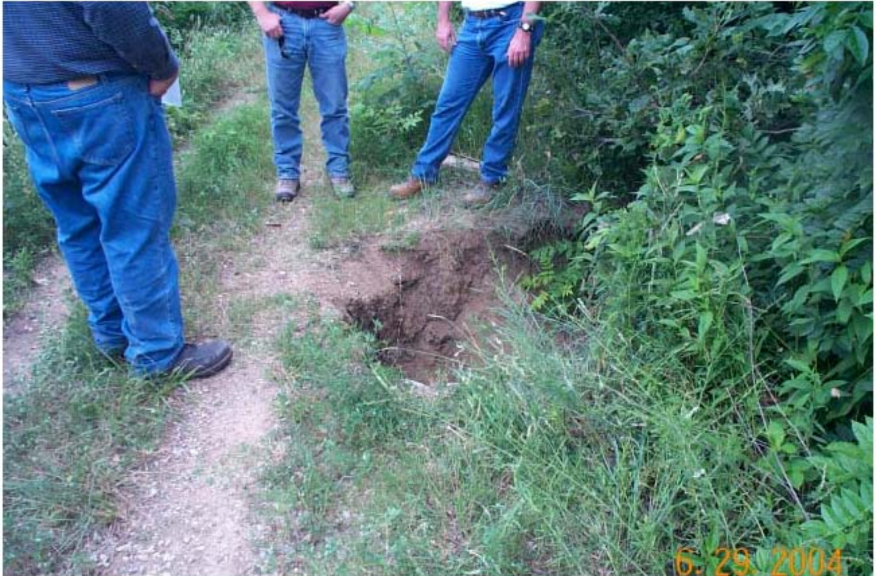
Photo 5: View of collapse feature on dike at the Admiralty Mine site. This dike is located east of the Douthat Bridge on E40 Road near the confluence of Tar Creek and Lytle Creek.
