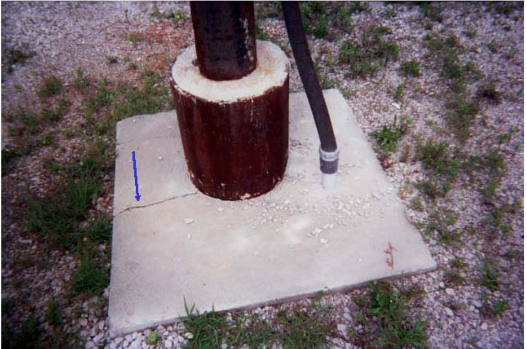
Photo 52: View of well pad for Quapaw #5 MW. Well pad is cracked (blue arrow).
