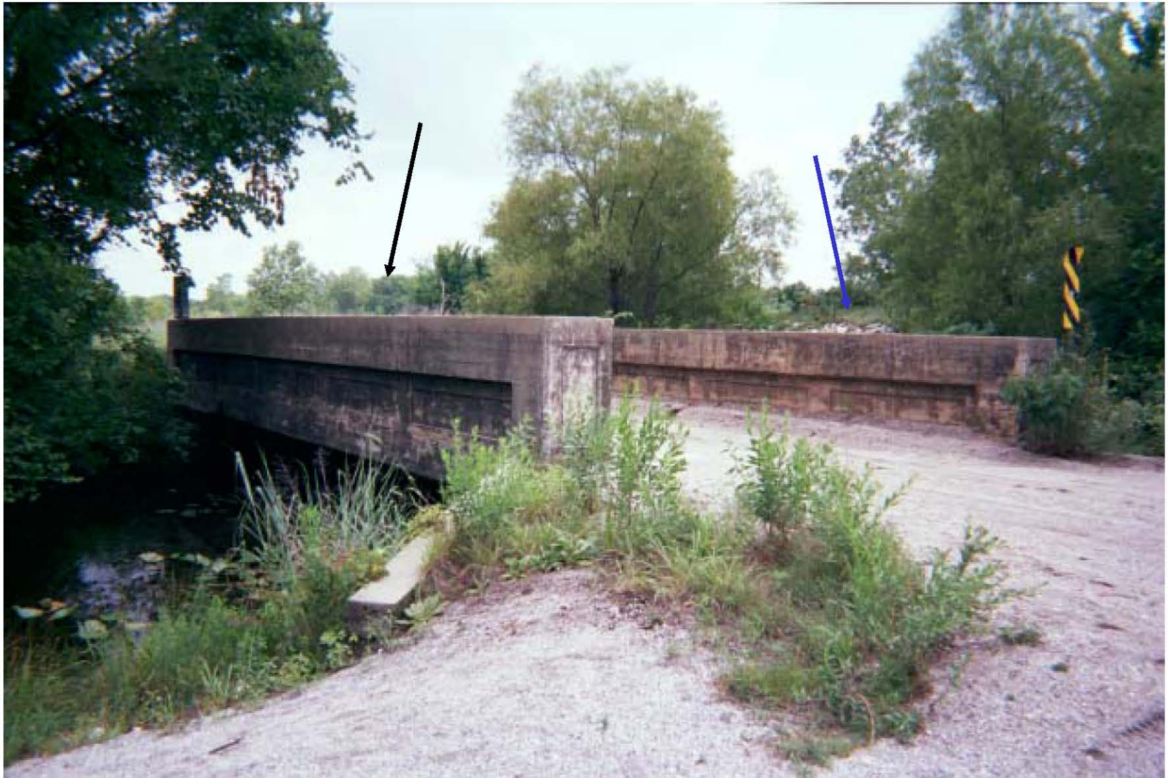
Photo 67: View of the bridge over the old Tar Creek channel at the Big John Mine site, located in Kansas (facing northwest). The backside of the diversion dike is barely visible above the bridge (at the blue arrow). Tar Creek has been diverted away from this location. The new channel is located in the trees in the background (at black arrow).
