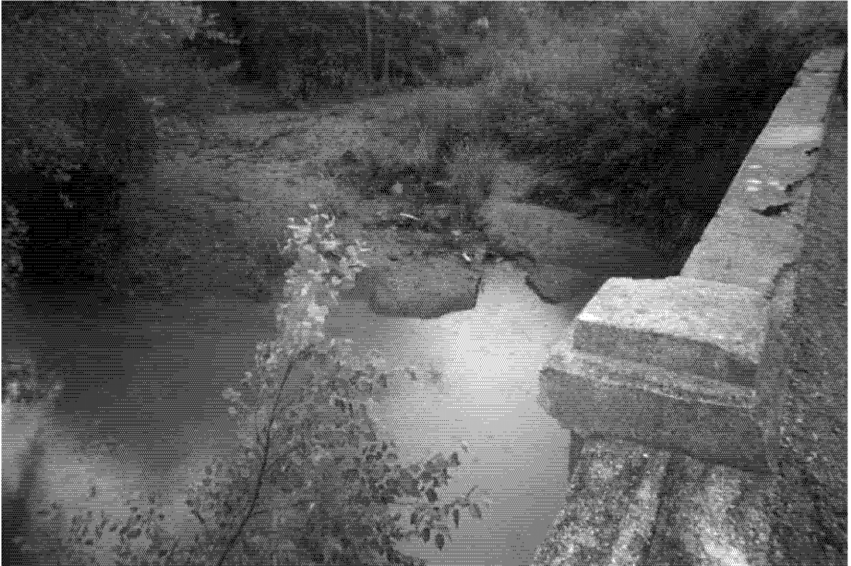
Photo 76: View of the downstream side of Tar Creek at the Douthat Bridge. The color of the water in the stream is red and orange from iron oxide precipitating out of solution in the water. Note the red staining on the shore, where the iron oxide has been deposited by the stream.
