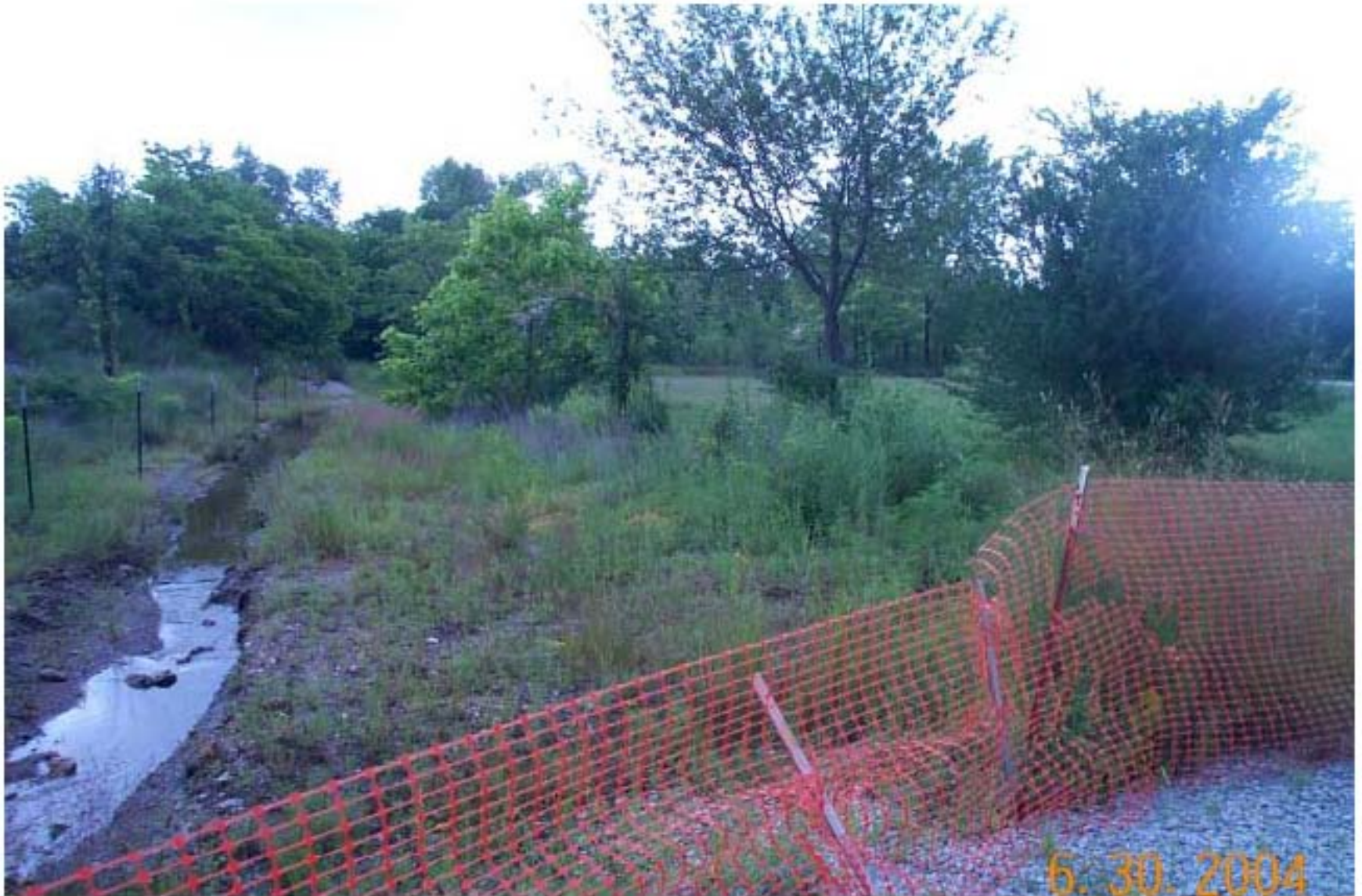
Photo 39: View of property under construction in Cardin, Oklahoma. There were still a few remaining items to complete on this property at the time of the site inspection.
