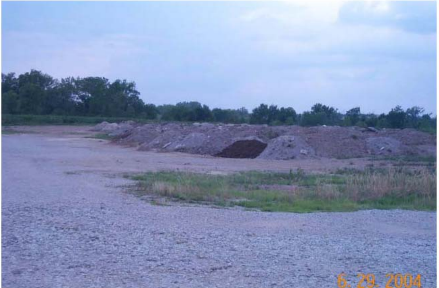
Photo 24: View of recently deposited soil at repository on E40 Road. Lead contaminated soil from residential yards is used at the repository to fill in an old mill pond.
