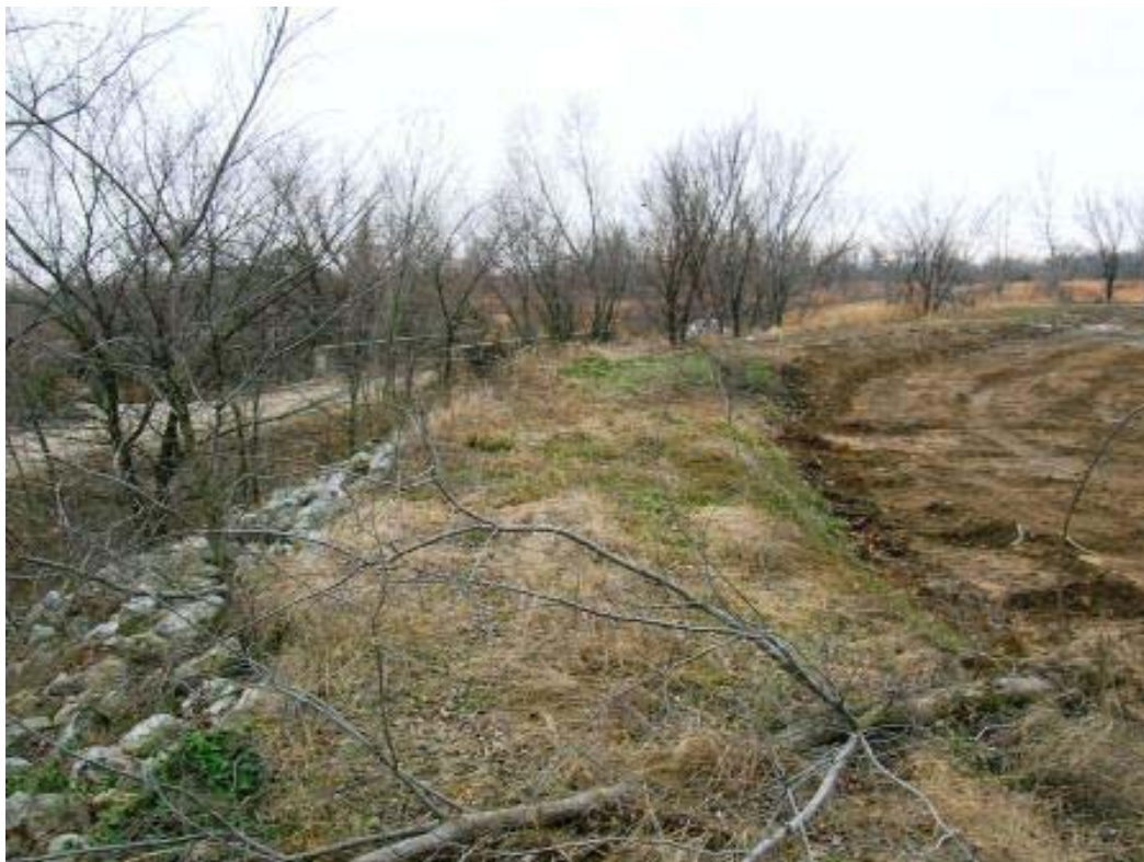
Photo 6: Remediation at the Muncie site in Kansas, being performed for the Treece Subsite of the Cherokee County Superfund Site (EPA Region 7). Rip-rap on the diversion dike is present to left. Bridge in center of picture goes over the old Tar Creek Channel. View is facing west.
