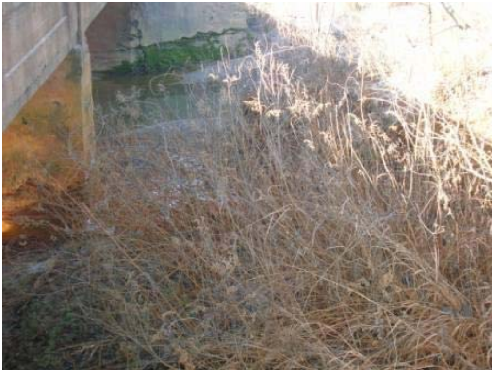
Photo 78: View of Tar Creek under Douthat Bridge. Mine water discharges into Tar Creek within vegetation in foreground.
