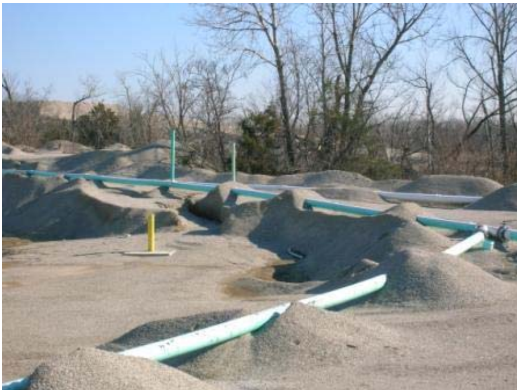
Photo 62: Piping used to feed wash-water and washed fine tailings from chat washer to injection well.
