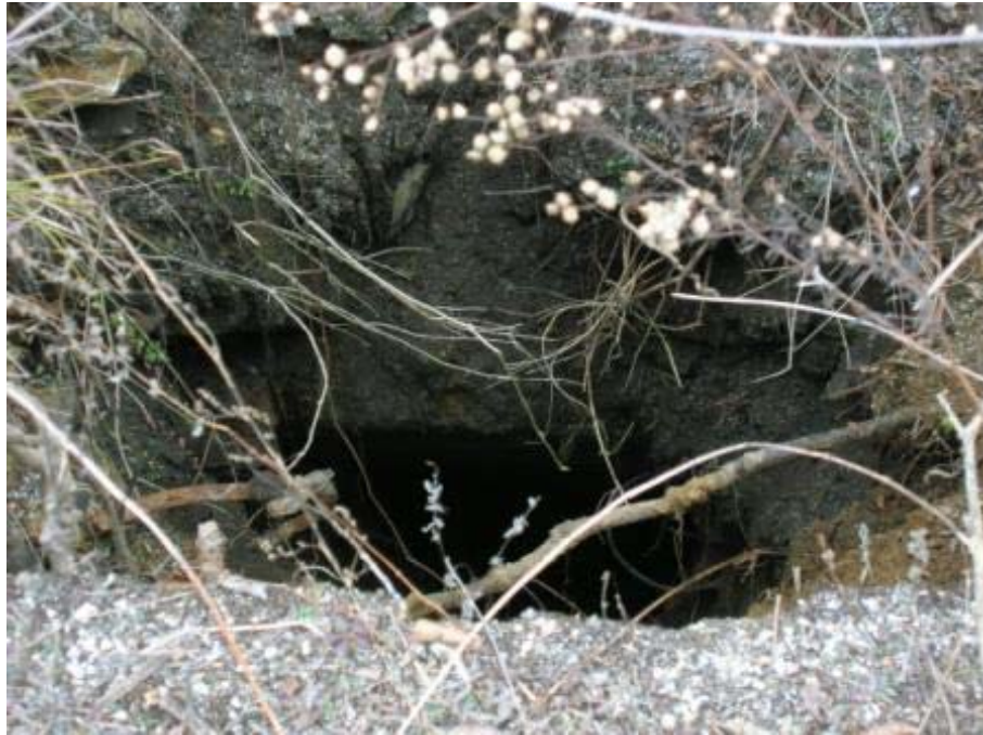
Photo 27: Close-up view of mine shaft collapse on the east side of Picher near Picher Well No. 6-MW.
