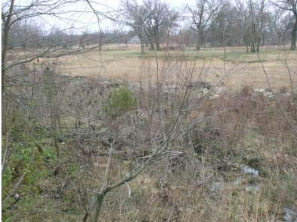
Photo 19: View of channel improvement on Tar Creek tributary west of Tar Creek and northeast of Big John site. Rip-rap is present along cut-bank in center of photograph. View is to the south.
