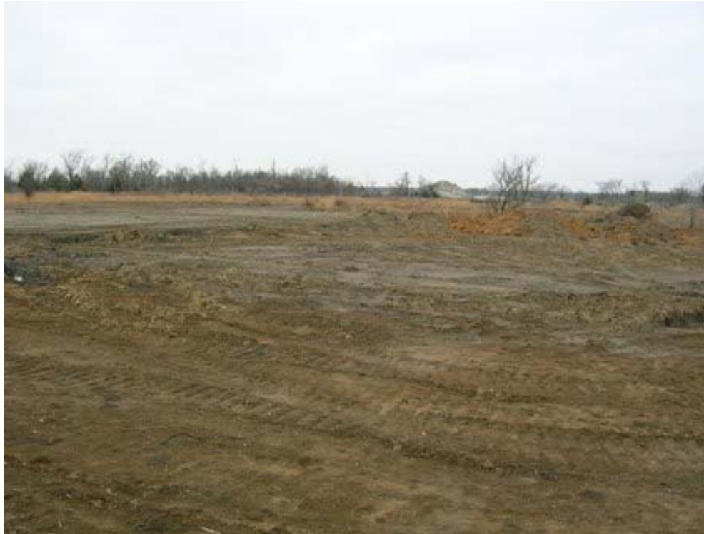
Photo 5: Remediation at the Muncie site in Kansas, being performed for the Treece Subsite of the Cherokee County Superfund Site (EPA Region 7).
