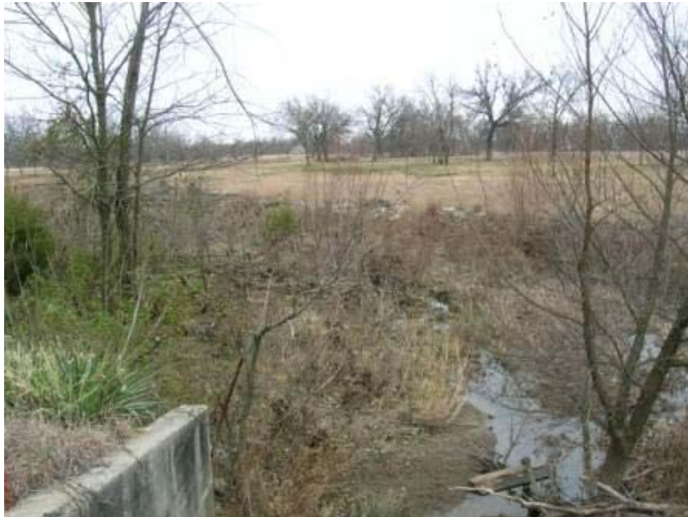
Photo 18: View of channel improvement on Tar Creek tributary west of Tar Creek and northeast of Big John site. Rip-rap is present along cut-bank in center of photograph. View is to the south.
