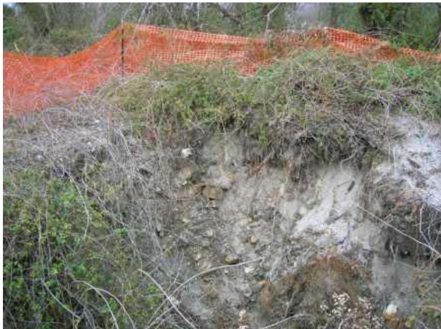
Photo 28: View of mine shaft collapse with orange barricading placed around it.
