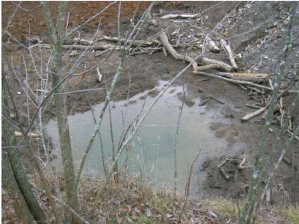
Photo 8: Close-up view of the bottom of the Muncie subsidence.
