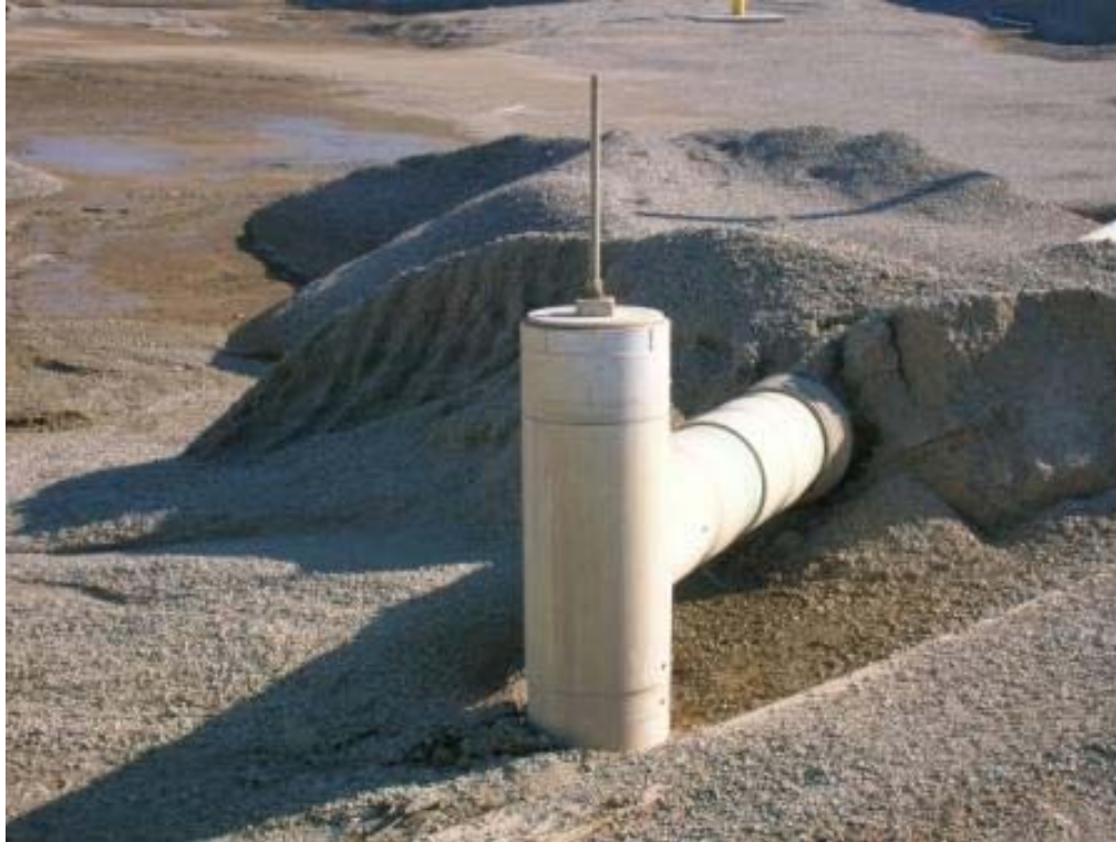
Photo 61: Close-up view of injection well.
