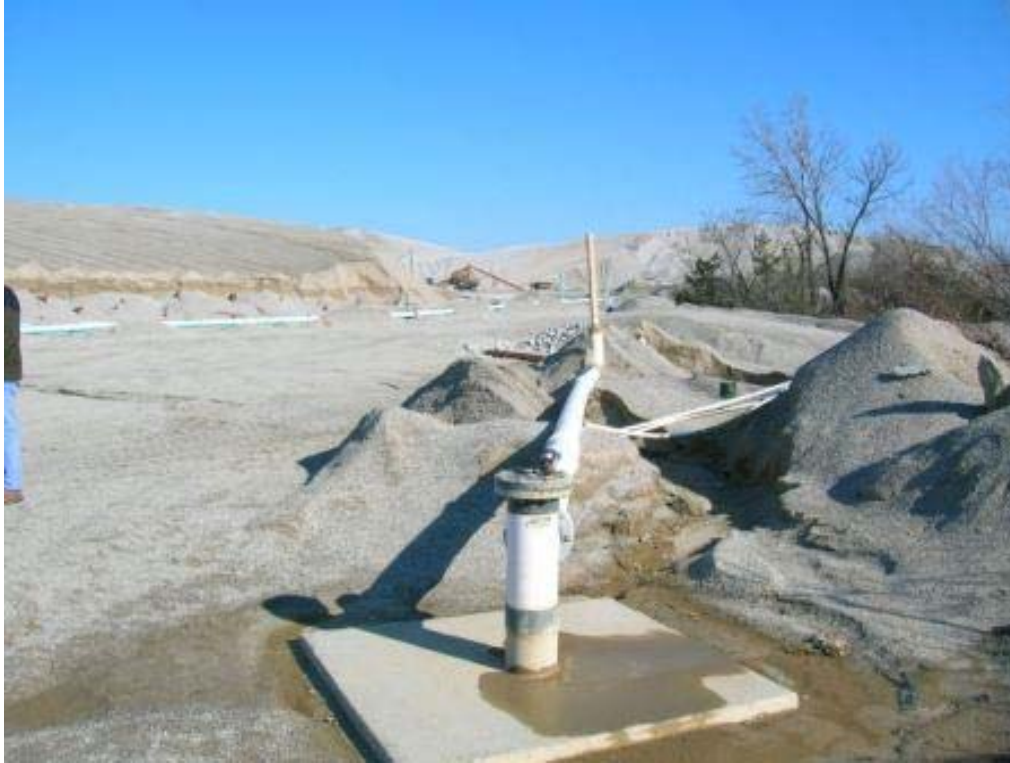
Photo 65: Close-up of injection well and pipeline. Chat washing unit is visible in center background.
