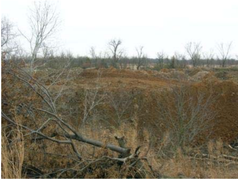
Photo 11: View of dirt being used to fill in subsidence at the Muncie site.
