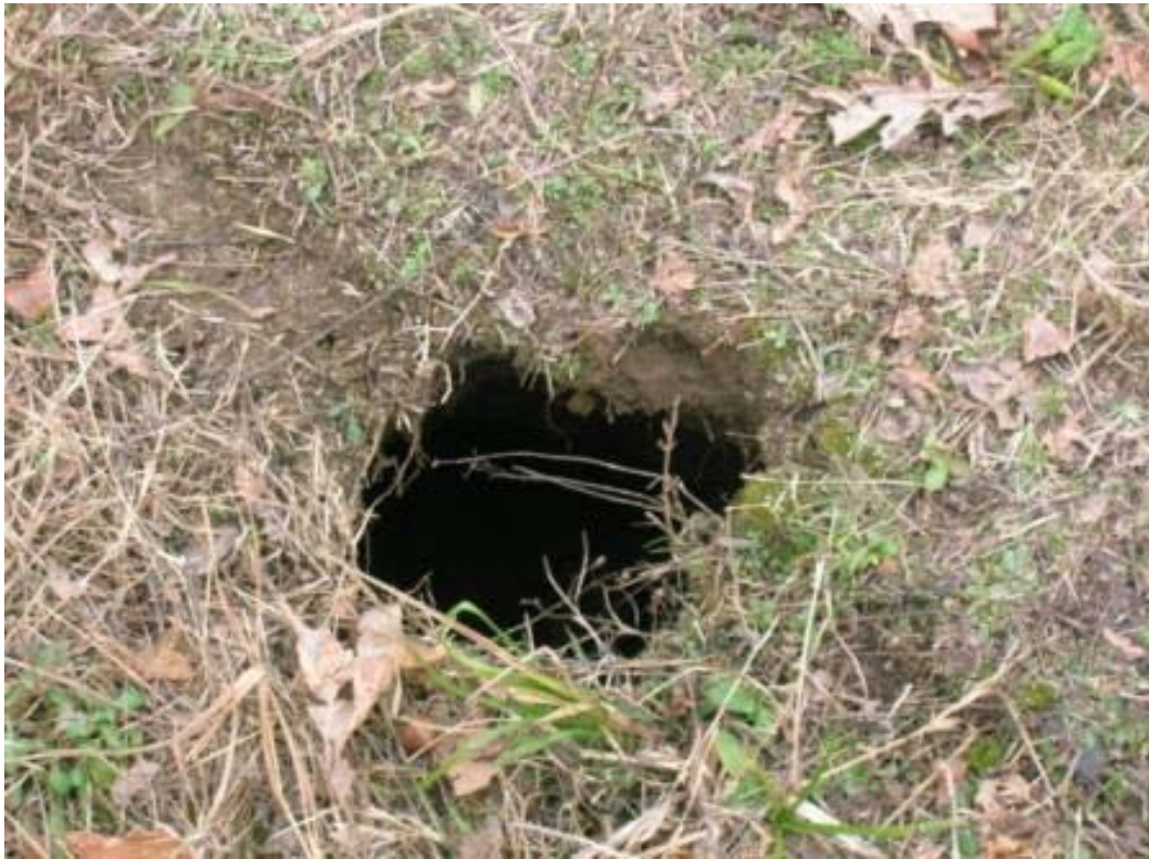
Photo 42: View of small collapse on top of Admiralty diversion dike. Hole is 10-12 inches across.
