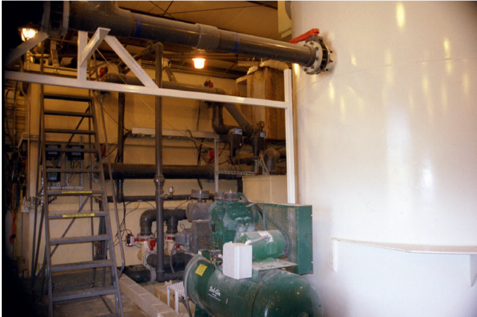
Inside reverse osmosis plant.
