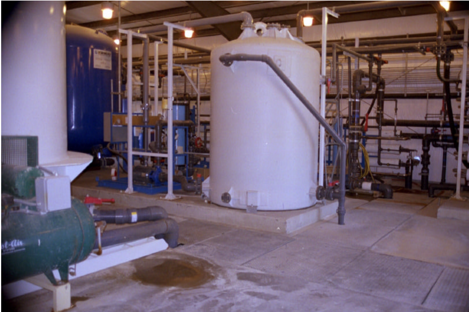
Inside reverse osmosis plant.
