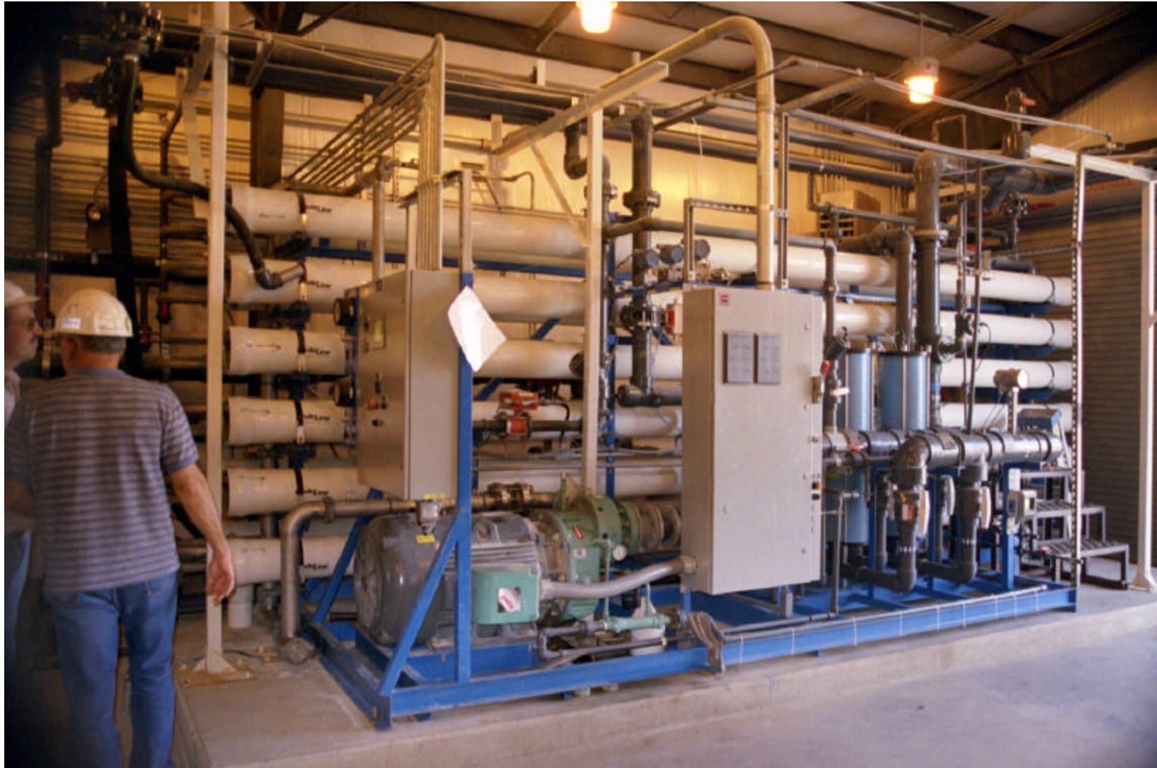
Inside reverse osmosis plant.
