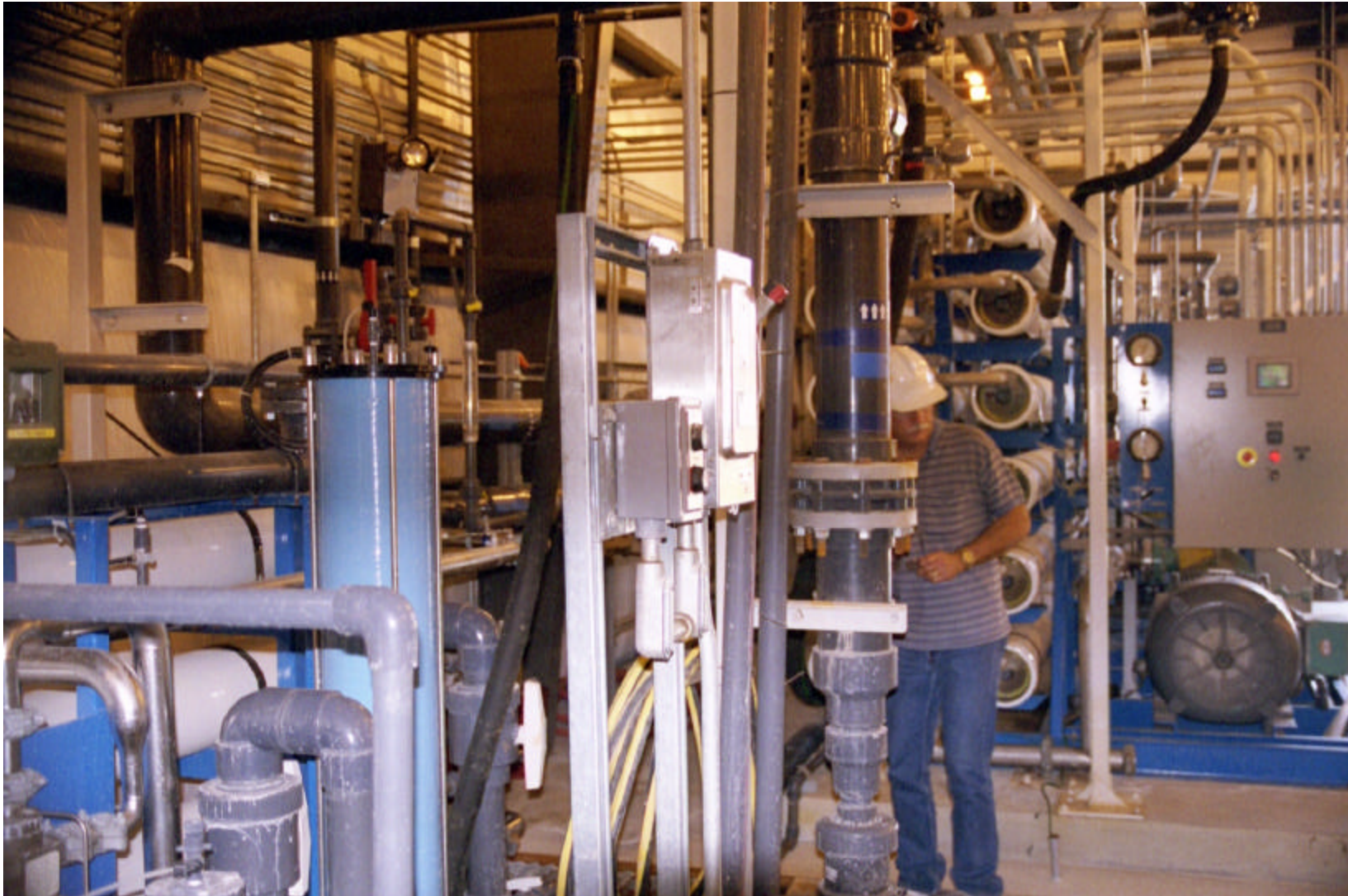
Inside reverse osmosis plant.
