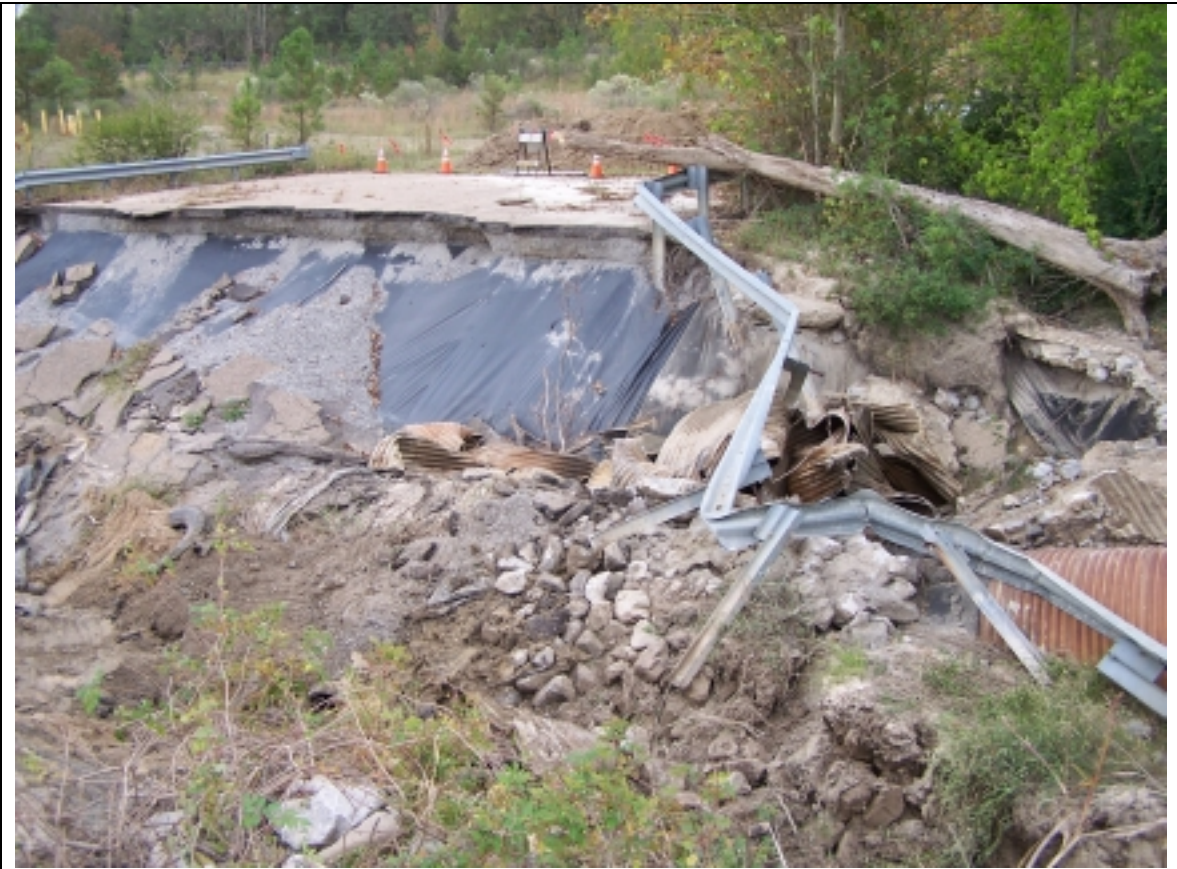
Photograph 27 – Bridge Failure, Scenic OU, Southwest 11/11/08
