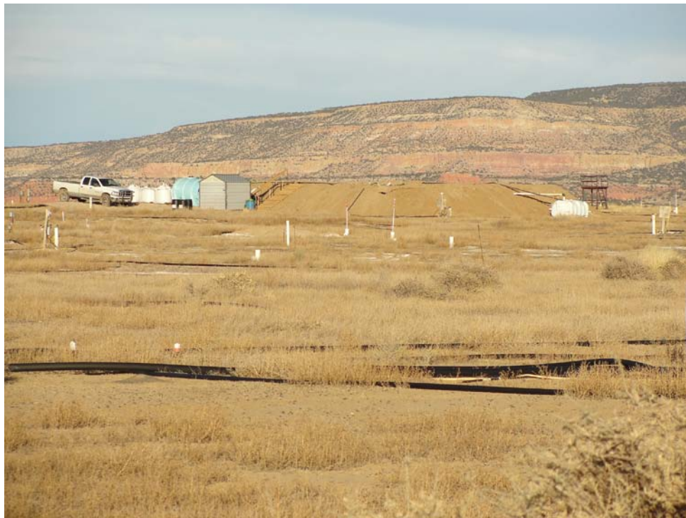
Photo 7: Zeolite pilot-test area on the south side of the top of the large tailing pile. Note extraction wells (white) and piping in foreground used to convey collected groundwater to the RO treatment plant or to one of the evaporation ponds for disposal. View looking northeast.
