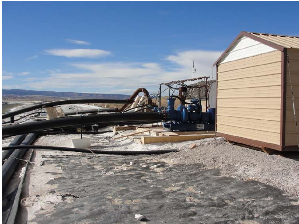
Photo 10: Pump, pump house, and piping at Evaporation Pond 1. Equipment is used to convey extracted groundwater from the large tailings pile (to the right out of the photo) to the evaporation pond. The black surface is an asphalt-emulsion liner that forms the base for the pond. View looking west.
