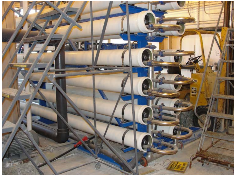
Photo 16: A portion of the membrane filtration system in the RO treatment plant.
