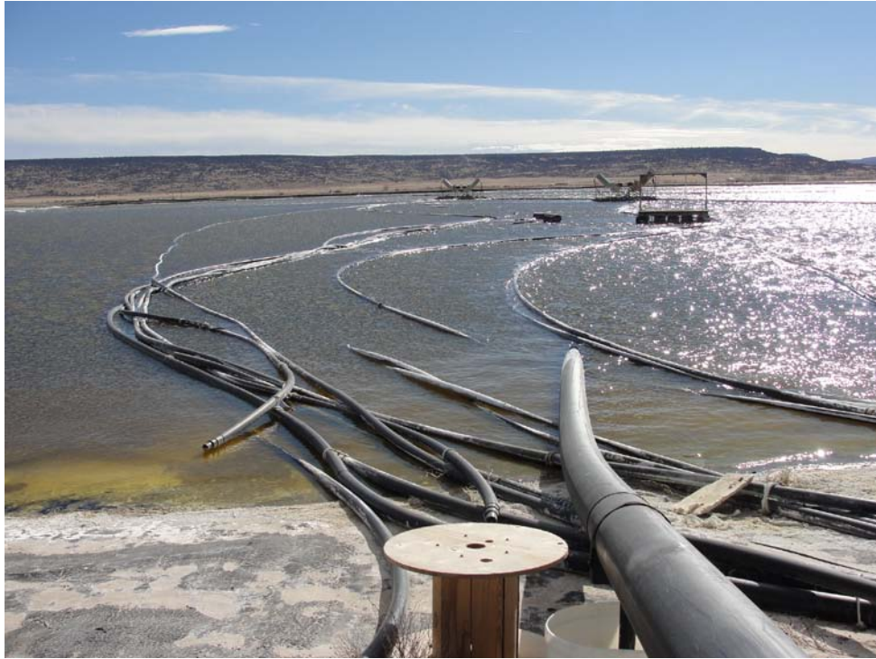
Photo 11: Evaporation Pond 1. Piping used to convey extracted groundwater from the large tailings pile to the evaporation pond and to the spray misters (structures in the center of the pond). View looking south.
