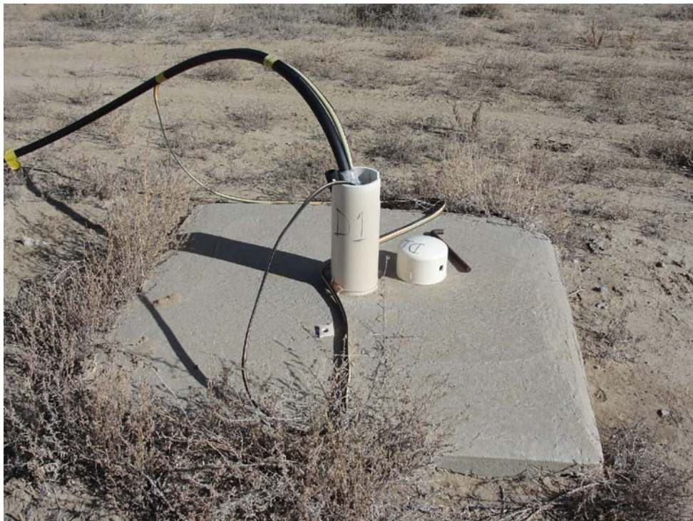
Photo 14: POC Well D1 near the RO treatment plant. Well D1 is a replacement well for the original POC Well D.
