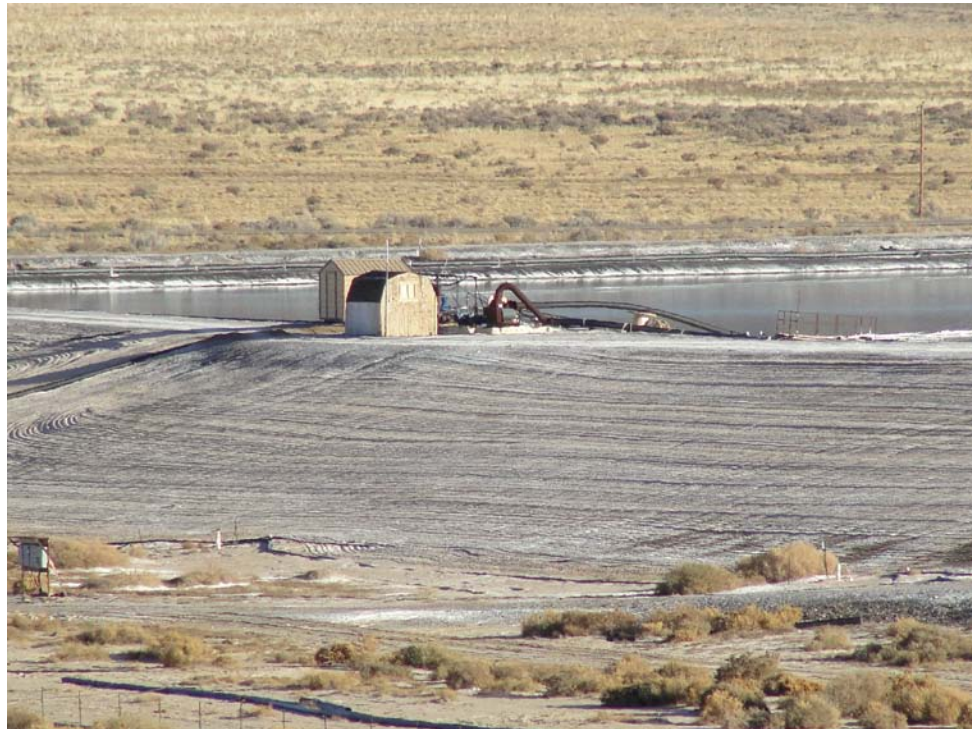
Photo 2: Pump house and equipment at Evaporation Pond 1. View looking southeast.
