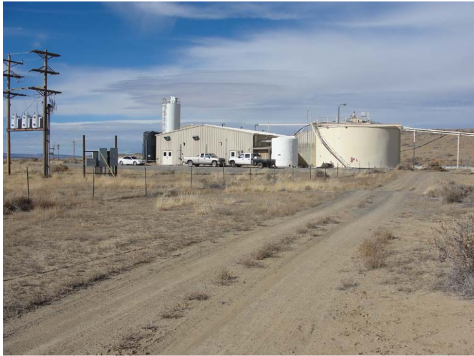
Photo 15: RO treatment plant. View looking west.
