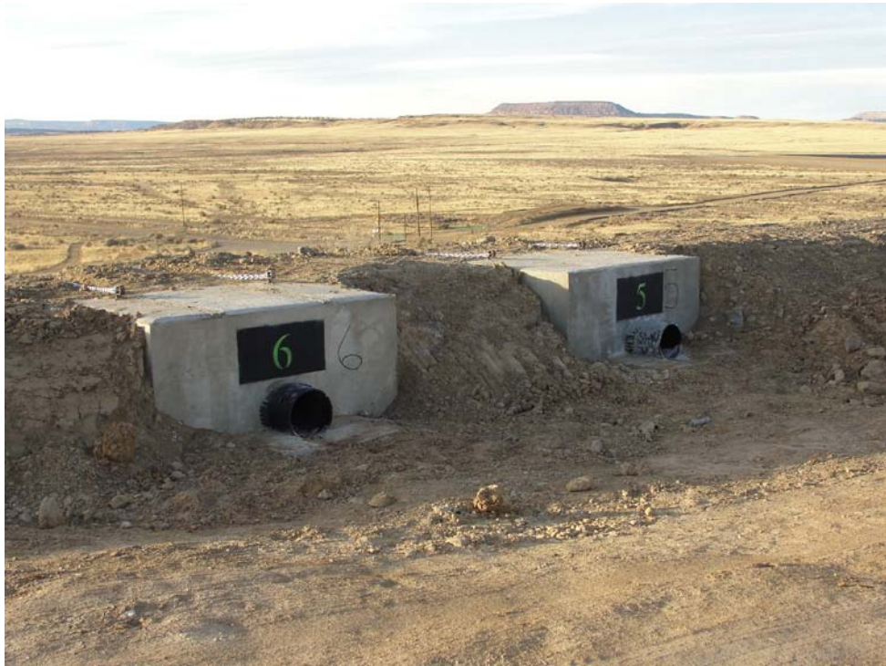
Photo 9: Two of 14 discharge structures used to convey surface water off of the top of the large tailings pile. View looking northwest.
