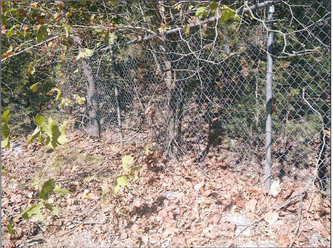
Photo 9: Breach in Perimeter Fencing On North Side
