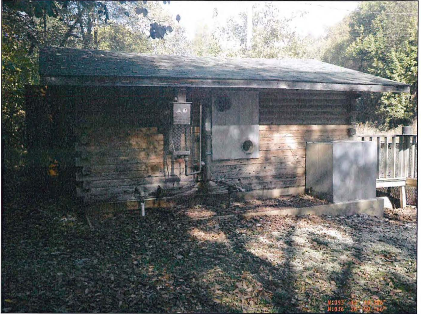
Photo 3: Ozone Treatment Station & Collection Sump
