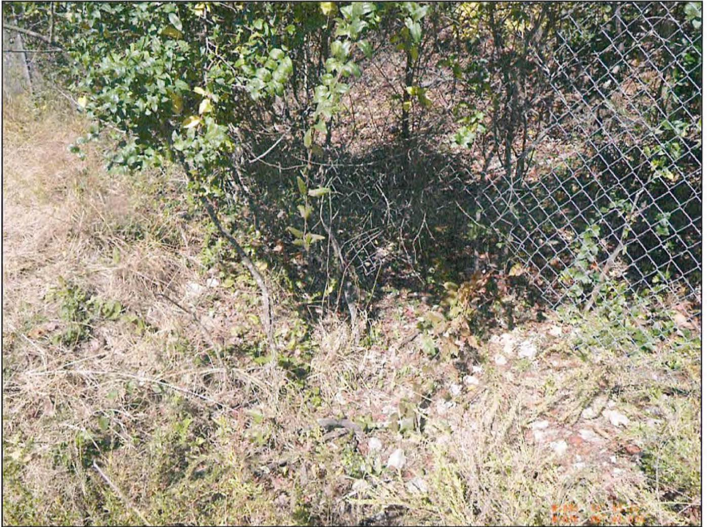
Photo 10: Breach in Perimeter Fencing On North Side
