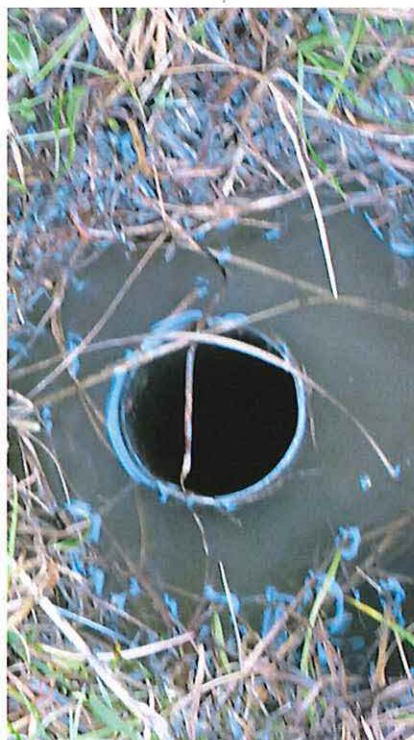
DNAPL recovery system piezometer BPZ 01, without cover and missing cap
