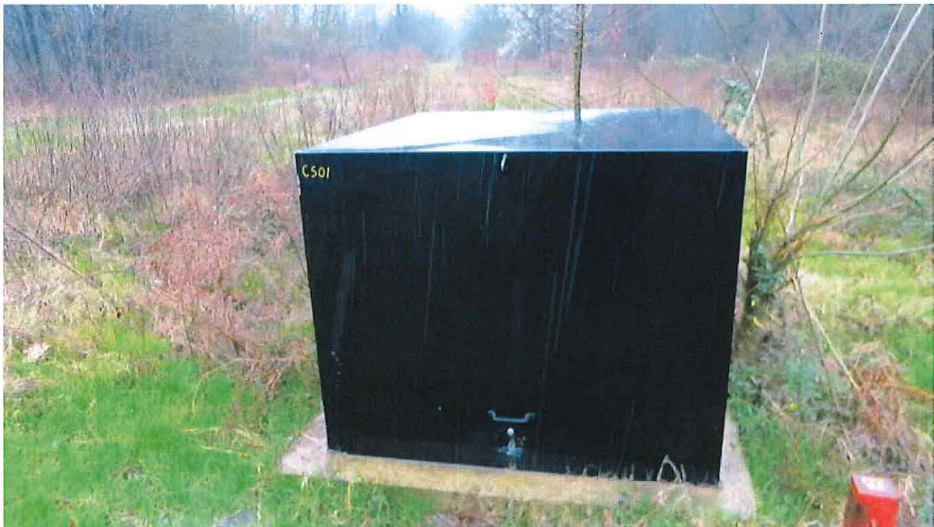
DNAPL collection sump, covered and locked
