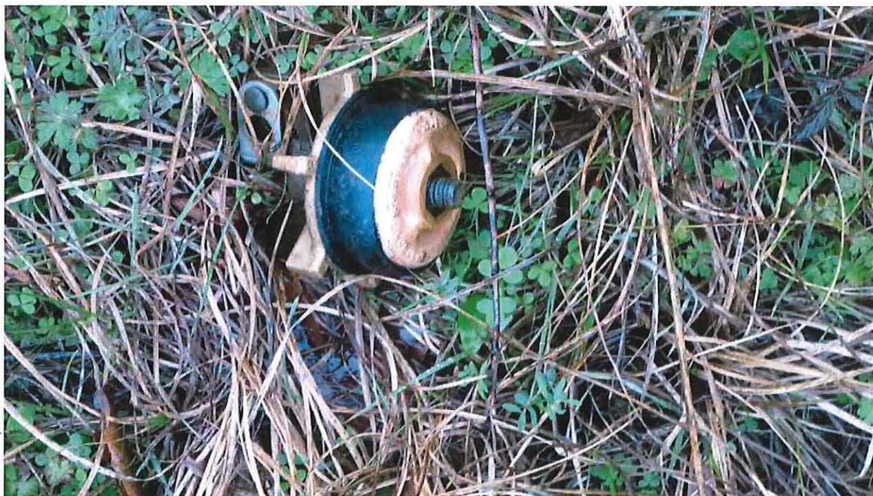
Well cap located near DNAPL recovery system piezometer BPZ 01
