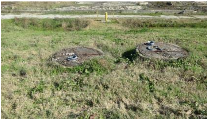
Sumps on top of the TRSF
