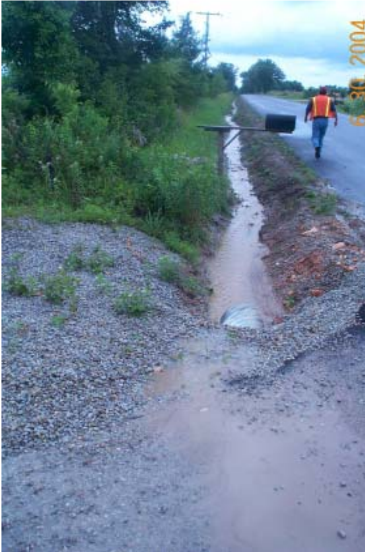
Photo 47: View upstream in the drainage ditch and culvert at entrance to borrow source. Runoff water in the drainage ditch is discolored from silt.
