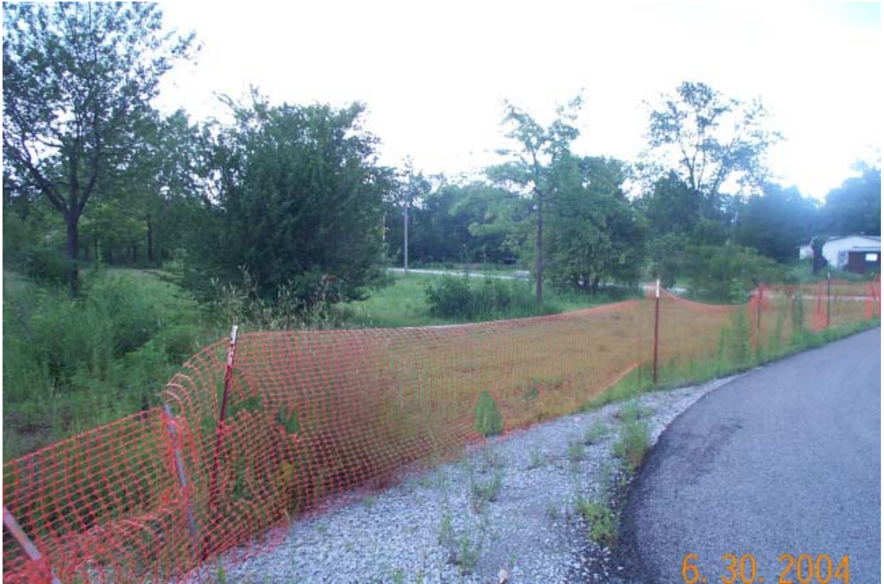
Photo 40: View of property under construction in Cardin, Oklahoma. There were still a few remaining items to complete on this property at the time of the site inspection.
