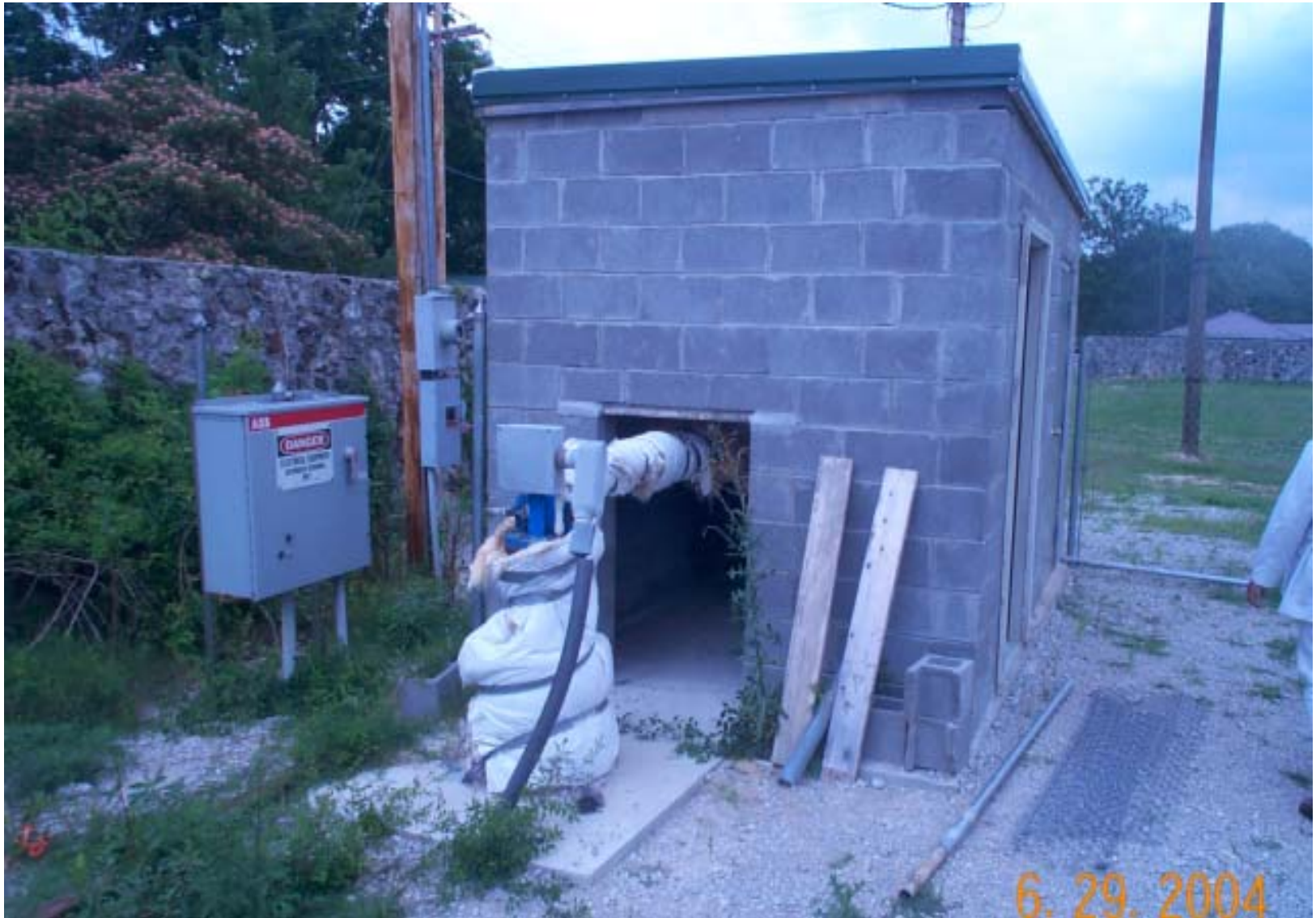
Photo 1: View of the Commerce #5 MW. The City of Commerce has erected a well house over the well-head in preparation for connecting the well to the public water supply.
