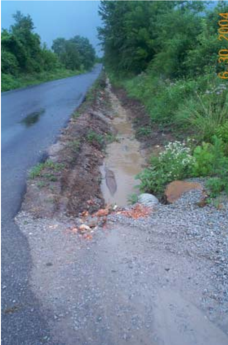
Photo 48: View downstream in the drainage ditch and culvert at entrance to borrow source. Runoff water in the drainage ditch is discolored from silt.
