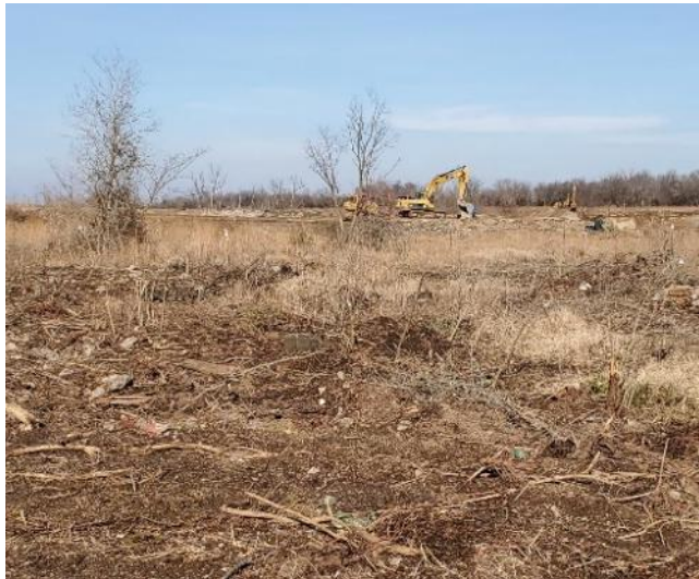
Distal 10a before remediation
