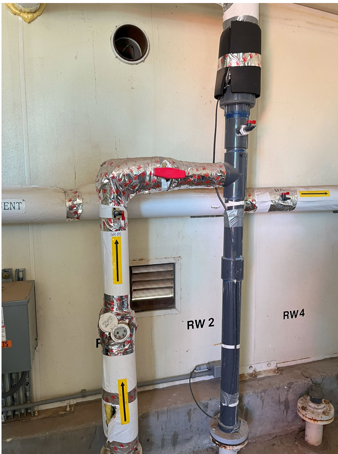
Photograph No. 2 Description: OU 03, Extraction Wells Influent and effluent from Old Treatment Building. Site: South Valley Superfund
