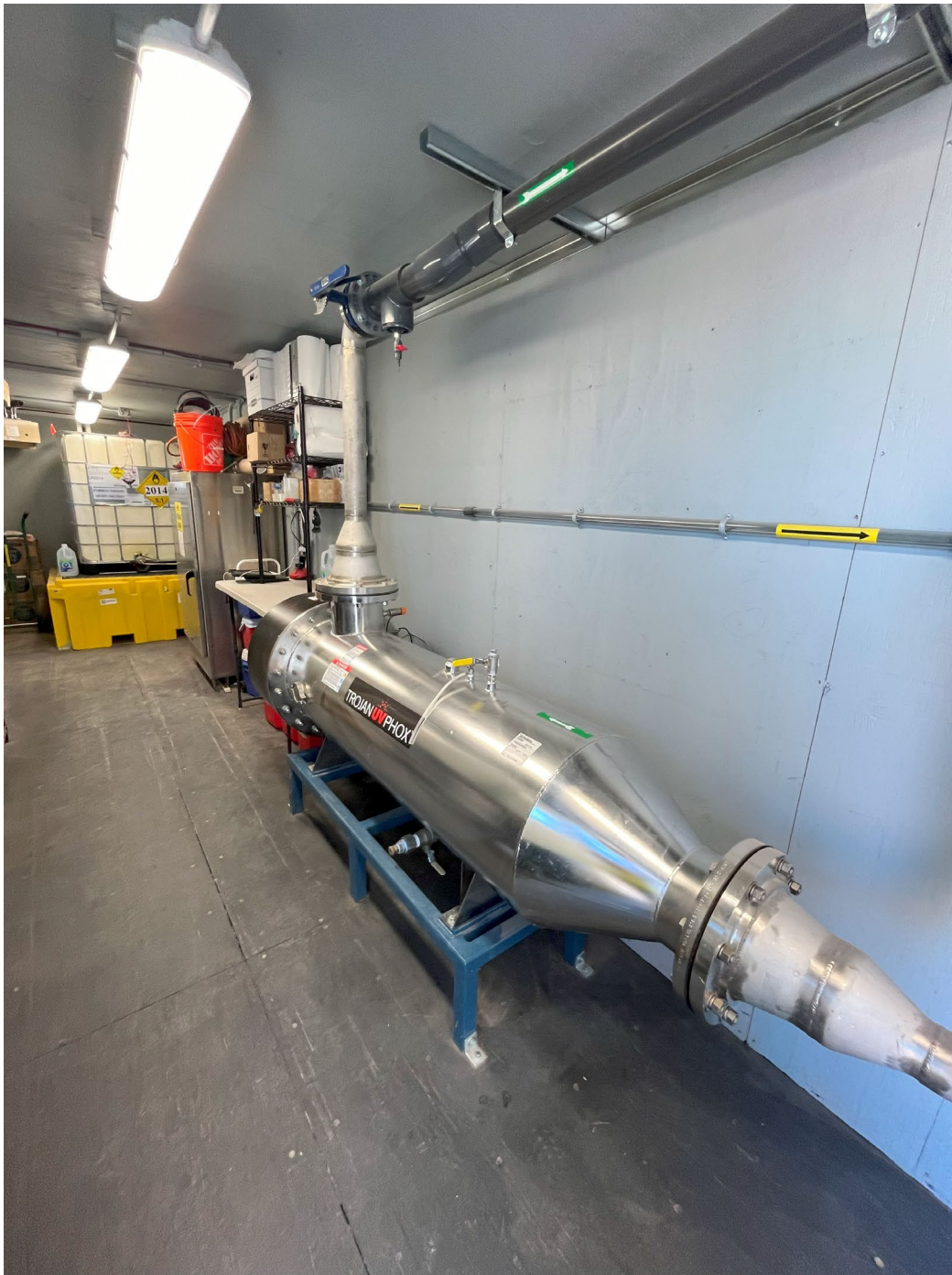
Photograph No. 4 Description: OU 03, UV Oxidation Unit and Hydrogen Peroxide tank in Treatment Building.
