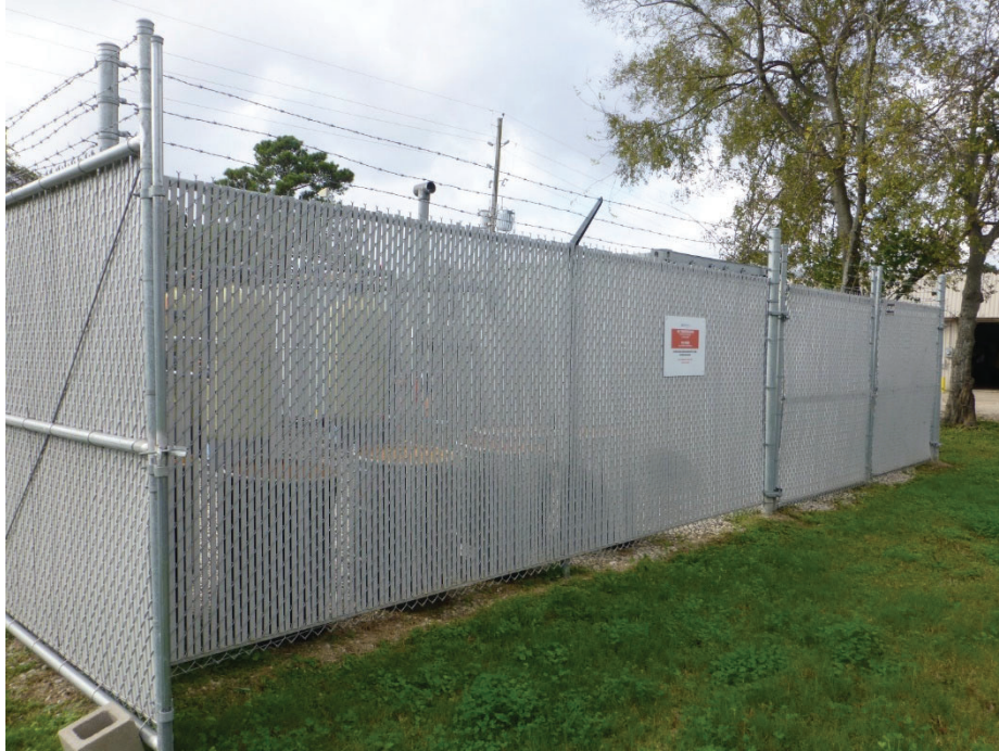
Fenced SVE system
