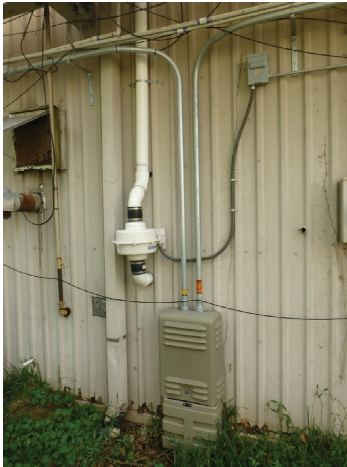
Vapor mitigation system
