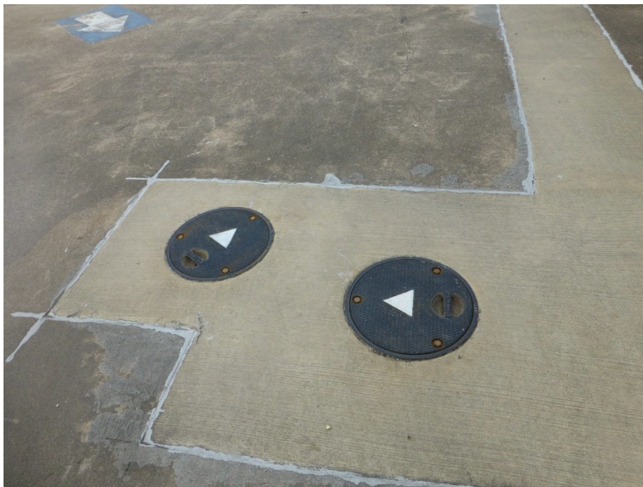
Monitoring wells in Cypress Shopping Centre
