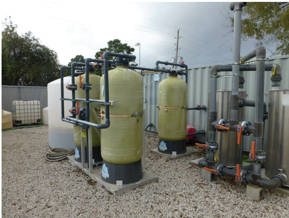
SVE treatment system
