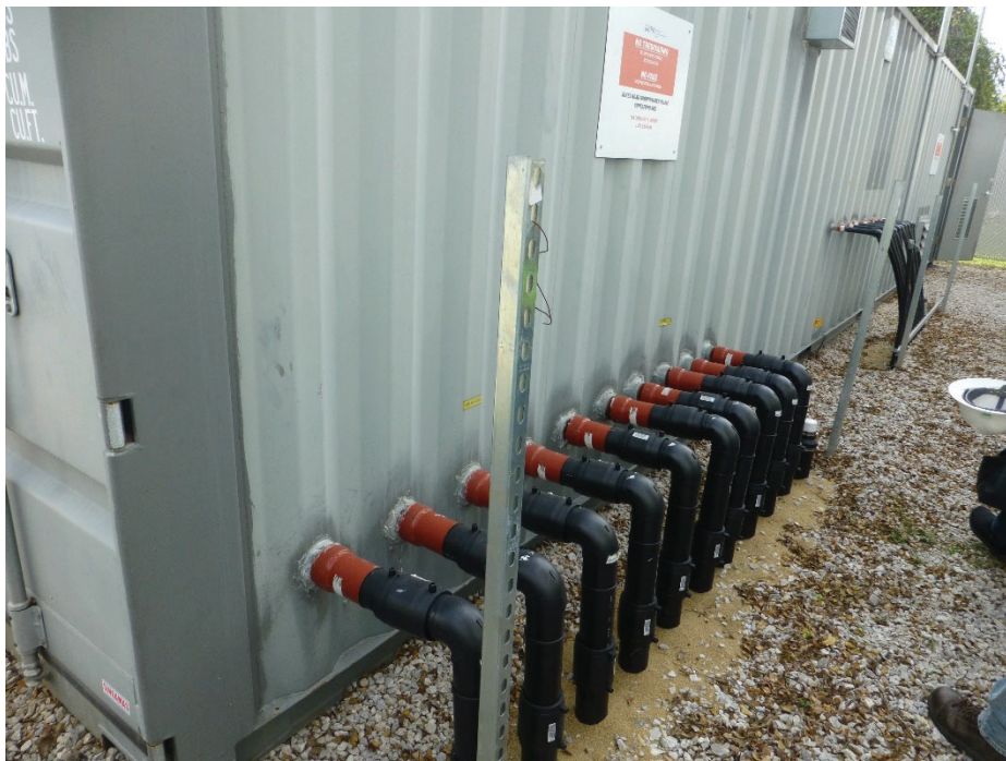
Deep SVE well lines
