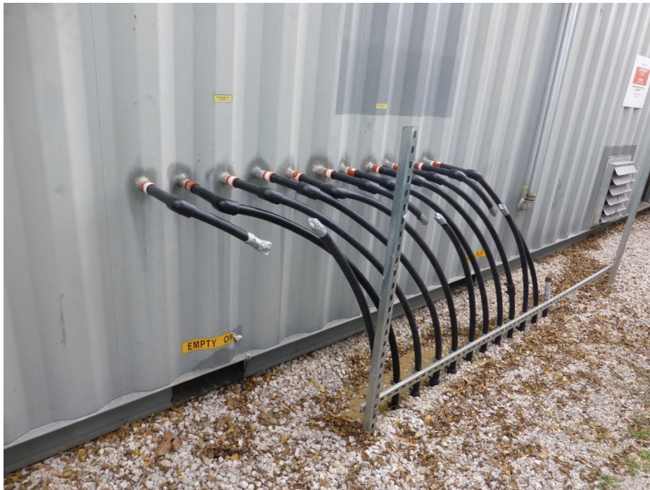
Shallow SVE well lines
