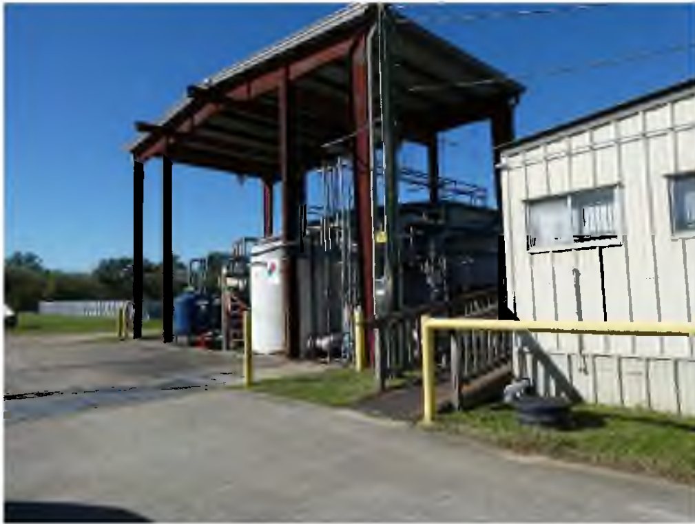
Groundwater treatment plant and site office, with aboveground storage ponds in the background
