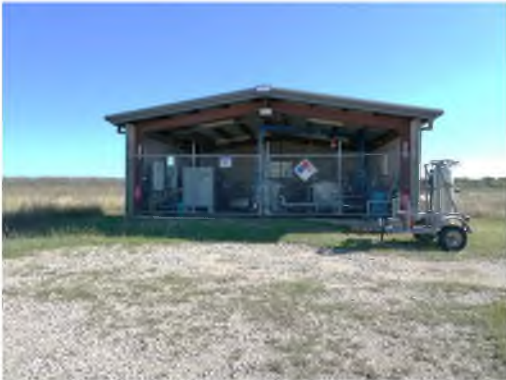
Brio North Hub B groundwater recovery system and gas collection vent (outside on the right of the building)
