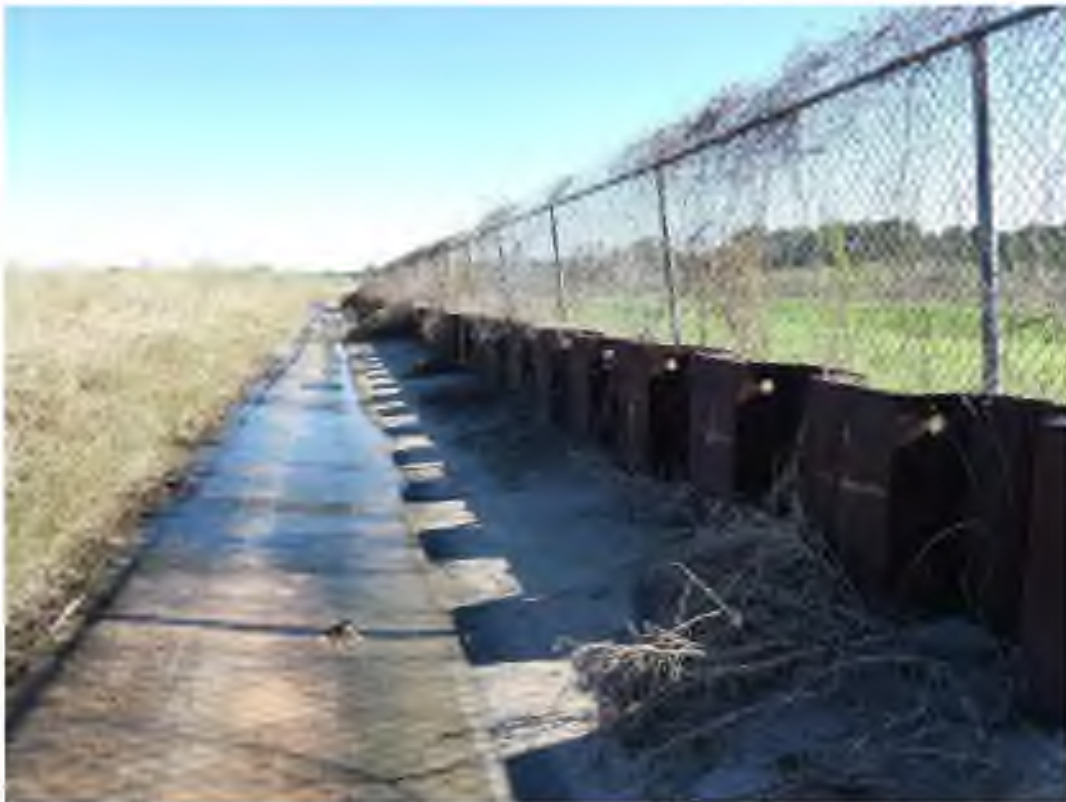
View looking east at the sheet pile along the Brio North southern boundary drainage road, with Mud Gully on the right
