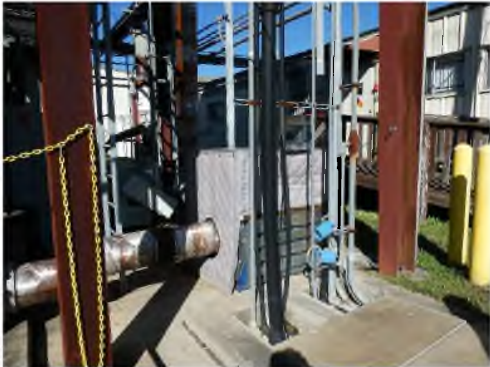
Air stripper blower unit, insulated to reduce noise
