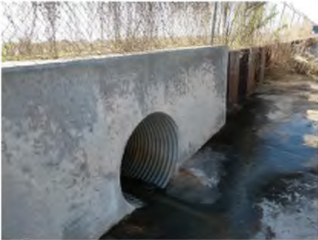
Surface runoff discharge to Mud Gully at the end of drainage road on the south end of Brio North
