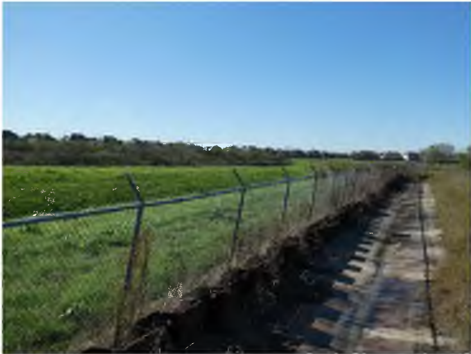
View looking west at the sheet pile along the Brio North southern boundary drainage road, with Mud Gulley on the left
