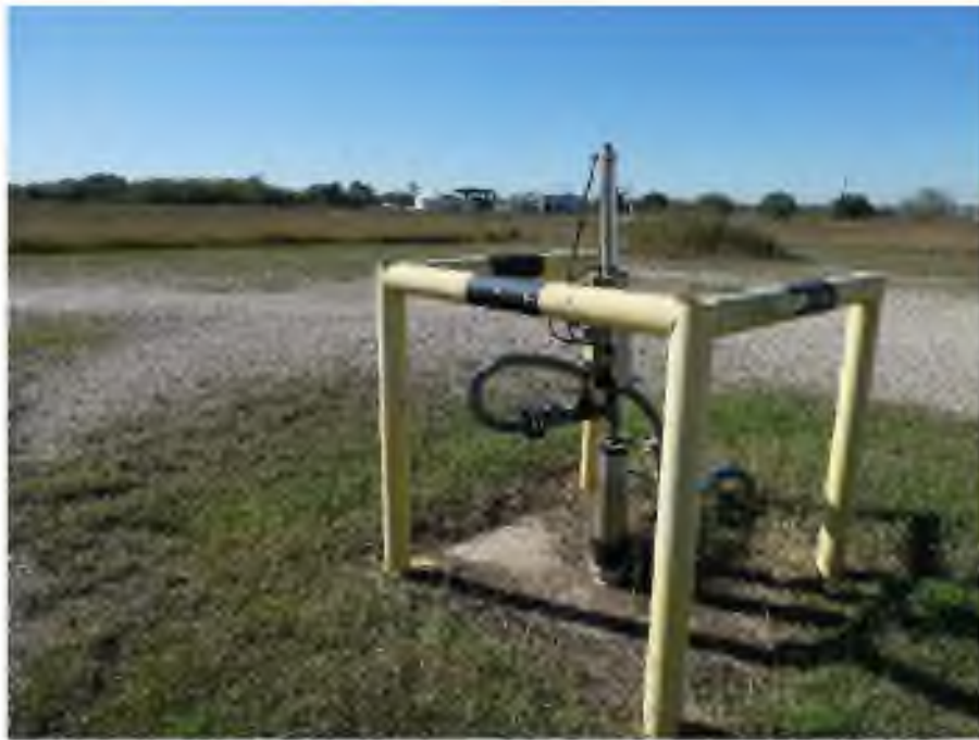
Brio North DNAPL recovery well near Hub B (groundwater treatment plant in background)
