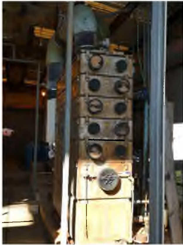
Groundwater treatment system air stripper
