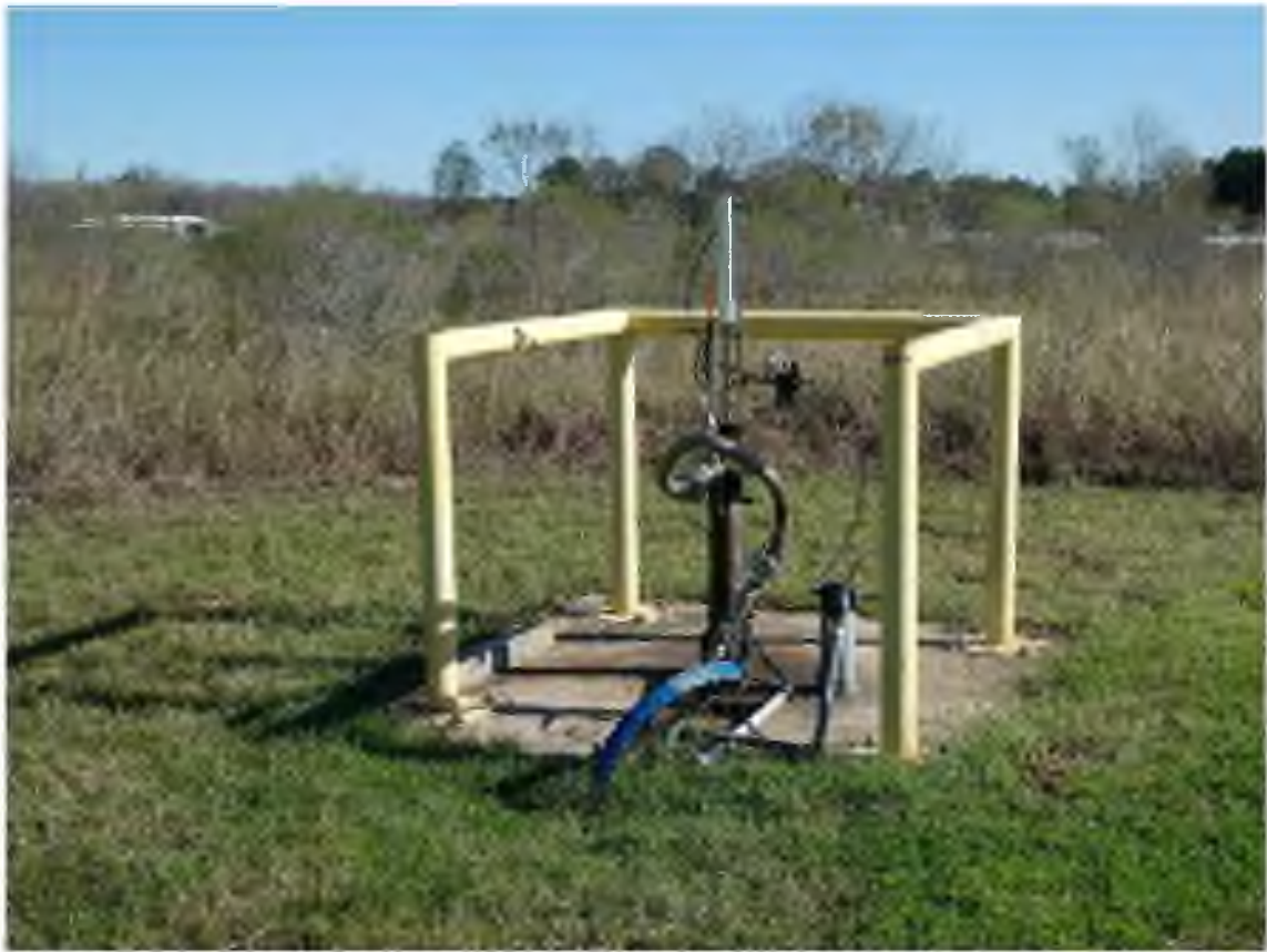
Brio South groundwater recovery well
