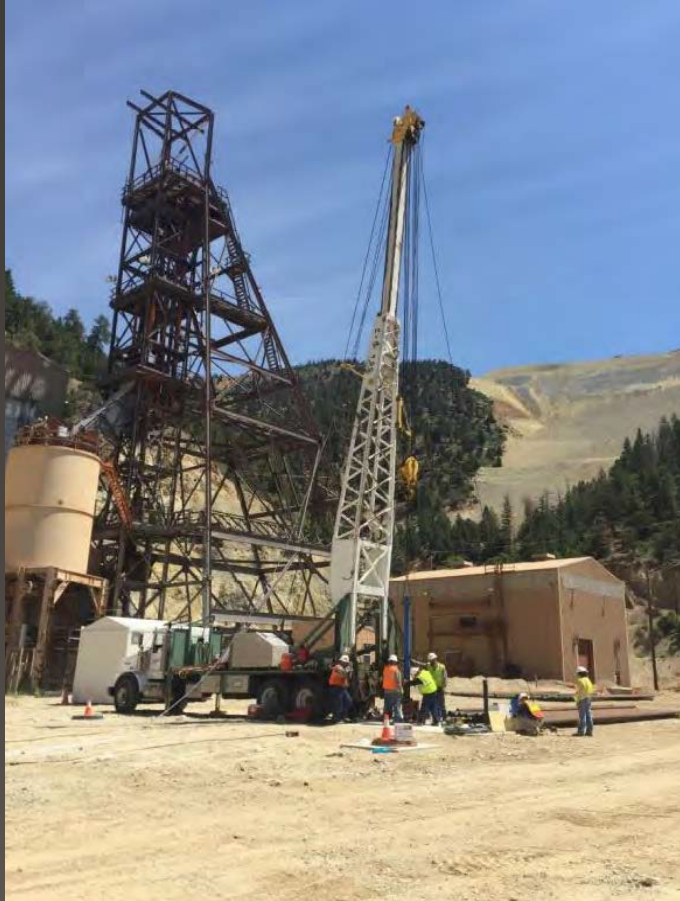
Underground Mine Dewatering System
