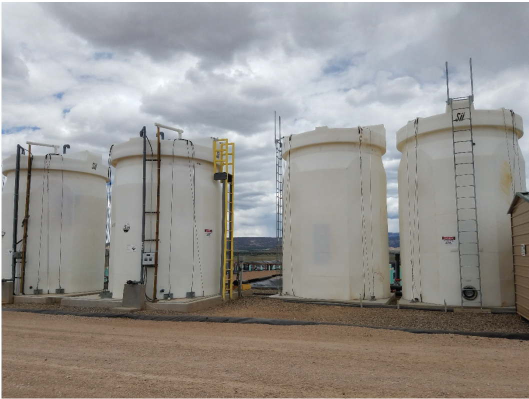
Zeolite treatment system tanks on top of the LTP
