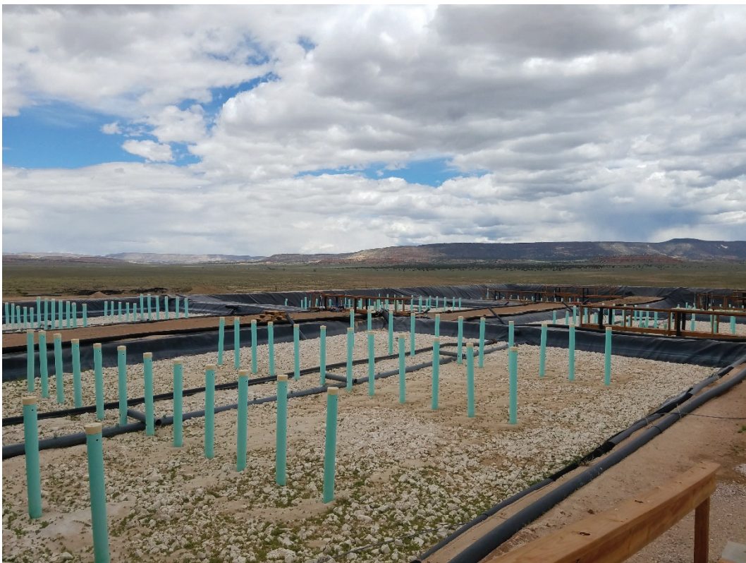
Zeolite treatment system
