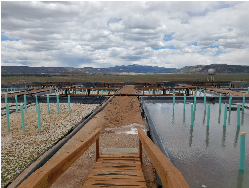
Zeolite filtration system on top of the LTP
