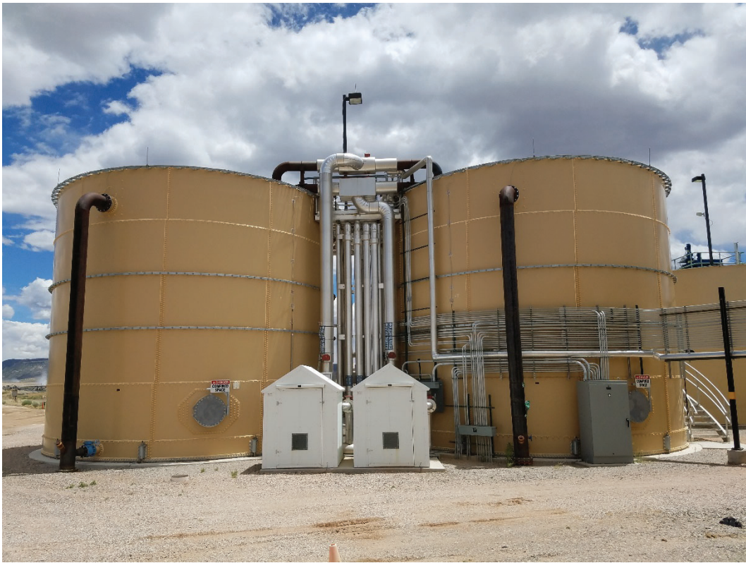
RO treatment plant storage tanks
