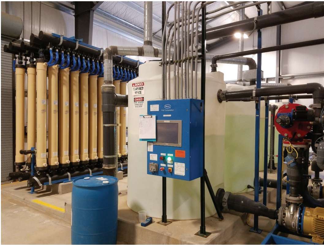
RO treatment plant interior
