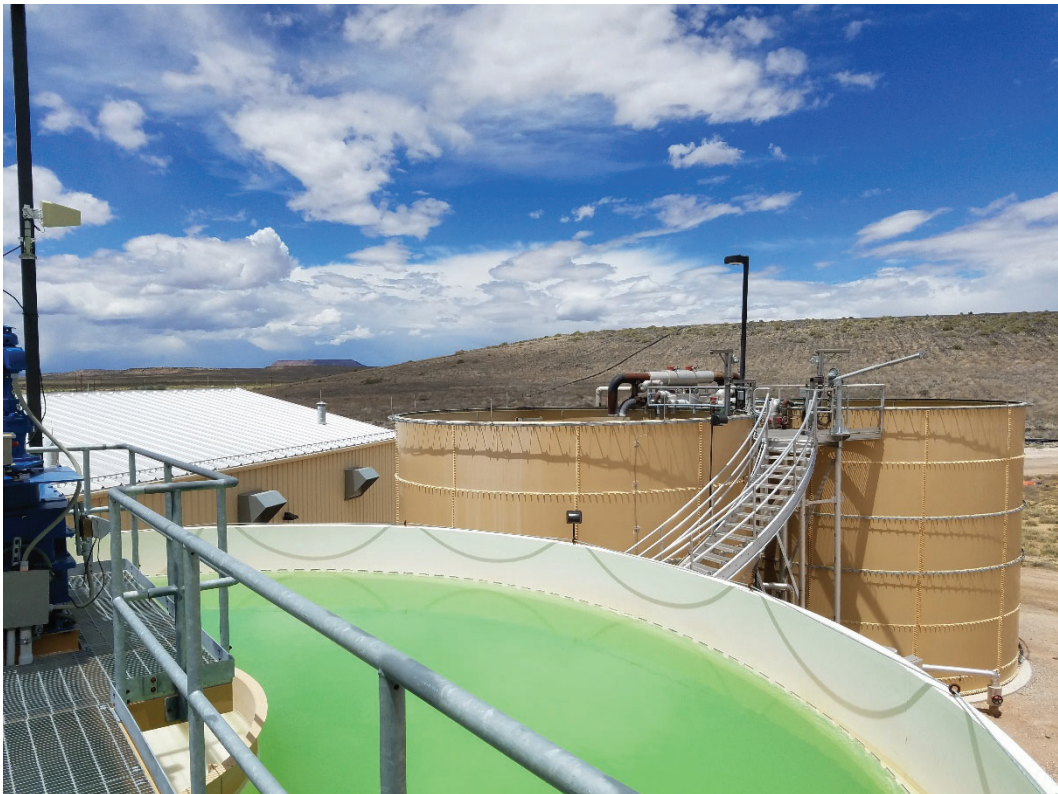
Top of RO storage tanks with LTP in the background
