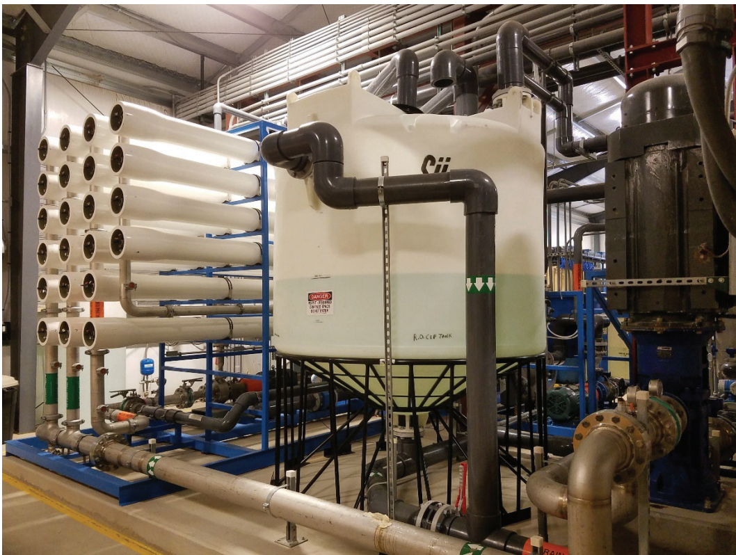
RO treatment plant interior
