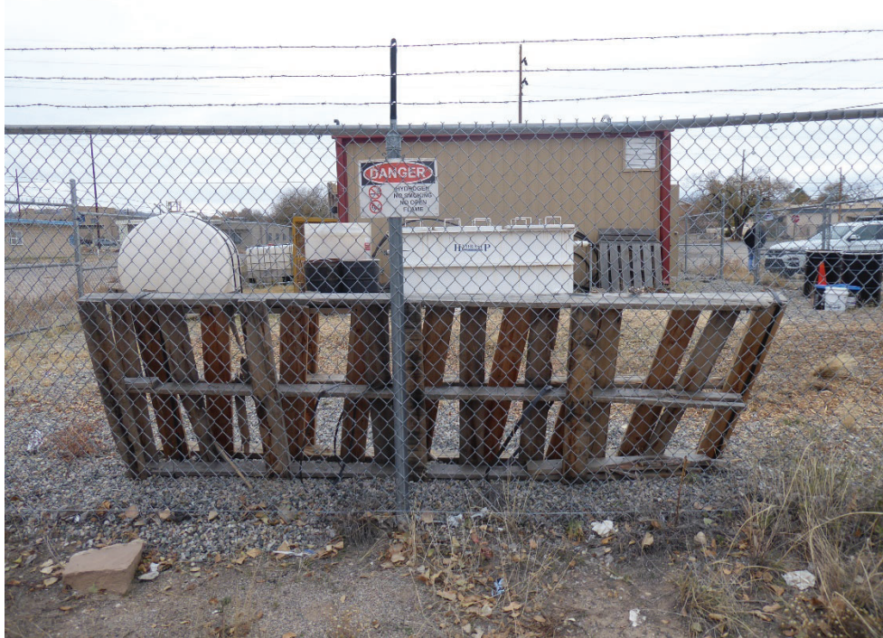
Photo7: Section of Fence on east side of the SA/HS enclosure that was cut by vandals and temporarily repaired with bailing wire. Photo looking west, DNAPL separator and building in background.
