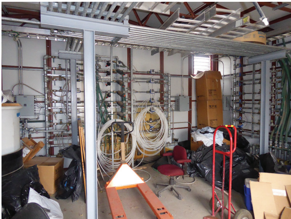
Photo 20: SA/HS building interior. Note injection and extraction manifolds mounted on the walls. The boxes in the corner contain auto samplers from the unexecuted SEAR. Photo looking south-southwest.
