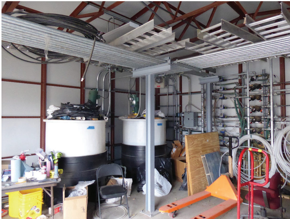
Photo 19: Southeast corner of SA/HS building. Note mixing tanks and mixers. Photo looking southeast.
