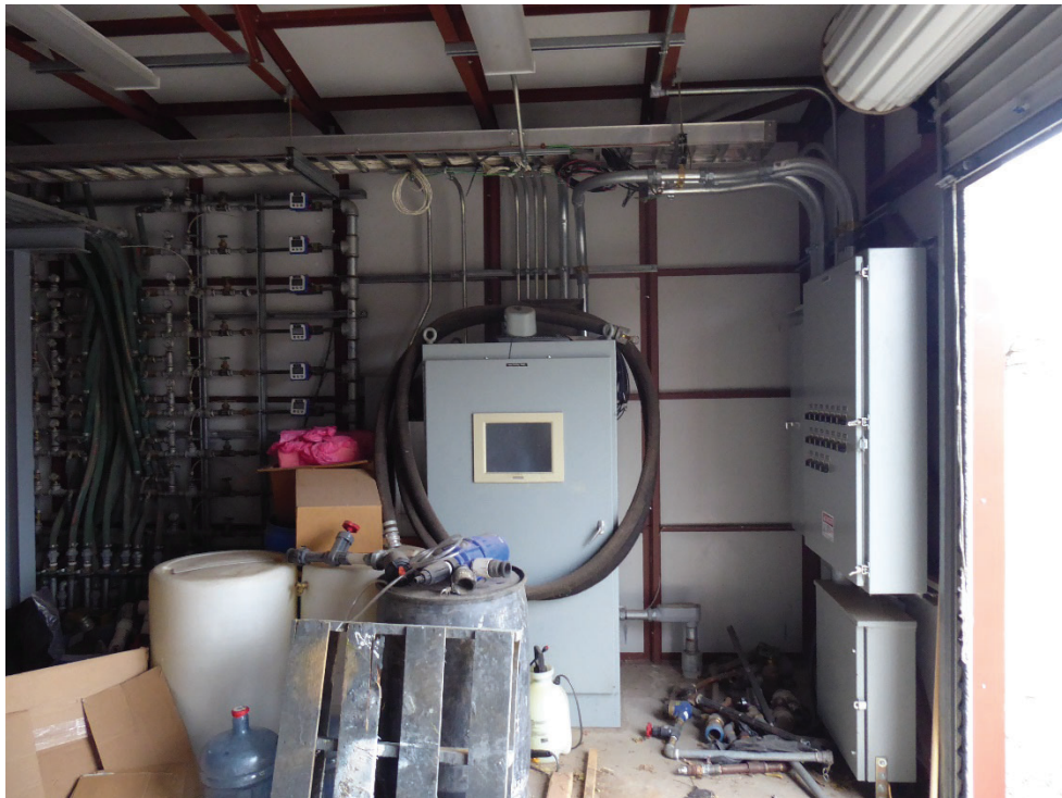
Photo 22: From left, manifold, SCADA cabinet with HMI panel, and breaker boxes/pump control cabinets in the SA/HS building. Photo looking west.
