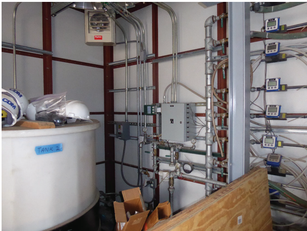
Photo 18: Interior (SE corner) of the SA HS building. The hydrogen injection system is shown in the center of the photograph. Photo looking southeast.
