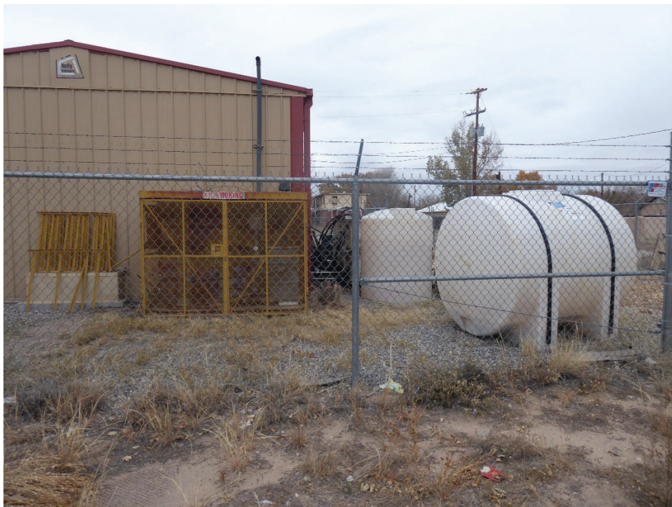
Photo 16: Tanks and SVE enclosure on the south side of the SA/HS Building. Photo looking north-northeast.
