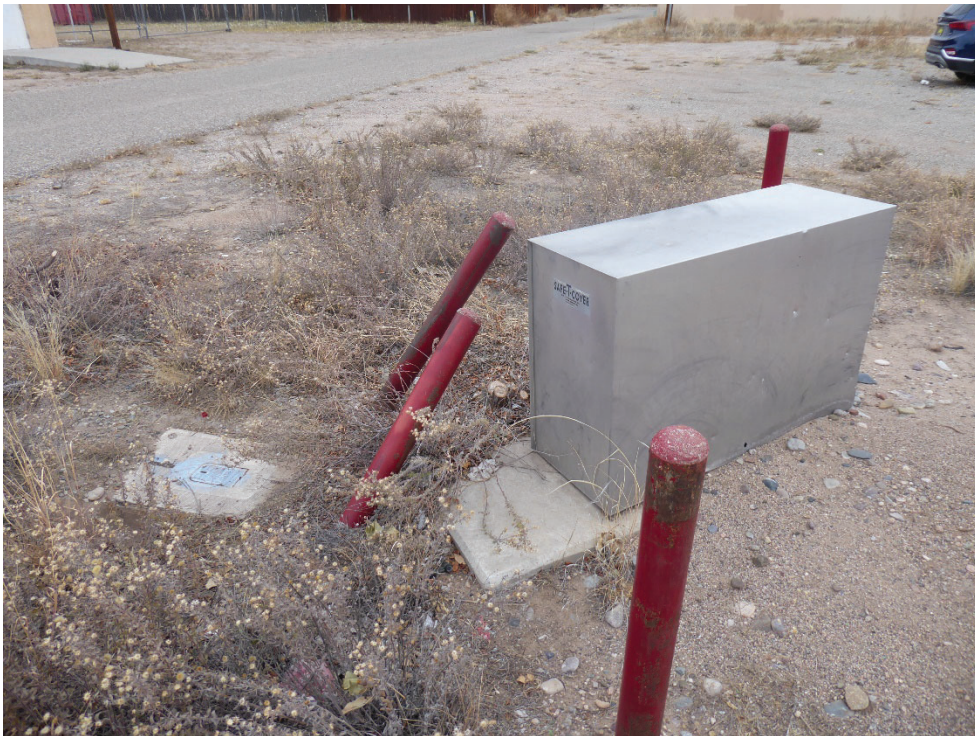
Photo 6: Hot Box over the backflow preventer installed on the water line that formerly serviced the Source Area/Hot Spot (SA/HS) building. Photo looking northeast. Note that bollards protected the box from damage.
