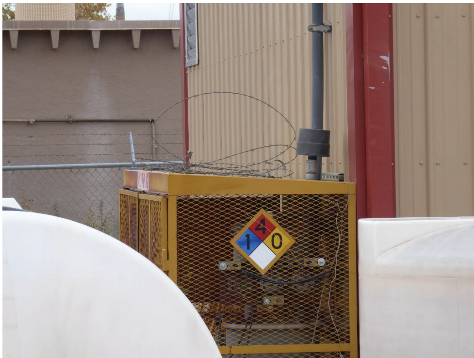
Photo 12: Placarded SVE/hydrogen storage enclosure on south side of SA/HS building. Photo looking west.
