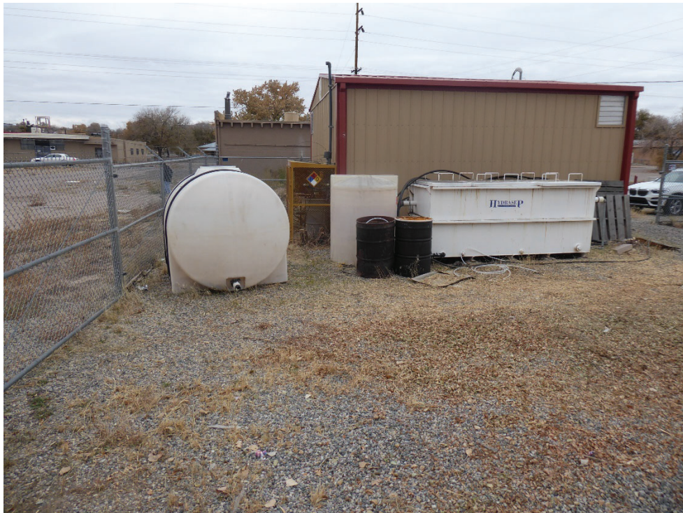
Photo 10: Tanks, DNAPL separator, and building inside of the SA/HS enclosure. Photo looking west.
