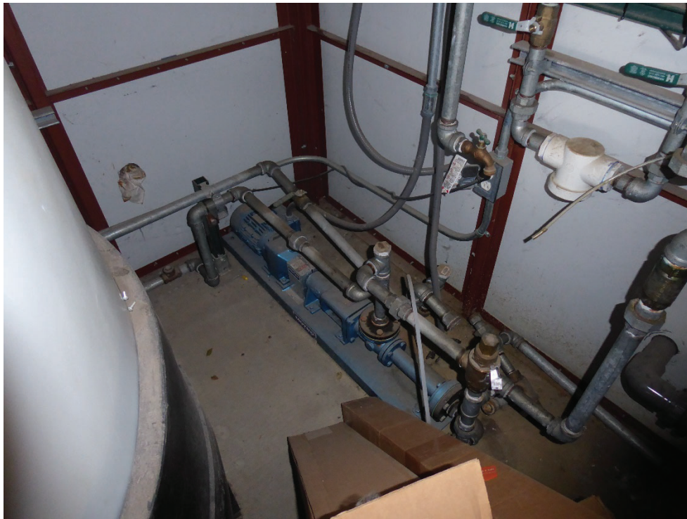
Photo 13: Existing unused injection pump in the SA/HS building. Photo looking southeast.
