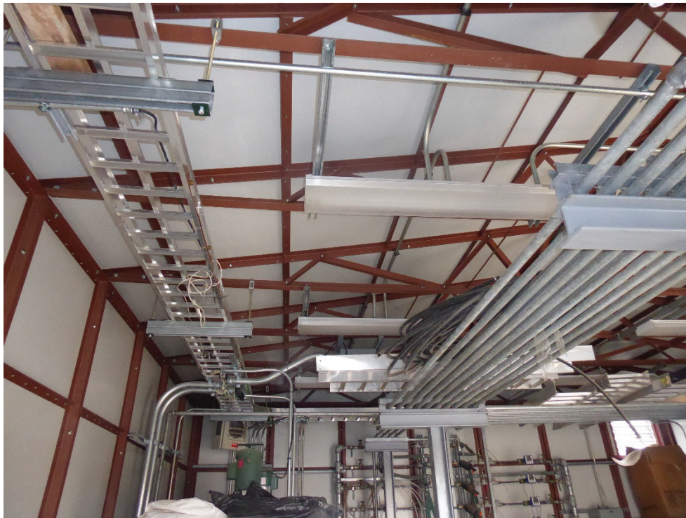
Photo 9: Interior of the SA/HS building, showing overhead conveyance pipe and conduit (looking south).
