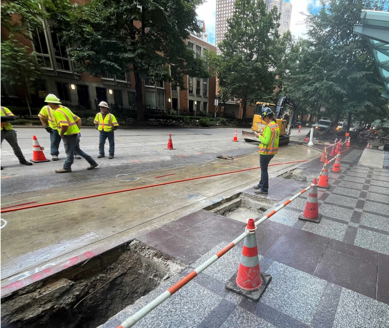
PICTURE 5: VIEW OF EXCAVATION ON SIDEWALK INFRONT OF 415 E NORTH WATER STREET CONDOS, FACING NORTHEAST.
