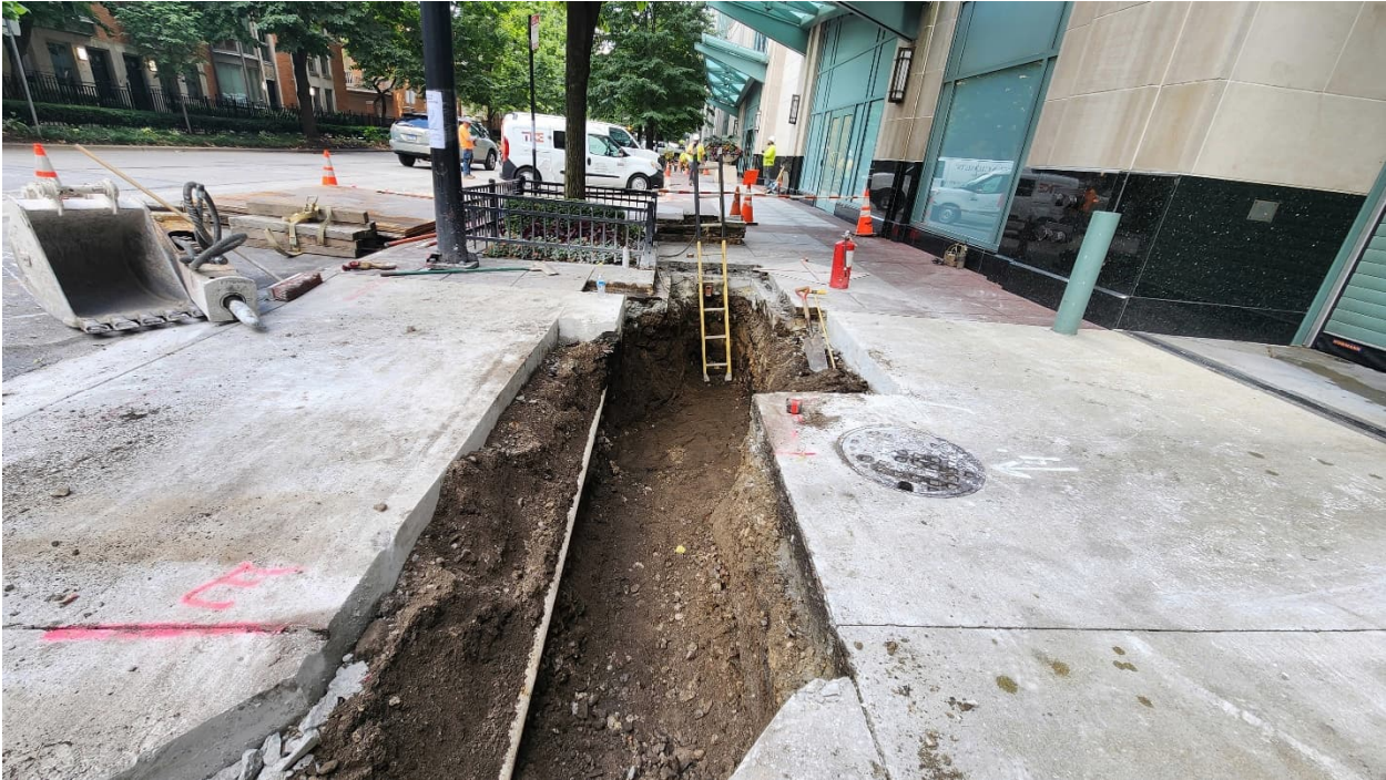
PICTURE 6: VIEW OF EXCAVATION, FACING EAST, COMPLETED ALONG DRIVEWAY LEADING INTO THE RIVERVIEW RECEIVING GARAGE.
