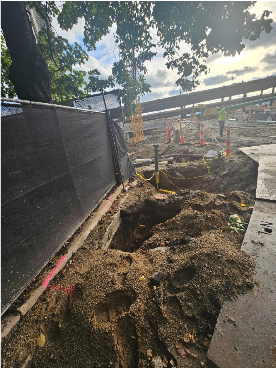
PICTURE 2: VIEW OF EXCAVATION FACING EAST, INSIDE OF THE 400 LSD PROPERTY GATE.
