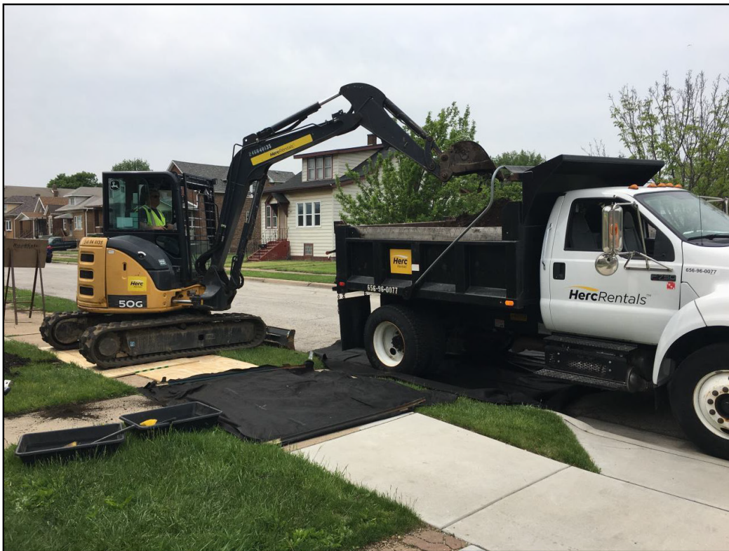
This is what typical soil excavation work looked like in yards near Federated Metals. Grass, trees and vegetation were restored after the contaminated soil was removed.
