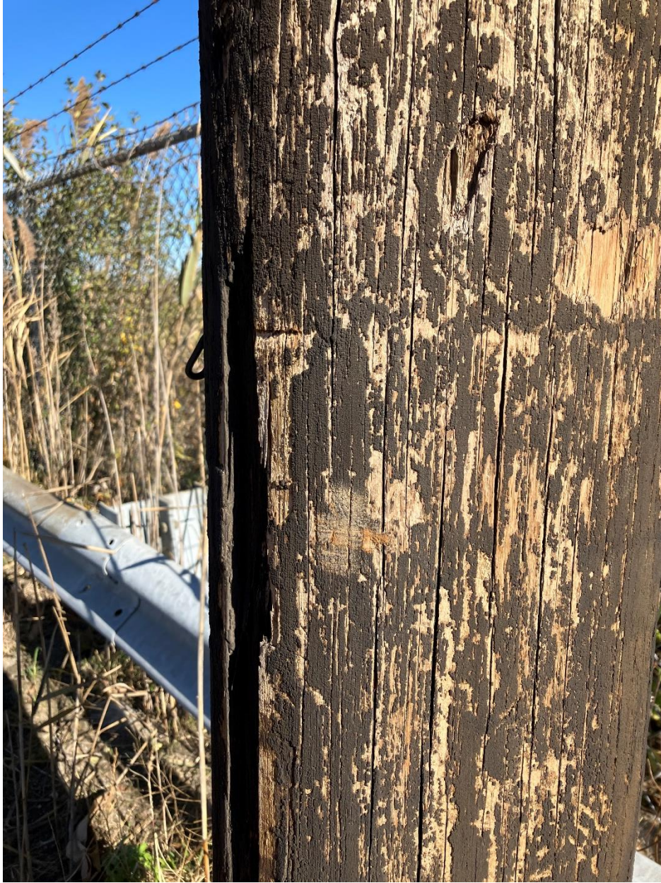
Closeup of the utility pole near well MW-4S coated from its base to approximately 5 feet with a dark substance.
