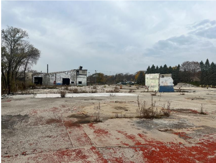
View southwest of Amcast North showing the partially demolished building, old underground parking access, and paved areas.
