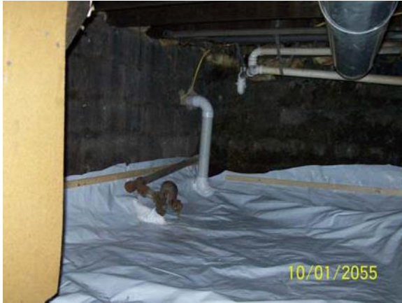
Figure 9-21. Piping Beneath Membrane
