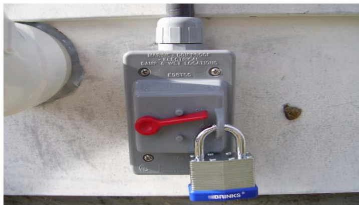
Figure 9-17. Electrical Box with Switch, Equipped with a Lock
