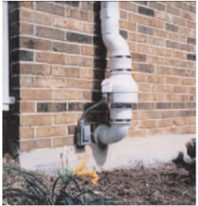
An example of a system that draws radon and other vapors out of the soil and vents them outside. It's known as a “sub-slab mitigation system.”
