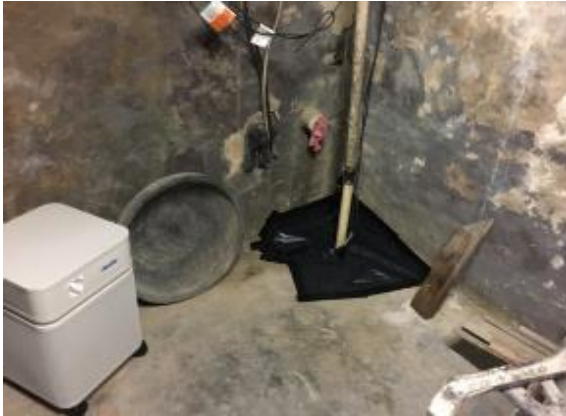
Figure 9-6. Sump Temporarily Sealed with Plastic and Tape
