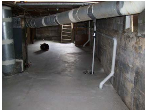
Figure 9-23. Basement with New Concrete Floor and SSDS
