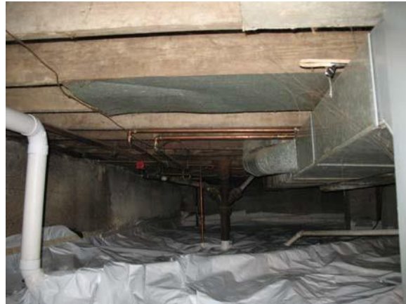
Figure 9-22. Piping in Crawl Space
