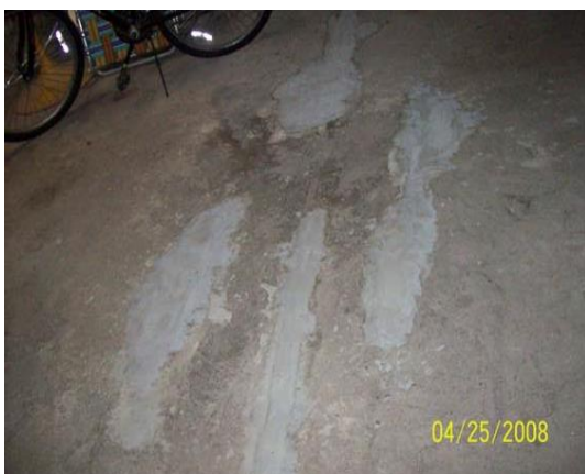
Figure 9-2. Cracks in Floor Sealed with Hydraulic Cement
