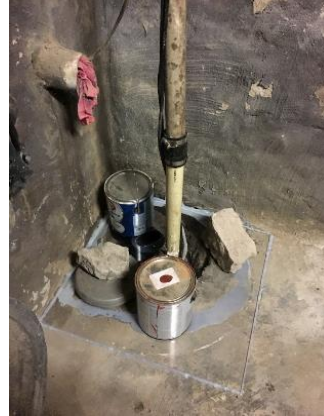
Figure 9-7. Sump More Permanently Sealed with Plexiglass Cover and J-Valve
