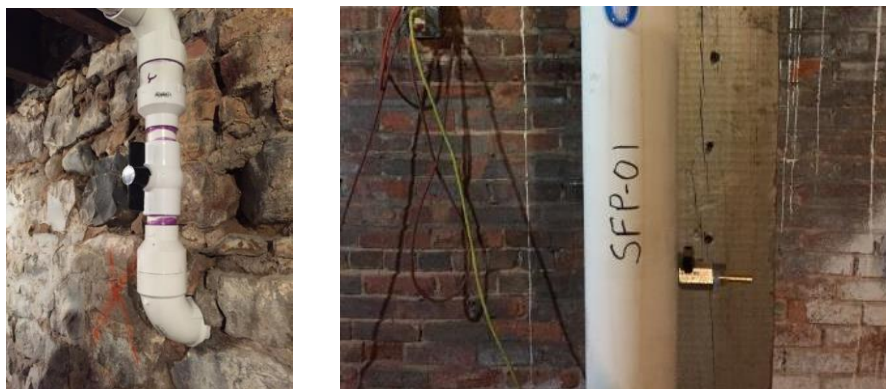
Figure 9-14. Installations of Flow Adjustment Valves (Left) and Sampling Ports (Right) on Piping
