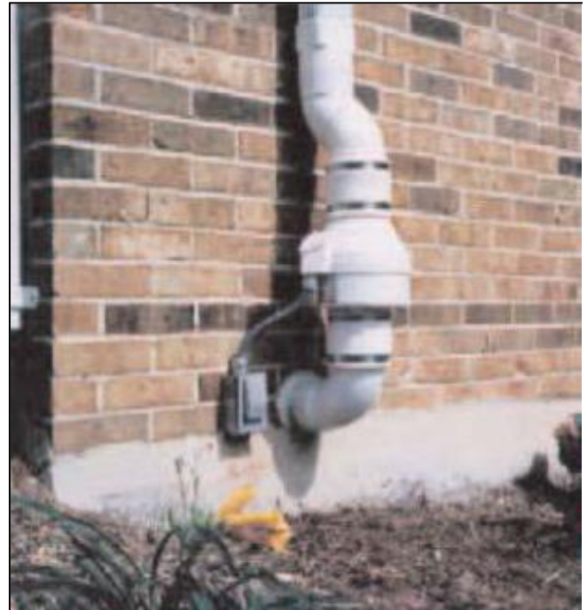
This photo shows a system that draws vapors out of the soil from below a structure and vents them outside of the building. This is known as a “sub-slab vapor mitigation system”, which is the same type of system used for radon mitigation.
