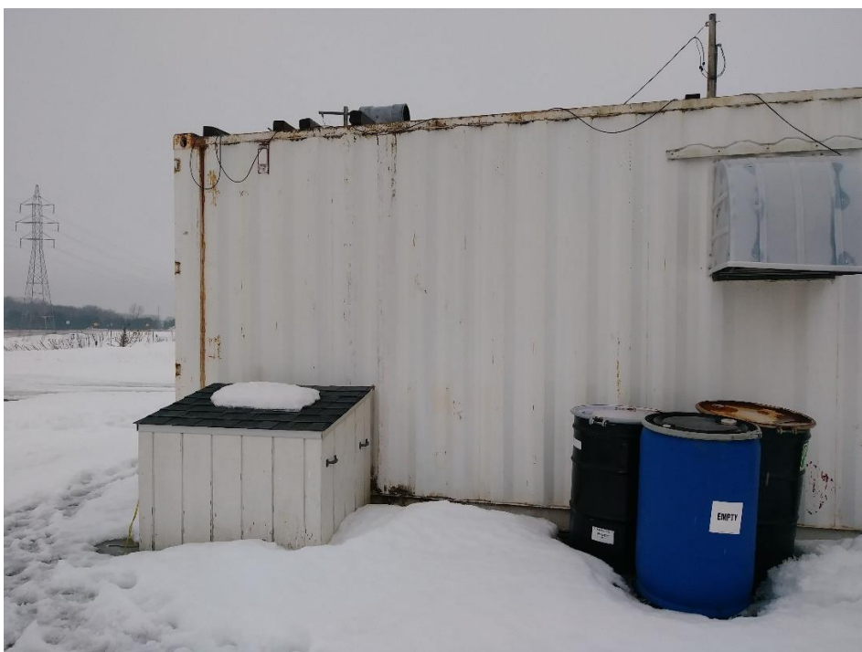
Photo 5: Treatment System Trailer, South Side
