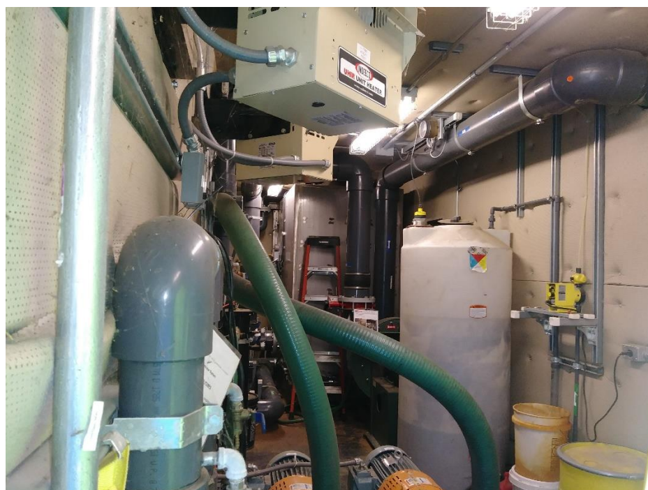
Photo 10: General view of inside treatment system trailer
