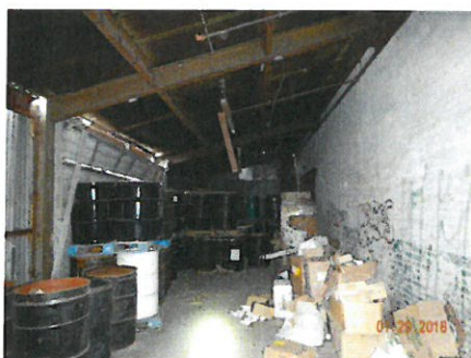
DSCN0042 –East area. Drums used to secure against entry.
