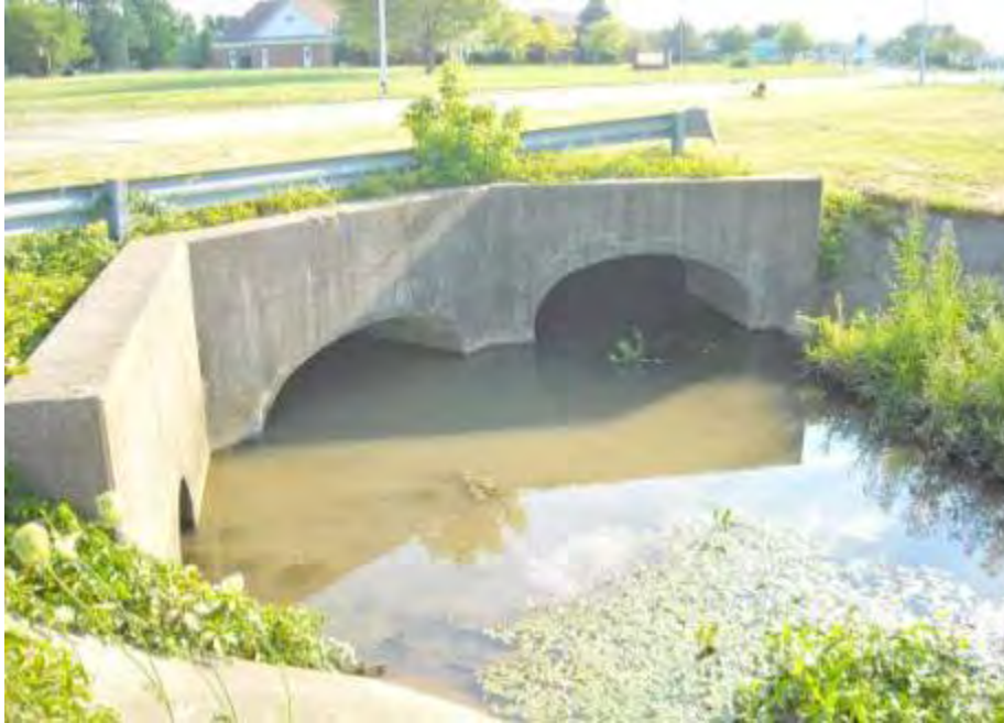
Figure 3-19 Three large culverts are located immediately upstream of the Amlosch Ditch sampling location (AD-1). The center culvert transmits upstream flow beneath Dustin Road.
