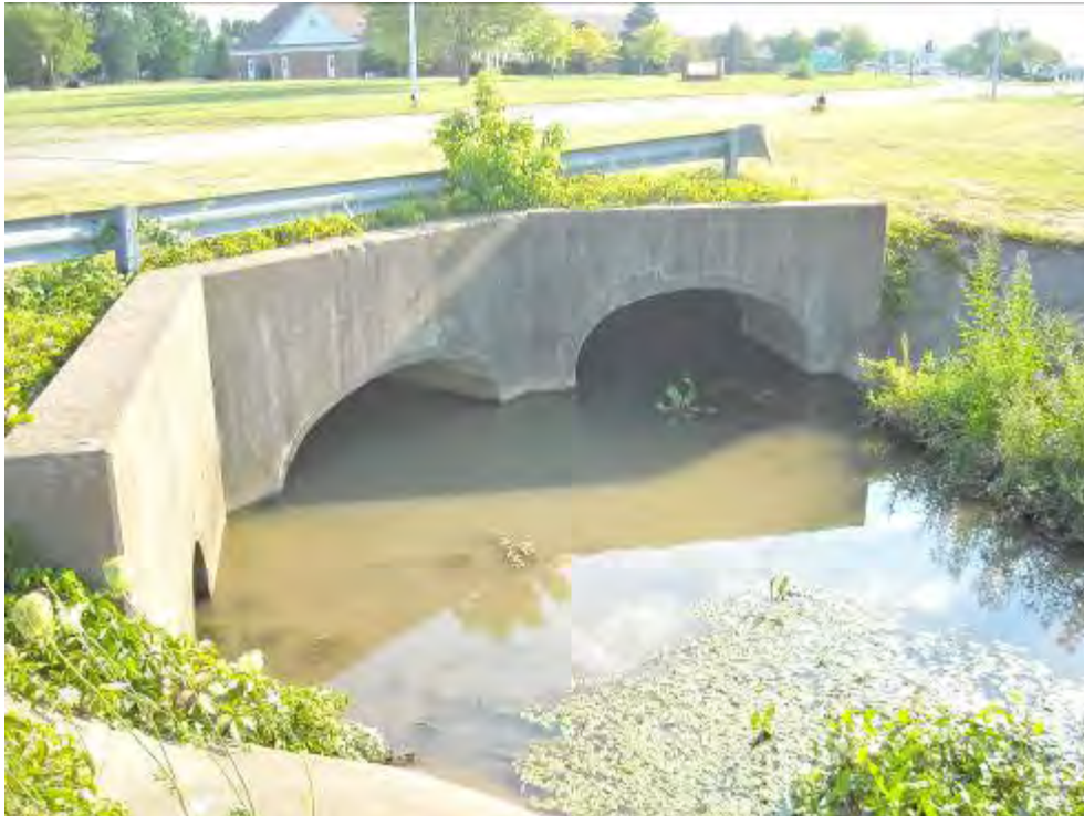
Figure 13. Amlosch Ditch receives storm water from large underground pipes at Dustin Road on Oregon, Ohio. DGI sample AD-1 was collected near this area.
