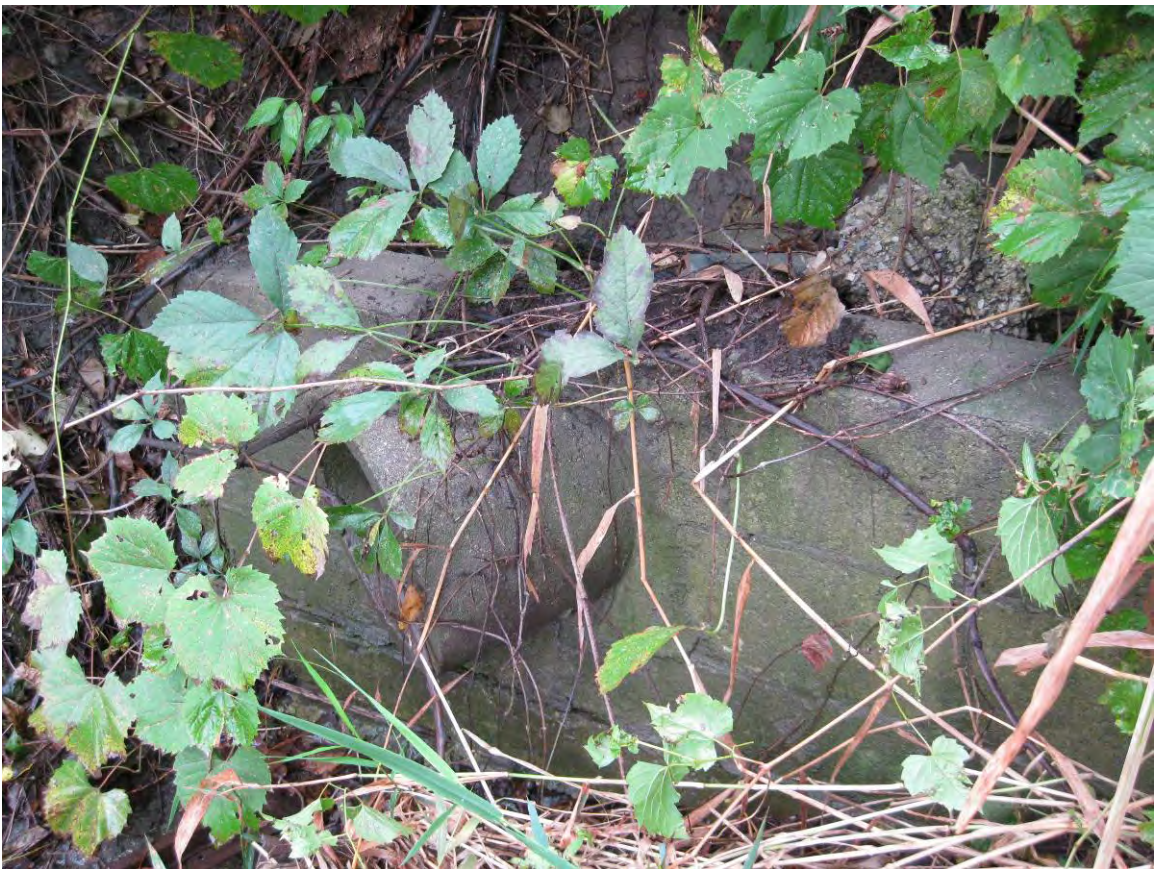
OC-16 Photo 3: Outfall pipe along Otter Creek.
