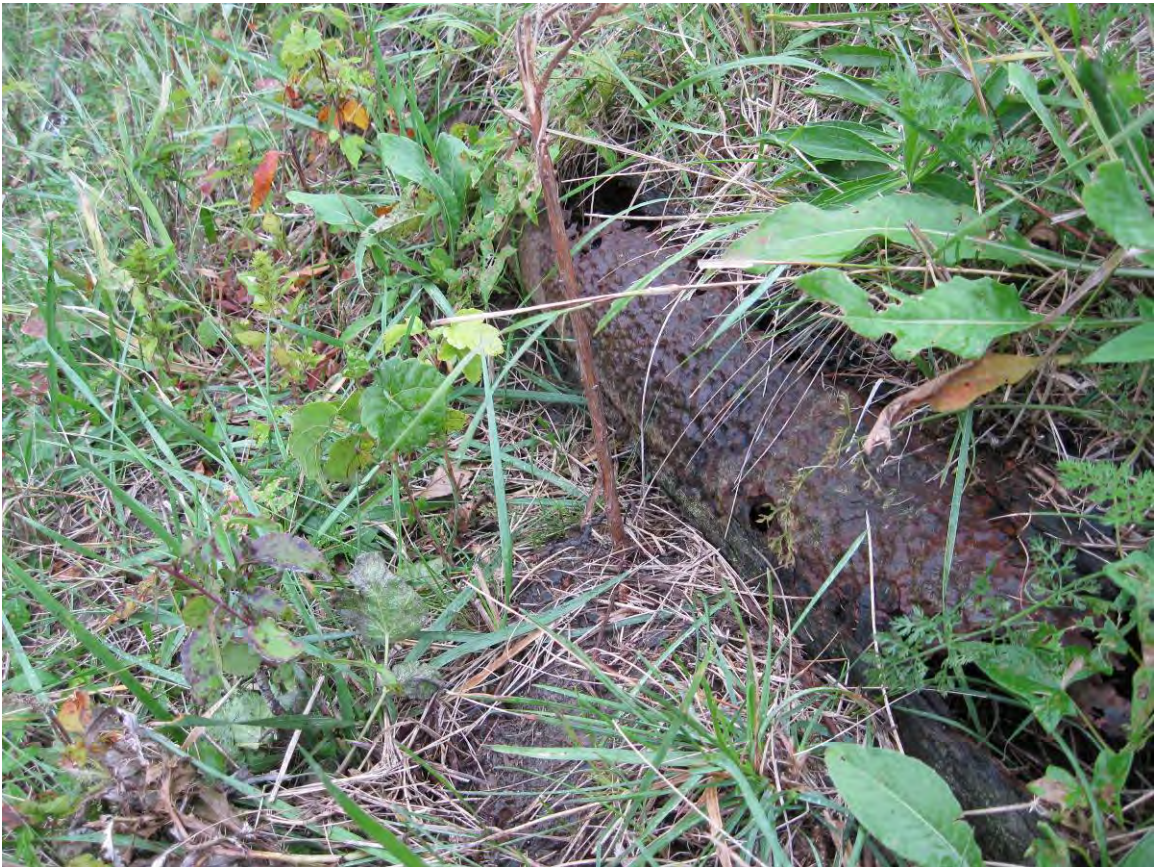
Amlosch Ditch Photo 2: Deteriorating outfall pipe along Amlosch Ditch.
