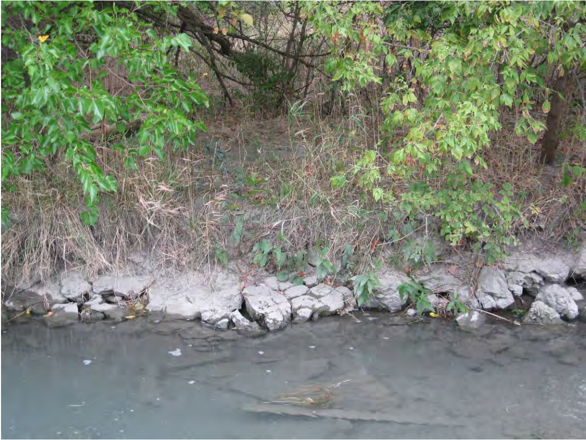
OC-9-10 Photo 5: Boulders along Otter Creek.
