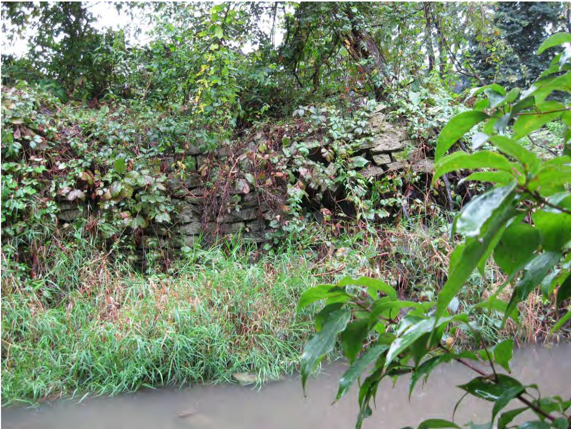
OC-22 Photo 6: Outfall pipe along Otter Creek.
