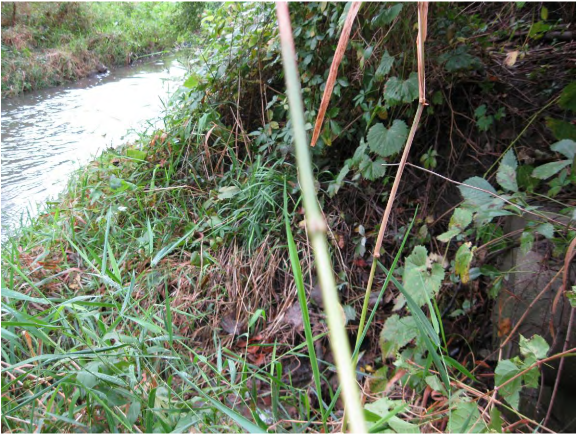
OC-16 Photo 2: Outfall pipe along Otter Creek.
