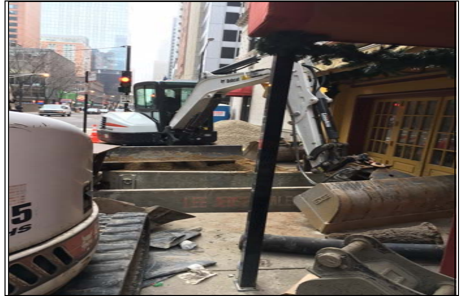
Photo 2: View facing south along west side of N Saint Clair Street of excavation
