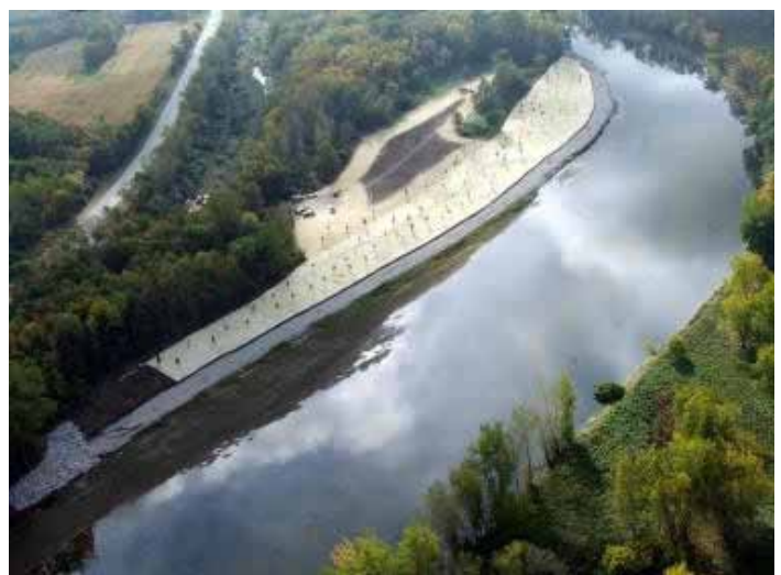
Riverbank removal in 2007; more than 300 mature trees were removed, today the area is a meadow with native vegetation and younger trees.
