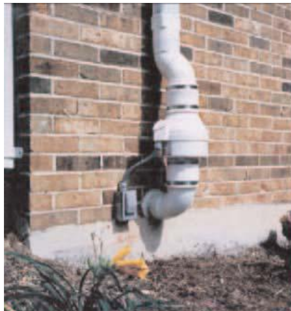
An example of a system that draws radon and other vapors out of the soil and vents them outside. It's known as a “sub-slab mitigation system.”
