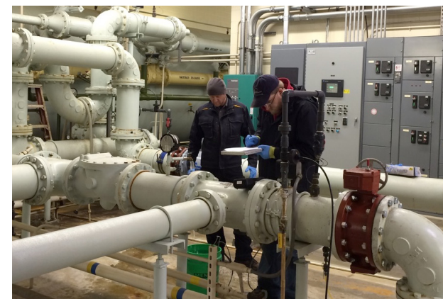
Drinking water treatment plant.
