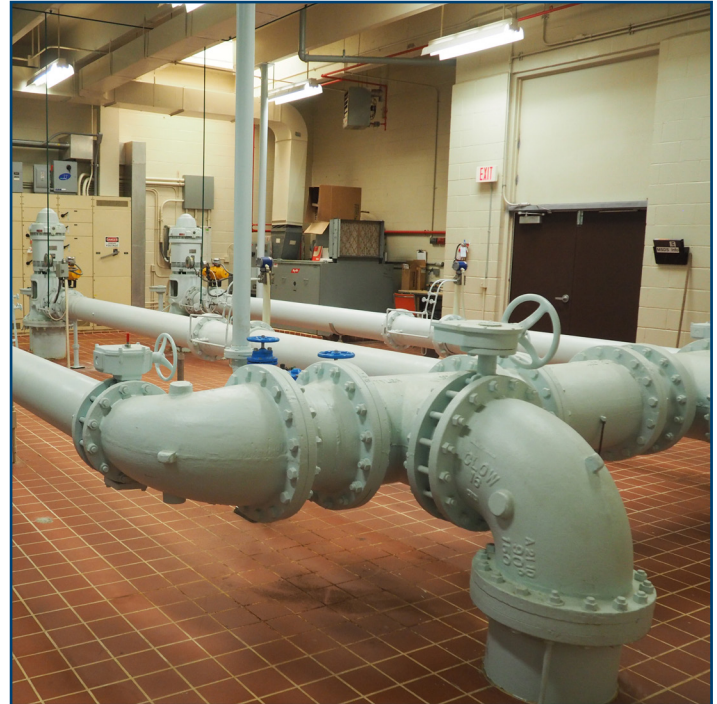
Drinking water treatment plant.
