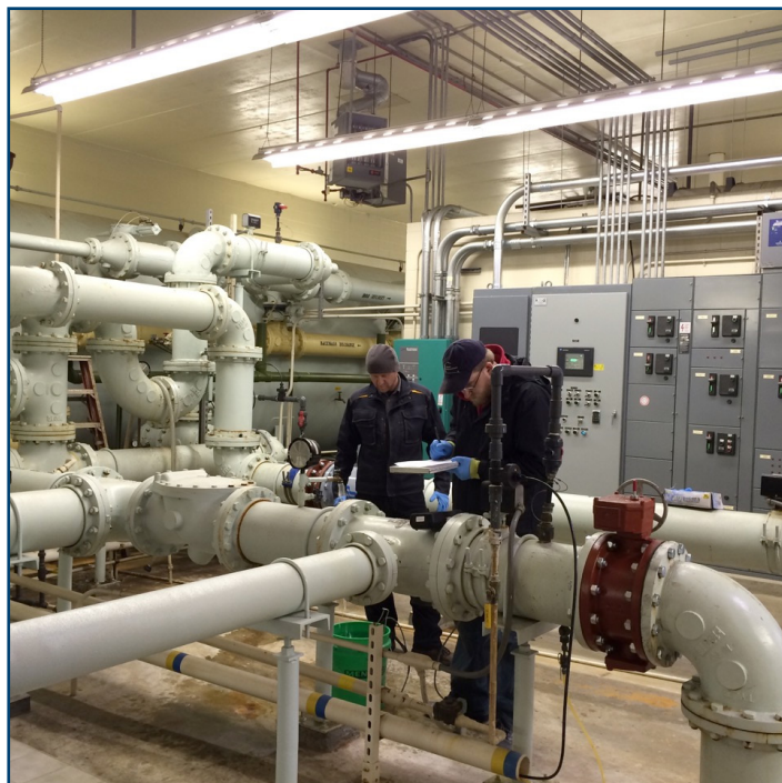
Drinking water treatment plant.
