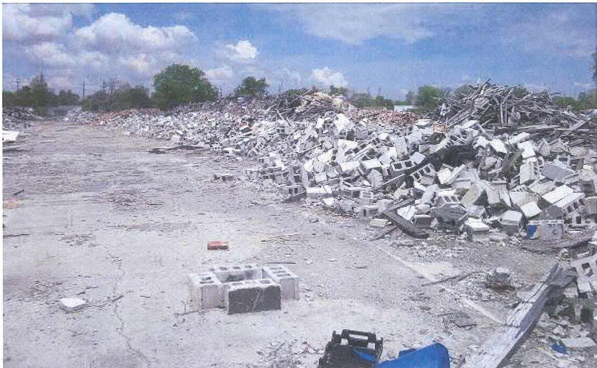
View of debris piles on-Site
