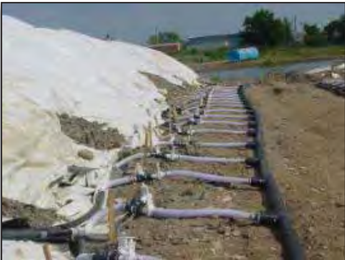
View of the vapor extraction system installed in Area 5.
