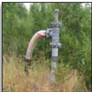
Landfill gas abatement system installed at the site.
