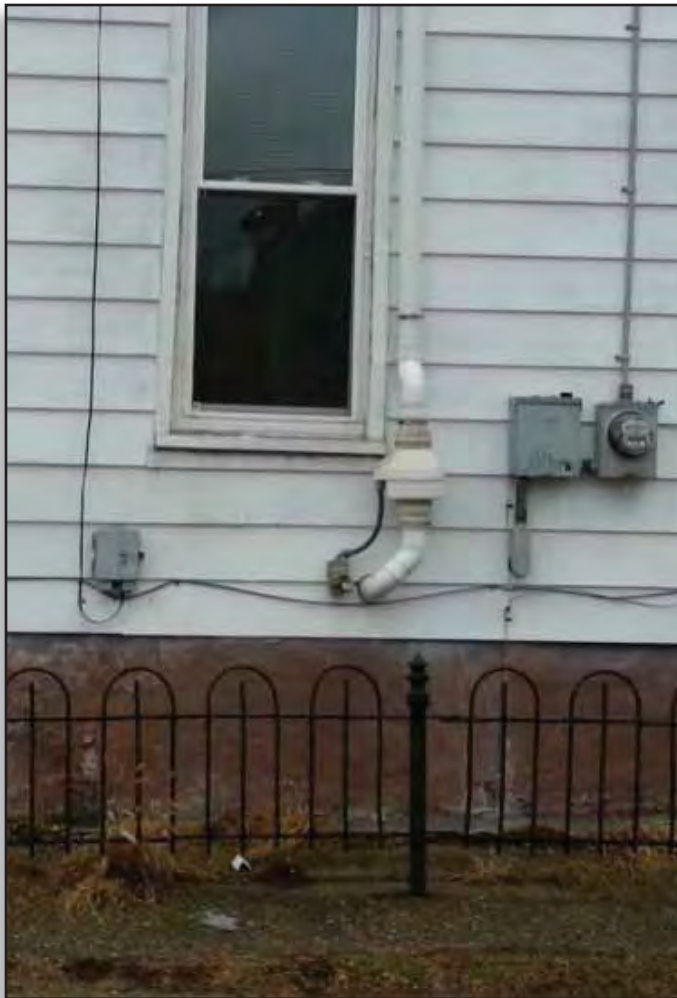
A vapor mitigation system installed in a residence.
