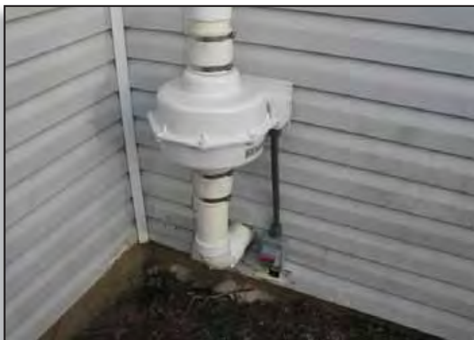
A vapor abatement system fan installed outside the house to remove contaminated vapor.
