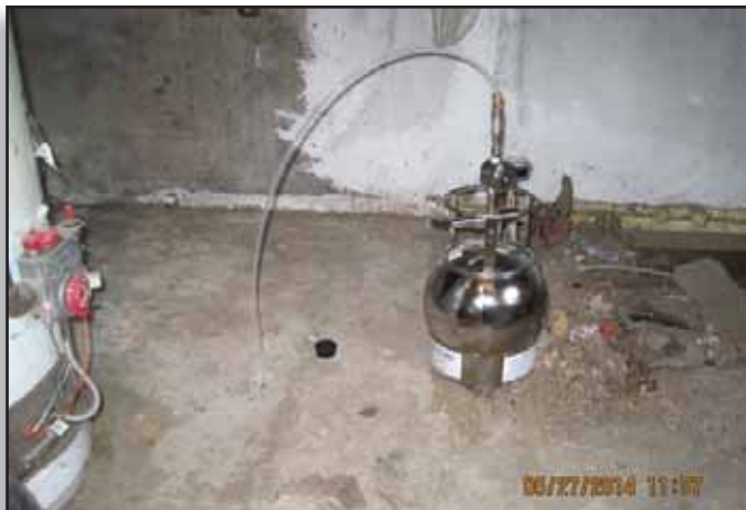
SUMMA canister used to collect a sub-slab sample.
