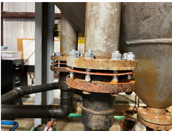
Photograph 15: Carbon vessel connection corrosion
