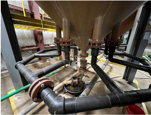
Photograph 17: Carbon vessel connection leaks w/containment and conveyance
