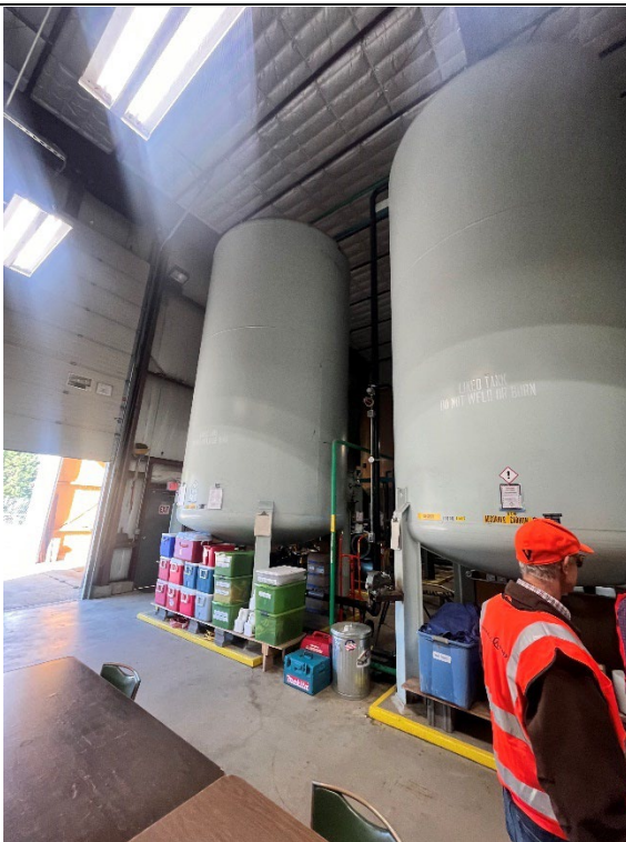
Photograph 19: Treatment plant interior and tanks
