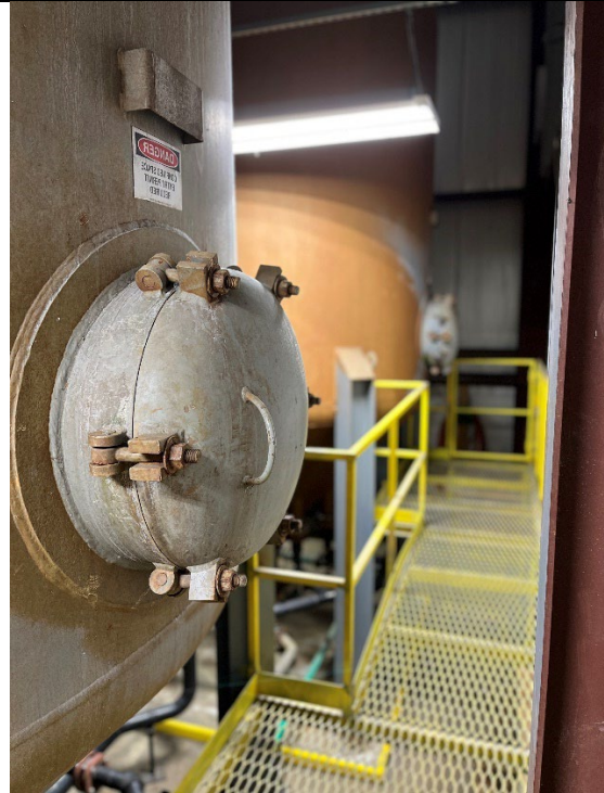
Photograph 14: Carbon vessel access point
