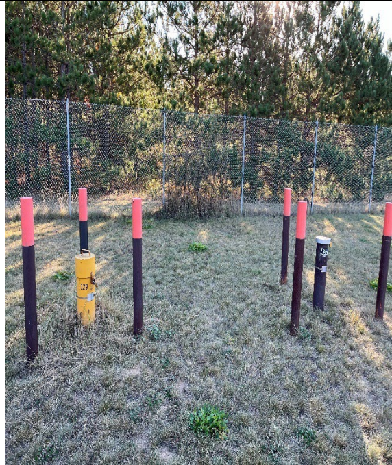
Photograph 2: OU2 Monitoring Wells 329 and 129 (looking east)
