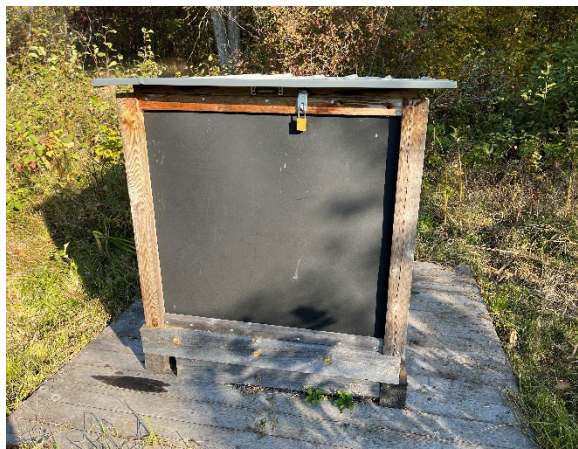
Photograph 6: OU3 Extraction Well house
