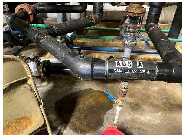
Photograph 16: Treatment plant sample valve
