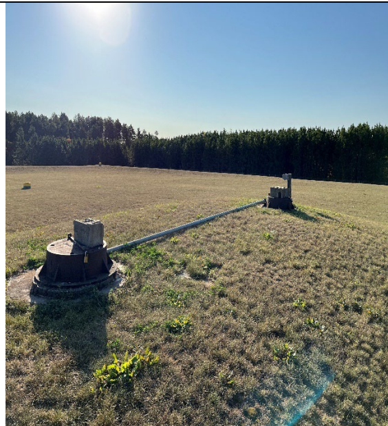
Photograph 4: OU2 Leachate Collection Manhole and Leak Detection Manhole
