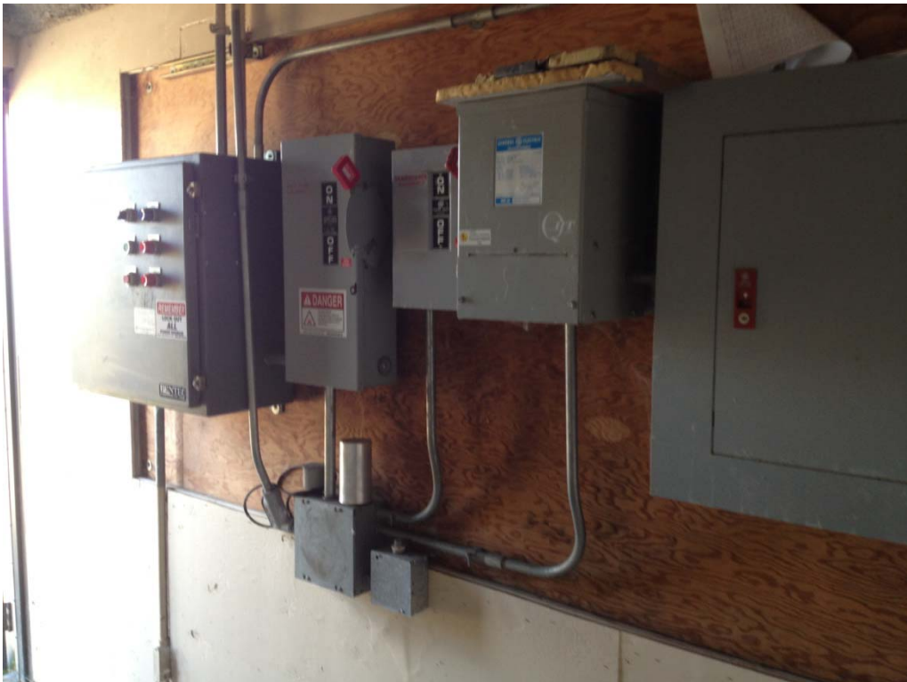
Relief Well B-6, Control Panel
