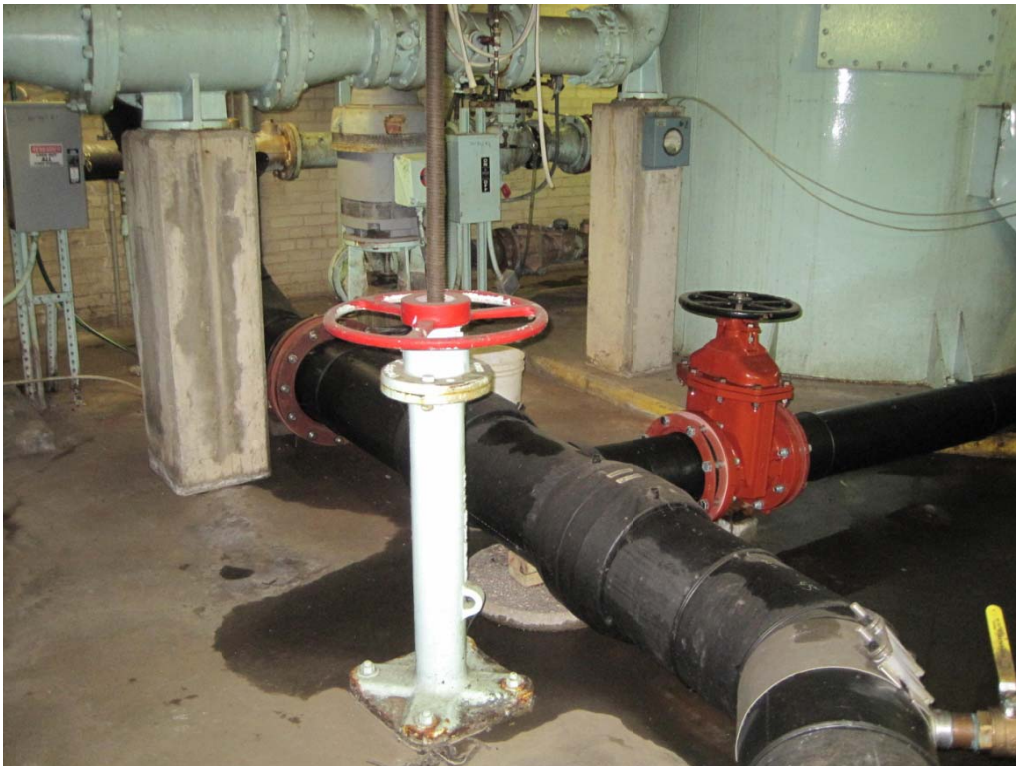
TCAAP Groundwater Recovery System inlet Piping(OU2)
