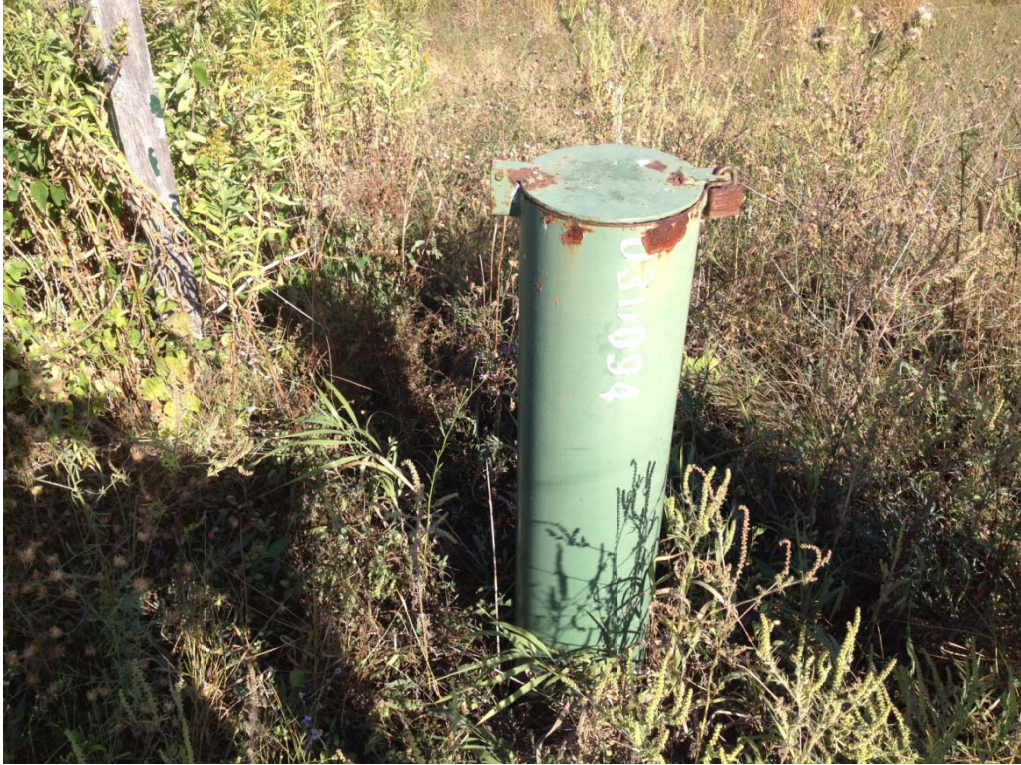
Site G, Monitoring Well 03U094 (uncertain of well ID – ID is worn). Well may need to be abandoned.
