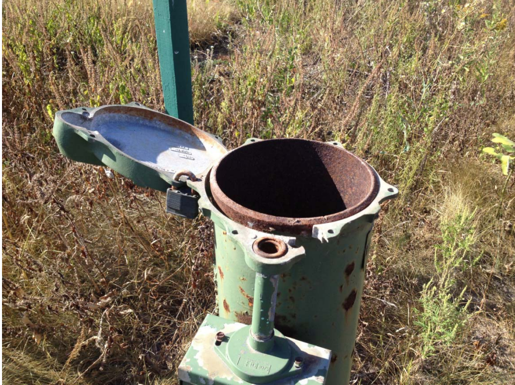
Site A, Monitoring Well 01U356. Cover broken and well not secure.
