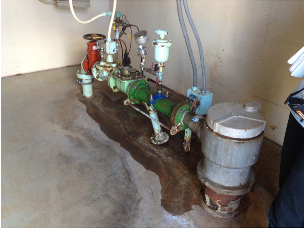
Relief Well B-6, Well and Pump
