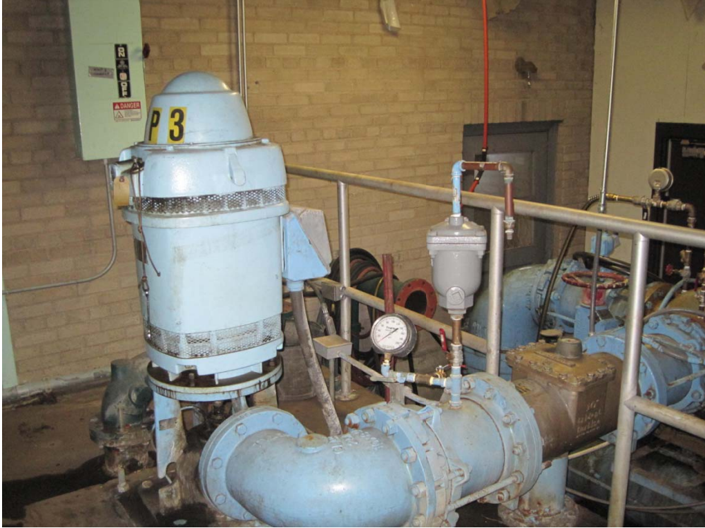
TCAAP Groundwater Recovery System Discharge side
