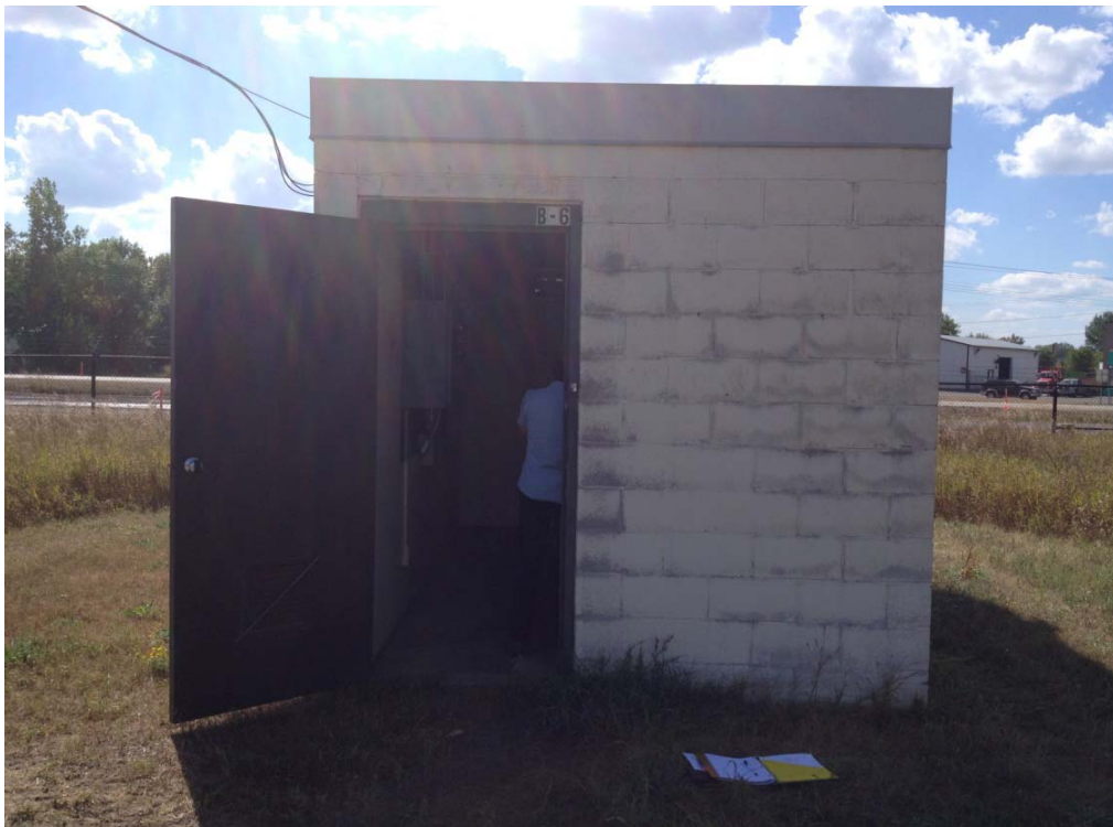
Relief Well B-6, Pump House
