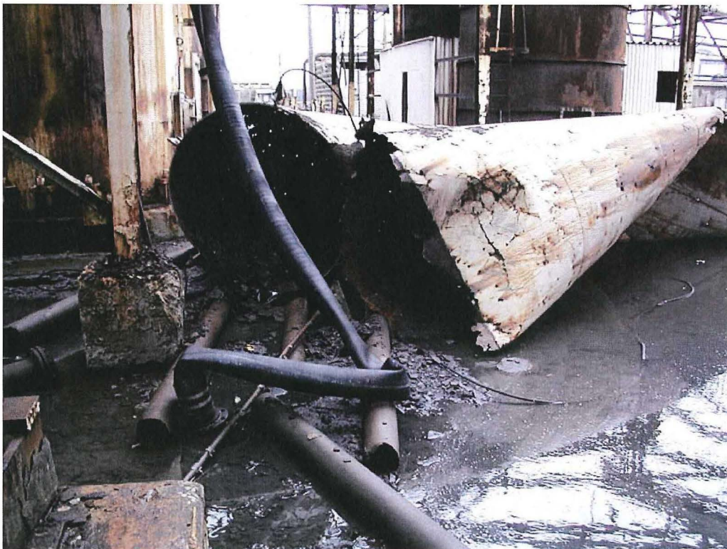
Flooding, scrap, and sludges at site, 2010.
