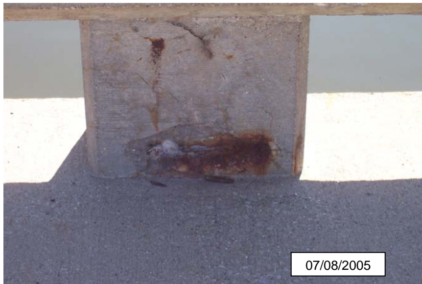
Photograph 22 - Representative parapet base spalling
