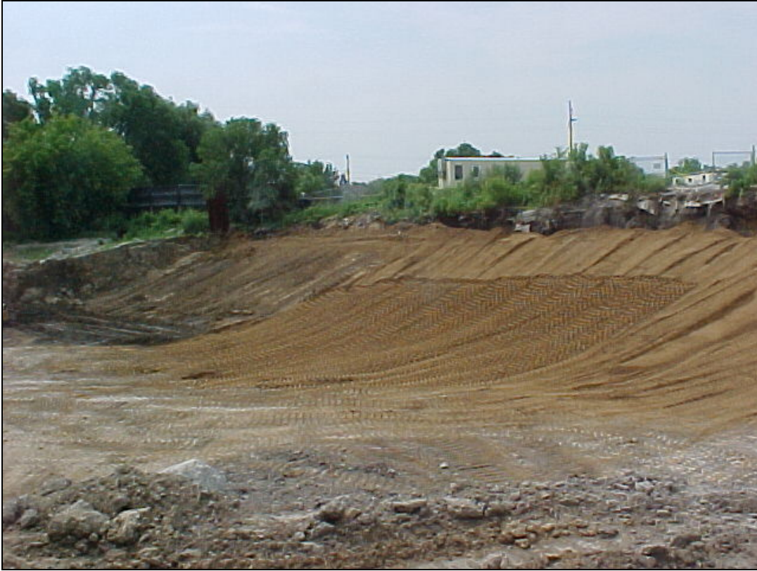
PHOTO 9—The equalization basin shoreline after backfill and placement of sand in July 2006.
