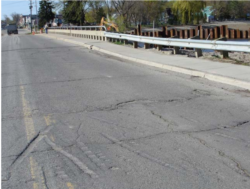
Photograph 7 - North approach pavement damage
