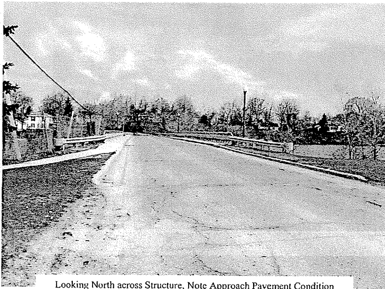
Looking North across Structure, Note Approach Pavement Condition
