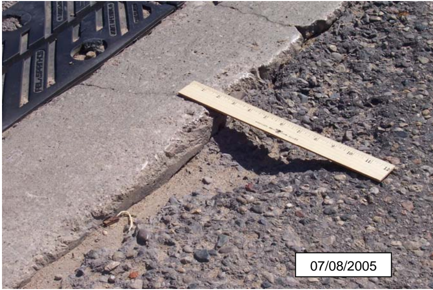
Photograph 23 - Asphalt condition at Pier 2 Expansion Joint
