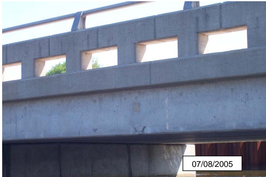
Photograph 28 - Damage at Span 2, west fascia beam
