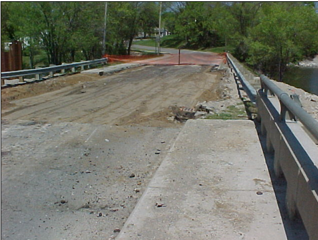
PHOTO 6—Damaged portion of Mill Street and adjoining sidewalk removed in May 2006.
