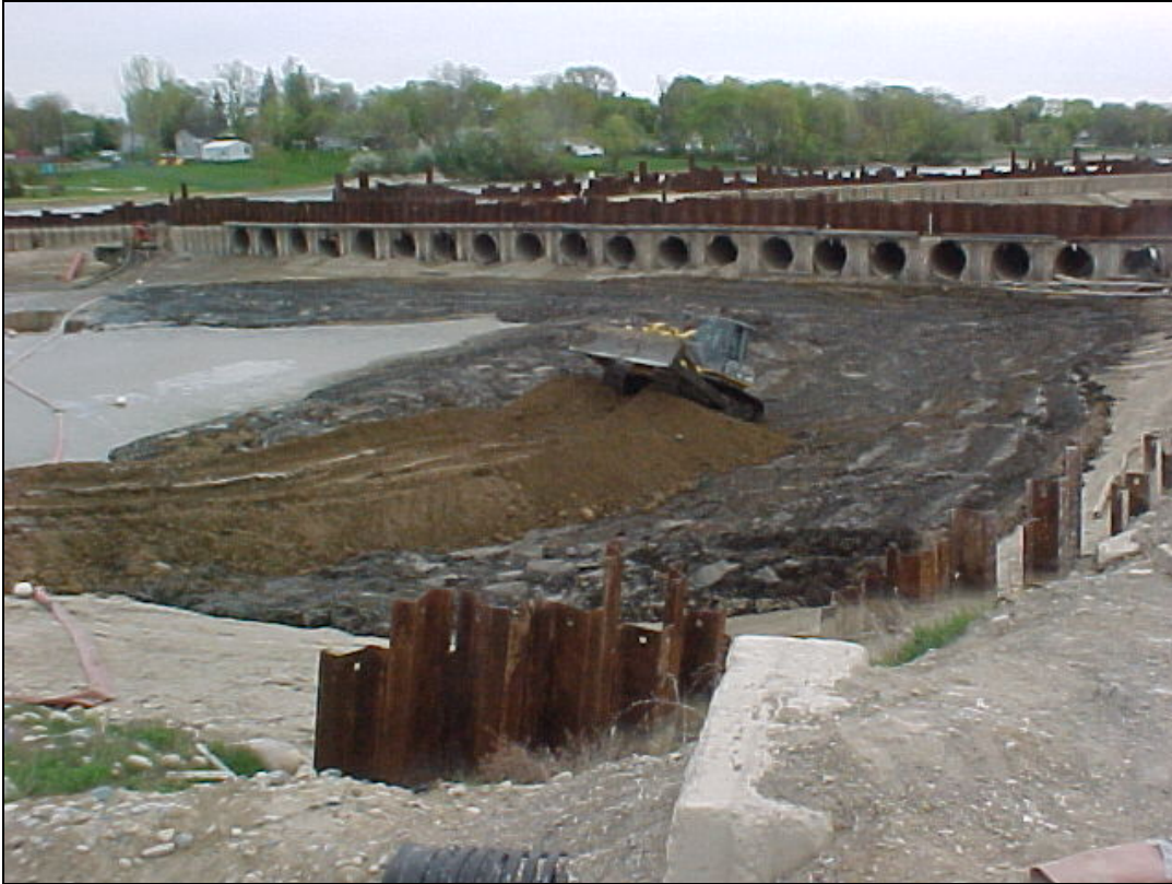
PHOTO 3—Creation of the berm/haul road around the perimeter of the equalization basin in April 2006.
