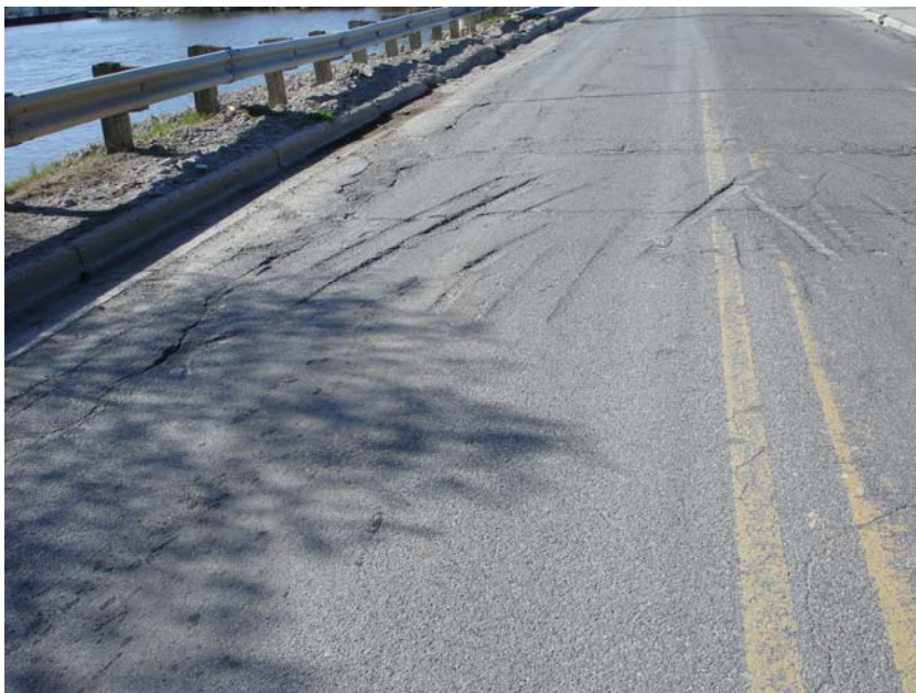
Photograph 6 - North approach pavement damage
