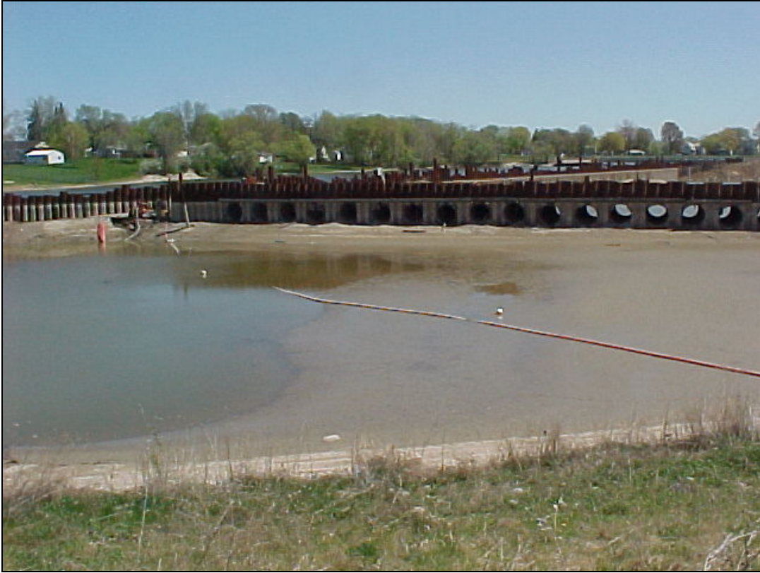
PHOTO 1—The location of the former Hot Spot Cell after dewatering in April 2006.
