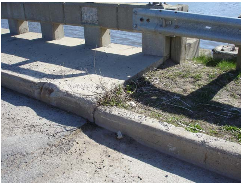
Photograph 8 - Southeast approach shoulder deterioration
