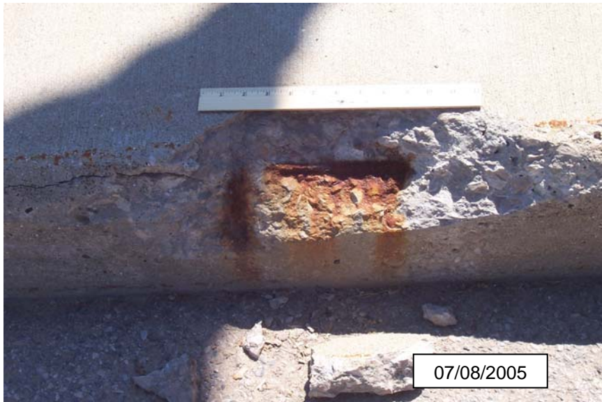
Photograph 26 - Curb spall at southeast corner
