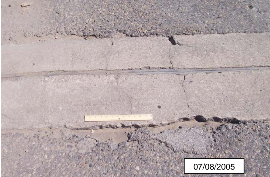
Photograph 24 - Asphalt condition at Pier 1 Expansion Joint
