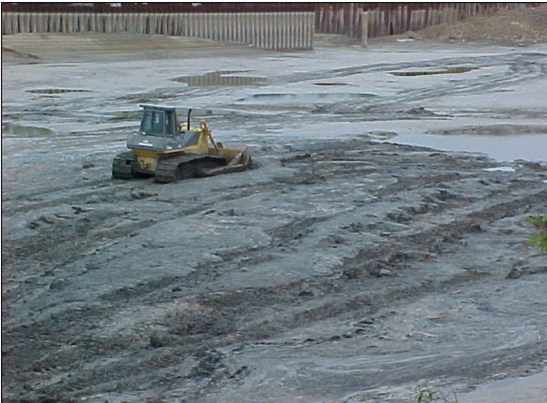
PHOTO 4—Bulldozer traversing Cell 1, 2, 3 in May 2006; approximately 1 foot of sediment had accumulated during the 2 years that river flow had been restored to the southern half of the river.
