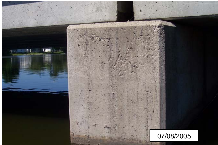
Photograph 27 - East face of Pier 2 showing scaling
