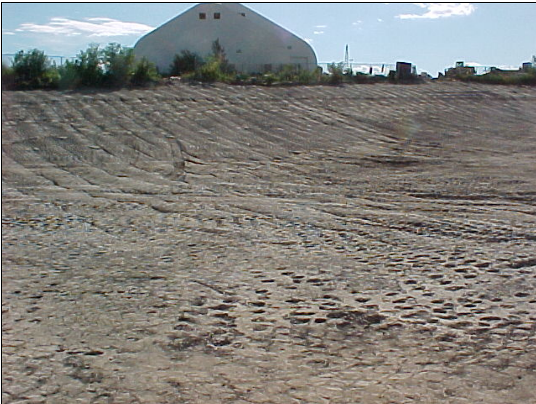
PHOTO 10—The equalization basin shoreline after placement and compaction of clay in July 2006.
