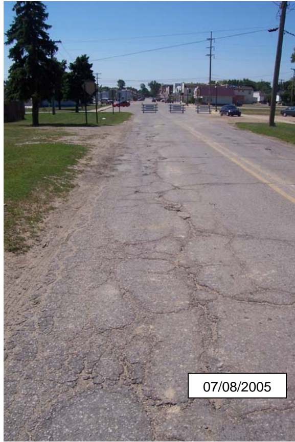
Photograph 21 - Southeast approach shoulder deterioration
