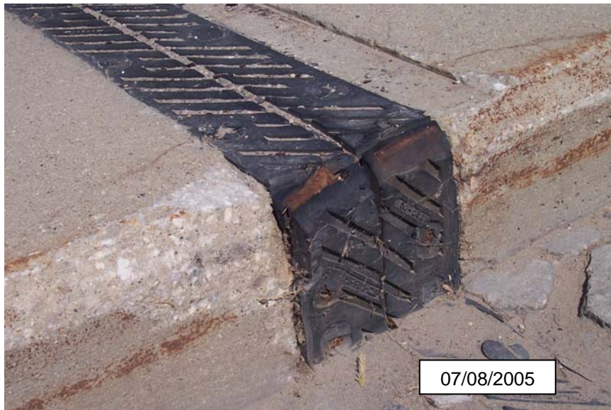
Photograph 25 - Pier 2 expansion joint damage
