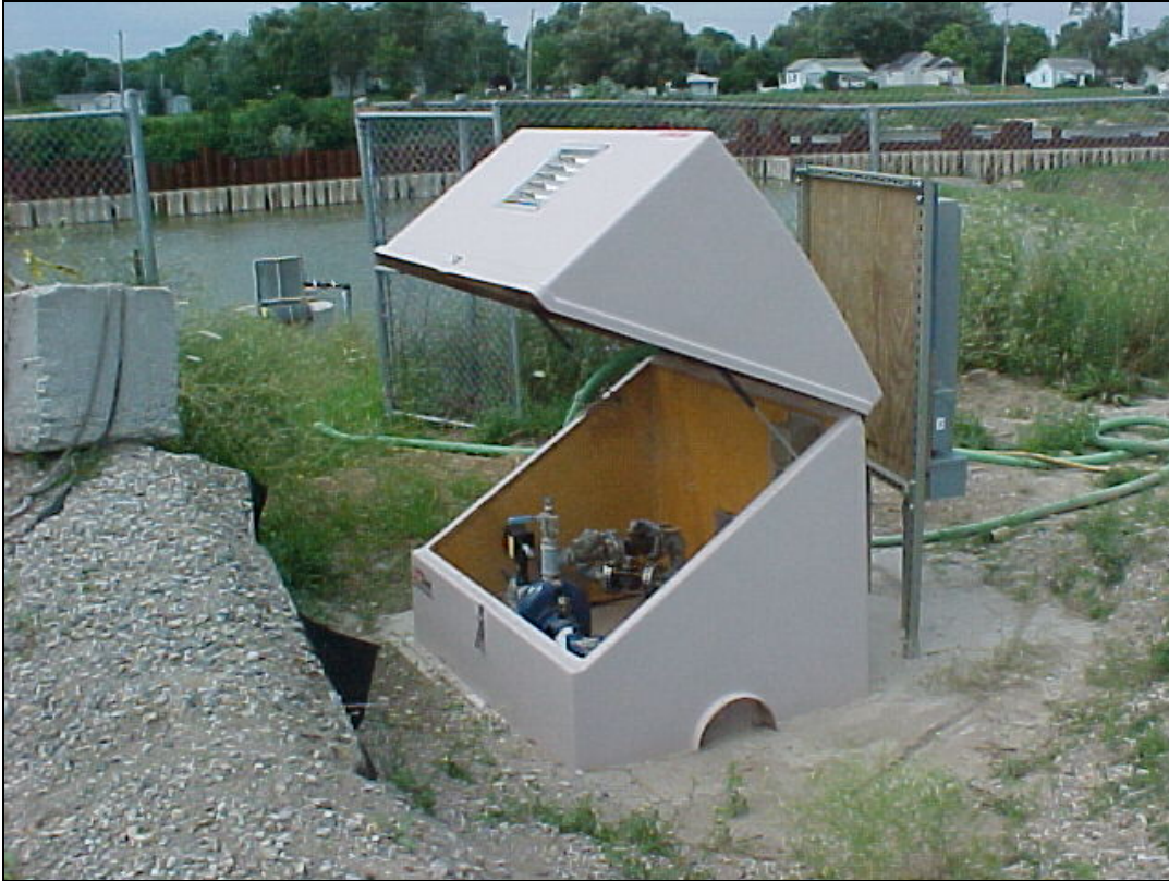
PHOTO 11—An open enclosure showing one of the pumps during modification of the GCS in July 2006.
