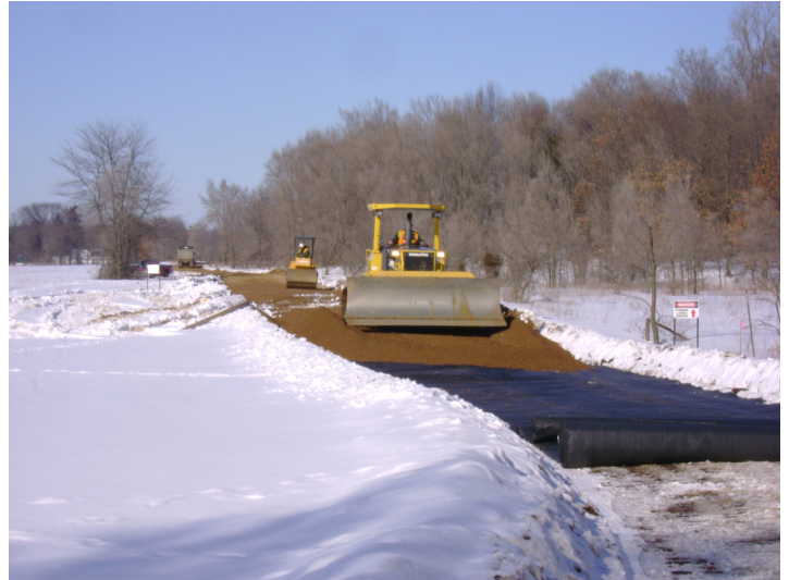
Grading the access road between Miller Road and the Kalamazoo River using a D61 dozer.
