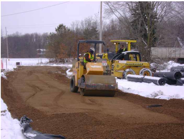
Compacting aggregate on the access road between Miller Road and the Kalamazoo River using a smooth drum roller.
