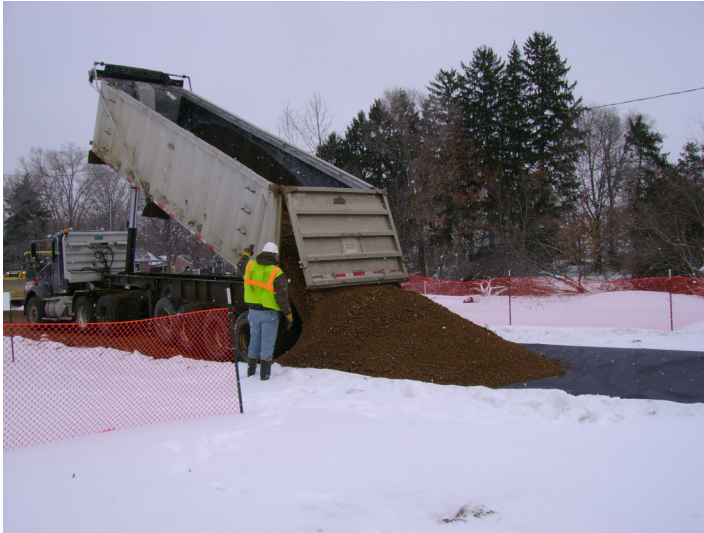
Placing aggregate for the construction of the access road between Miller Road and the Kalamazoo River.
