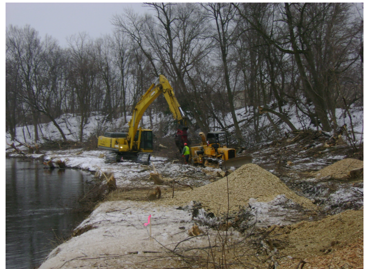
Clearing and chipping activities in Removal Area 12B using a PC 300 excavator and a Vermeer chipper.
