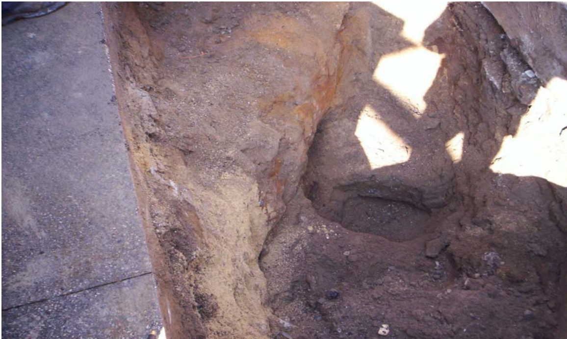
Photo 5: Taken south to north. Shows 24-inch gas main crossing test pit #1 location.
