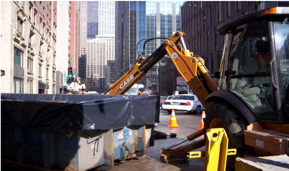
Photo 4: Taken south to north. Shows excavation of test pit #1, with backhoe loading clean soil into roll-off box.
