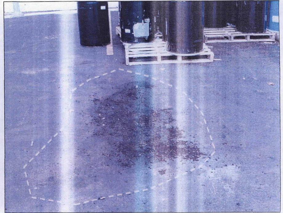
Staining and Deteriorated Asphalt Near Empty Drum Storage Area
