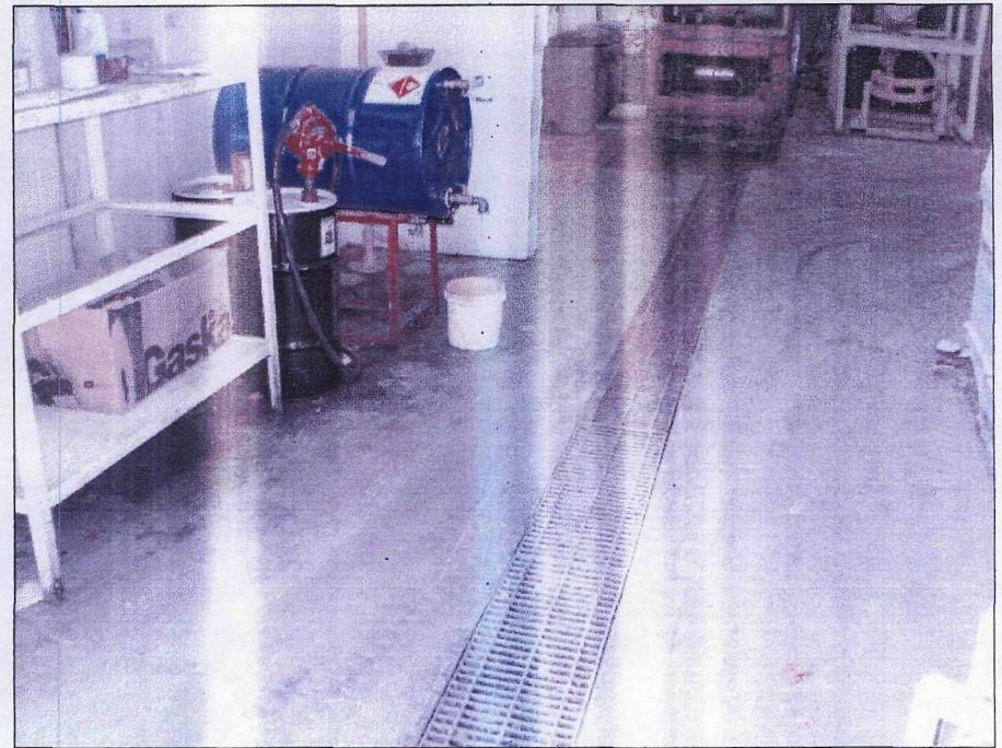
Trench Drain System Throughout Chemical Storage/Mixing Area
