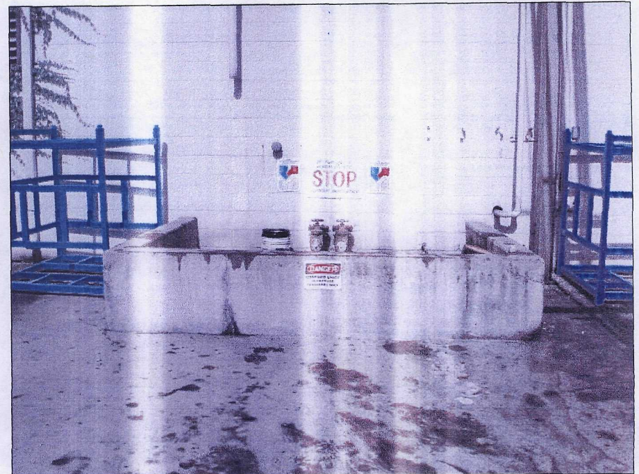
Remote Fill Manifold for Interior ASTs Located at Southwestern Exterior of Building (Note staining on concrete pavement and containment structure)
