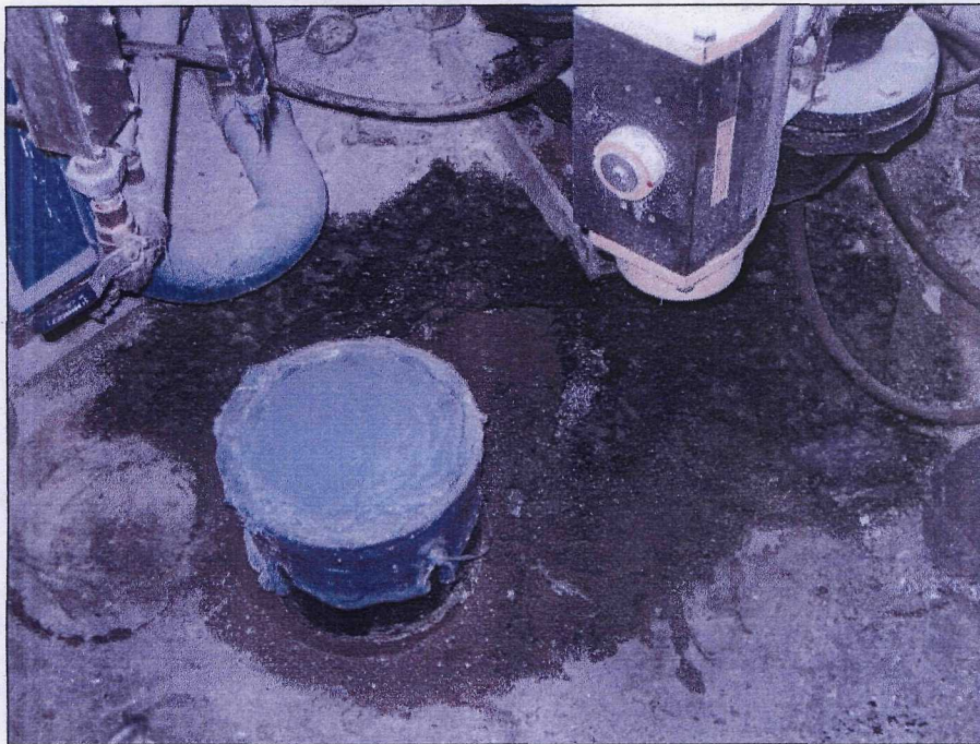
Typical Staining on Concrete Floor in Interior Chemical Storage Area
