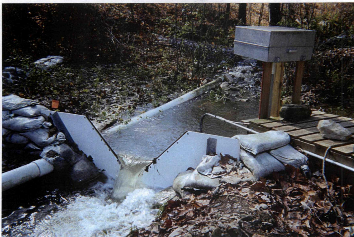
Photograph No. 13 Orientation: Southwest Description: Overflow at V-notch weir in Overflow Spring 34
